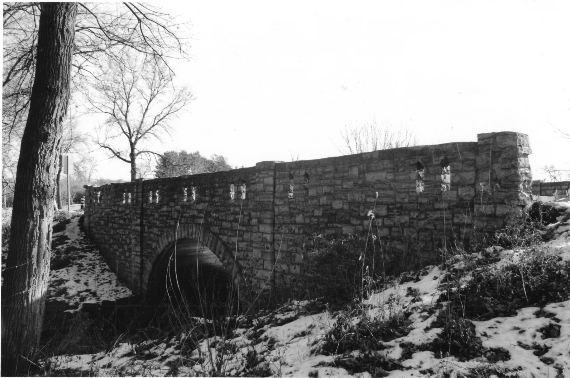
Bridge no. 8096 Mn Hwy. 19 over Spring Creek, Northfield Rice Co., MN 012839-21A/22
