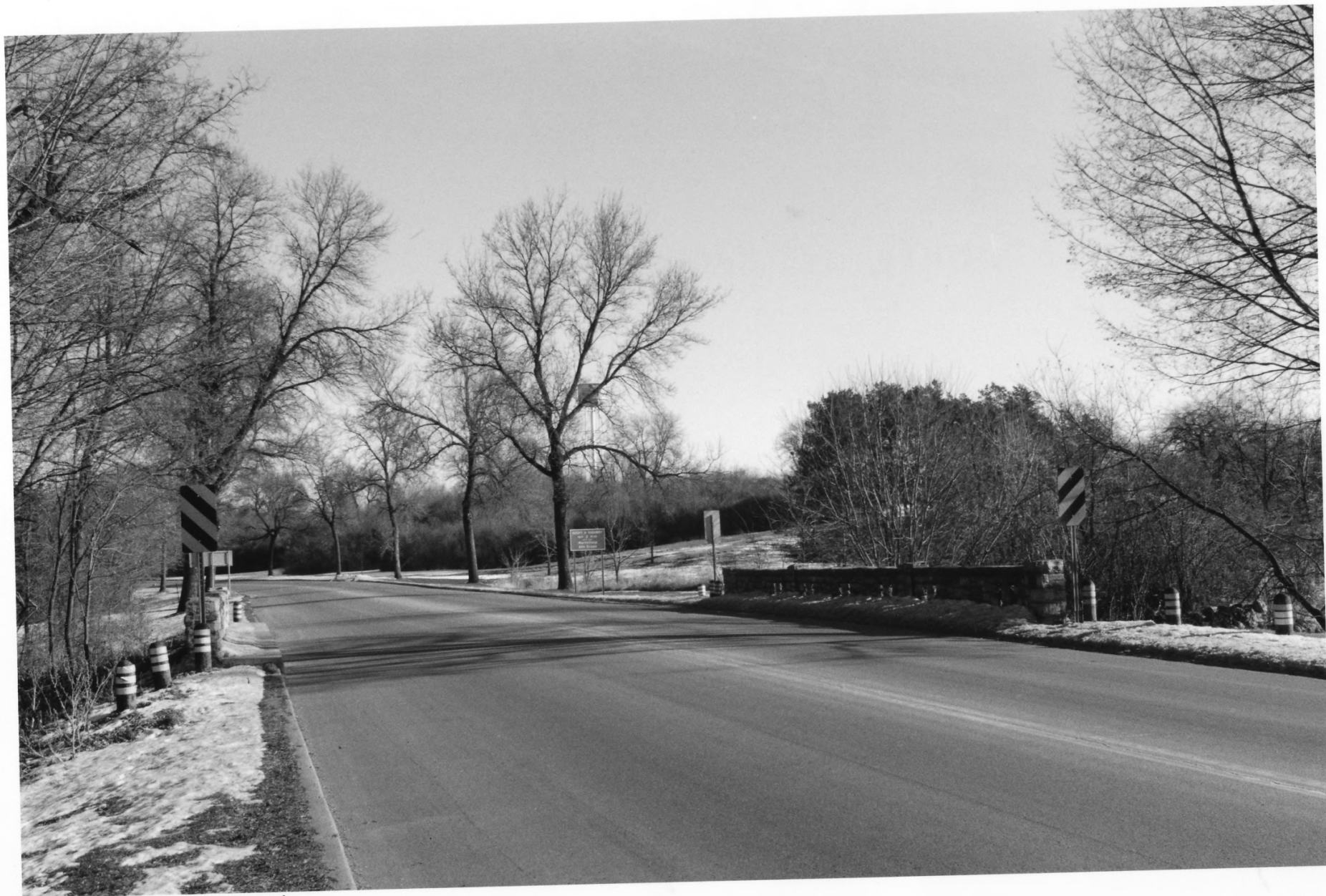
Bridge no. 8096 Mn Hwt. 19 over Spring Creek, Northfield Rice Co., Mn 012839-23A/24
