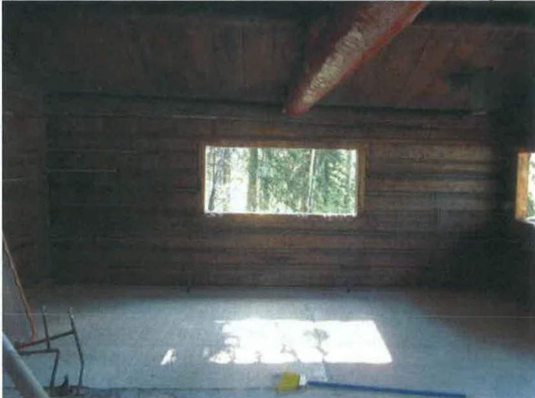
Figure 100- East Elevation. Historic logs and roof are in excellent condition (NPS Photo, August 2013).
