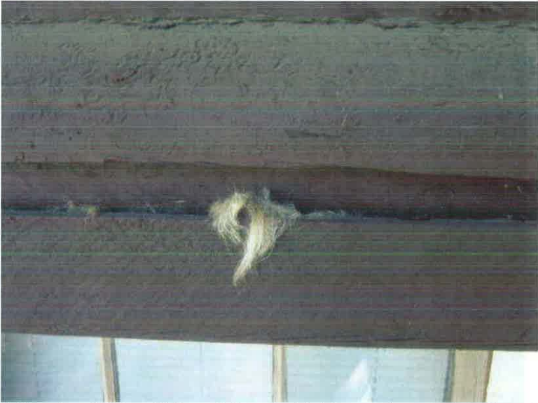
Figure 49- Chinking above Window #4, from window schedule (Figure 5 Figure 6). (NPS Photo, August 2012).
