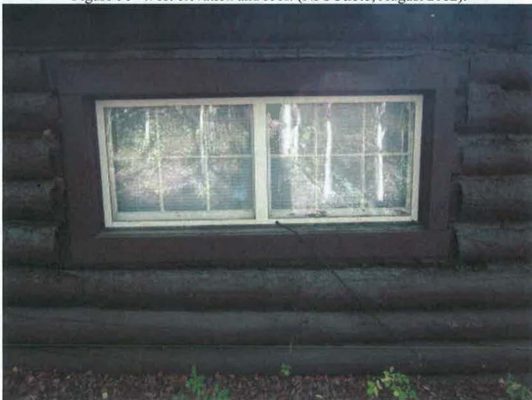
Figure 59- Window #8 (left) and Window #9 (right), from window schedule (Figure 5 Figure 6). (NPS Photo, August 2012).
