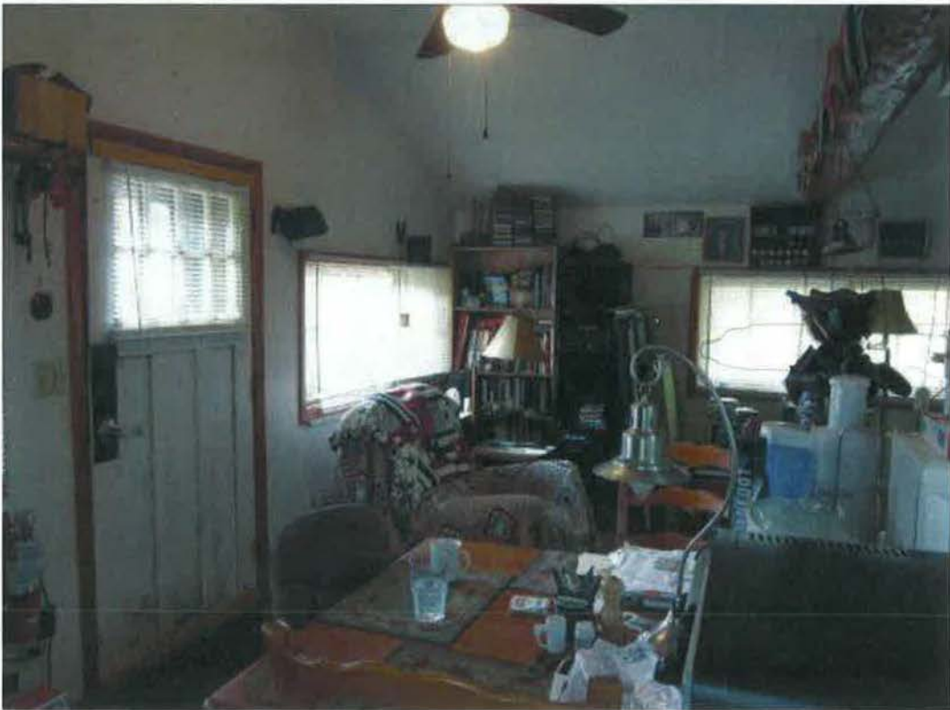
Figure 87- Living Area, note mildew on door. (NPS Photo, August 2012).
