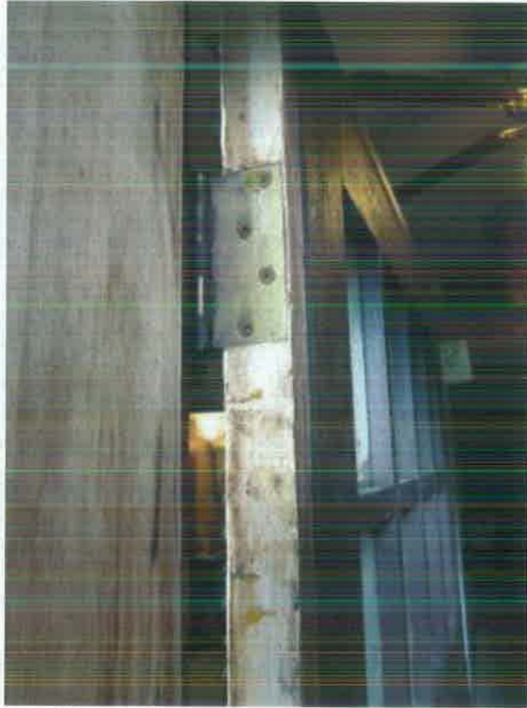
Figure 80- Hinge edge of door – evidence of previous hinge below existing hinge. (NPS Photo, August 2012)
