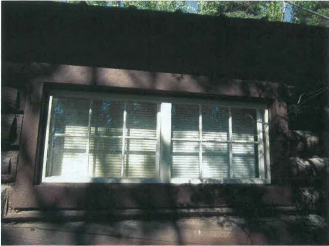
Figure 70- Window #5 (left) and Window #6 (right), E elevation, from window schedule (Figure 5 Figure 6). (NPS Photo, August 2012).
