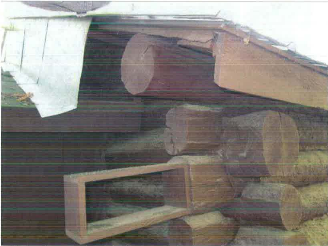
Figure 64- NW elevation; note 1x box (perhaps was used as an antenna support bracket). Note also "vent" above and behind bracket. (NPS Photo, August 2012).
