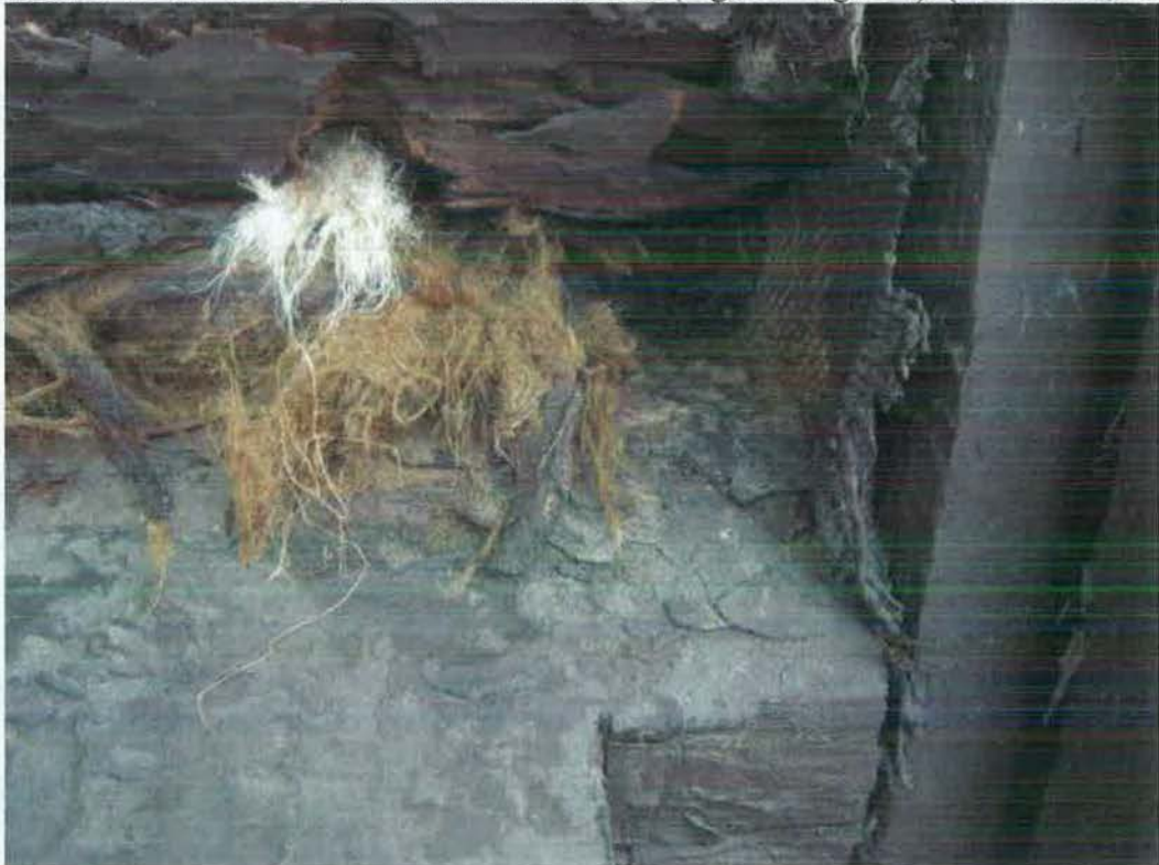
Figure 61- Chinking next to Window #8, from window schedule (Figure 5 Figure 6). (NPS Photo, August 2012).
