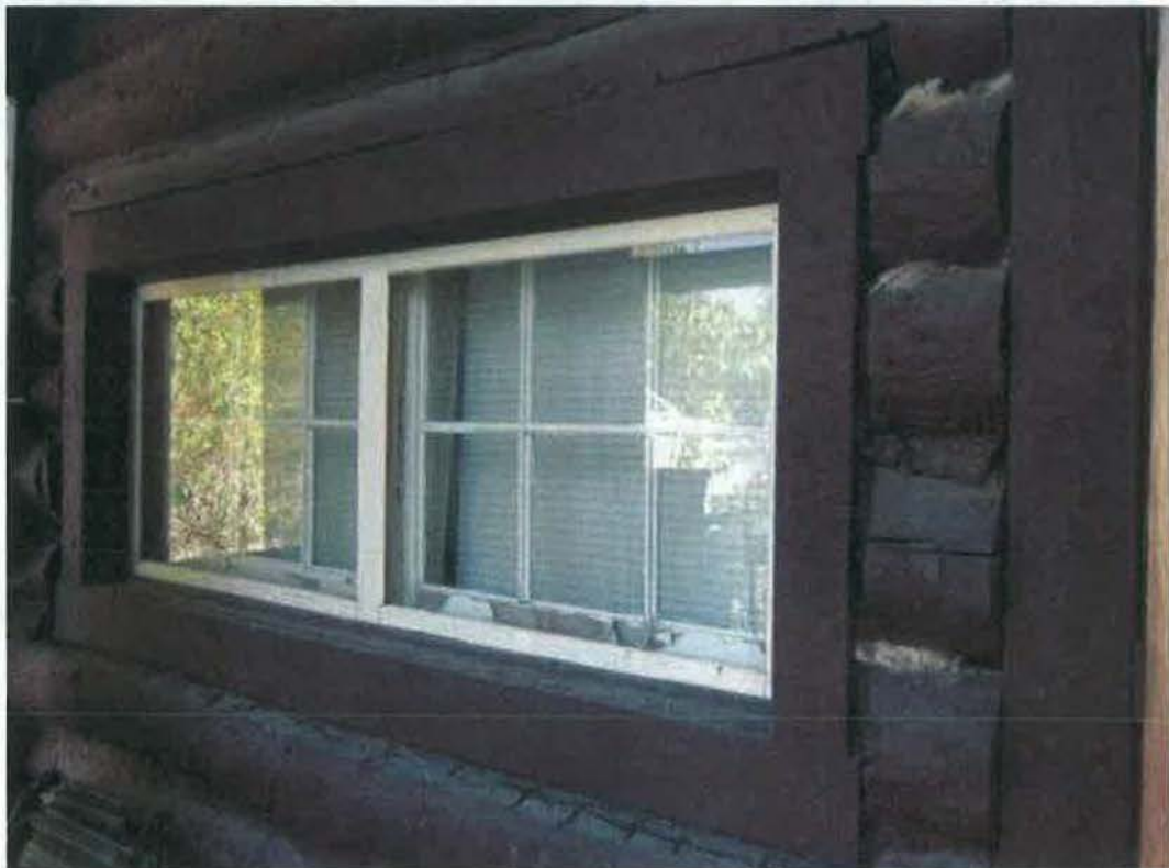
Figure 43- Window #1 (left) and Window #2 (right), from window schedule (Figure 5 Figure 6). (NPS Photo, August 2012).
