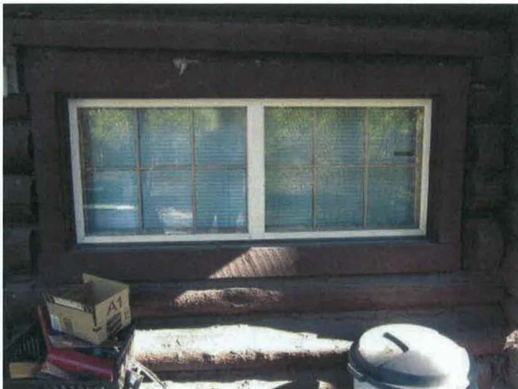
Figure 46- Window #3 (left) and Window #4 (right), from window schedule (Figure 5 Figure 6). (NPS Photo, August 2012).
