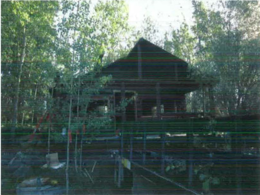
Figure 102- Removal of porch in progress. After relocation the porch will be reassembled (NPS Photo, August 2013).
