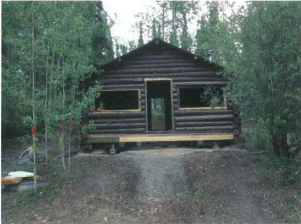
Figure 103- P-22 after removal of porch, 1979 addition, and modern interior elements. The building has been placed on jacks in preparation for moving it (NPS Photo, August 2013).
