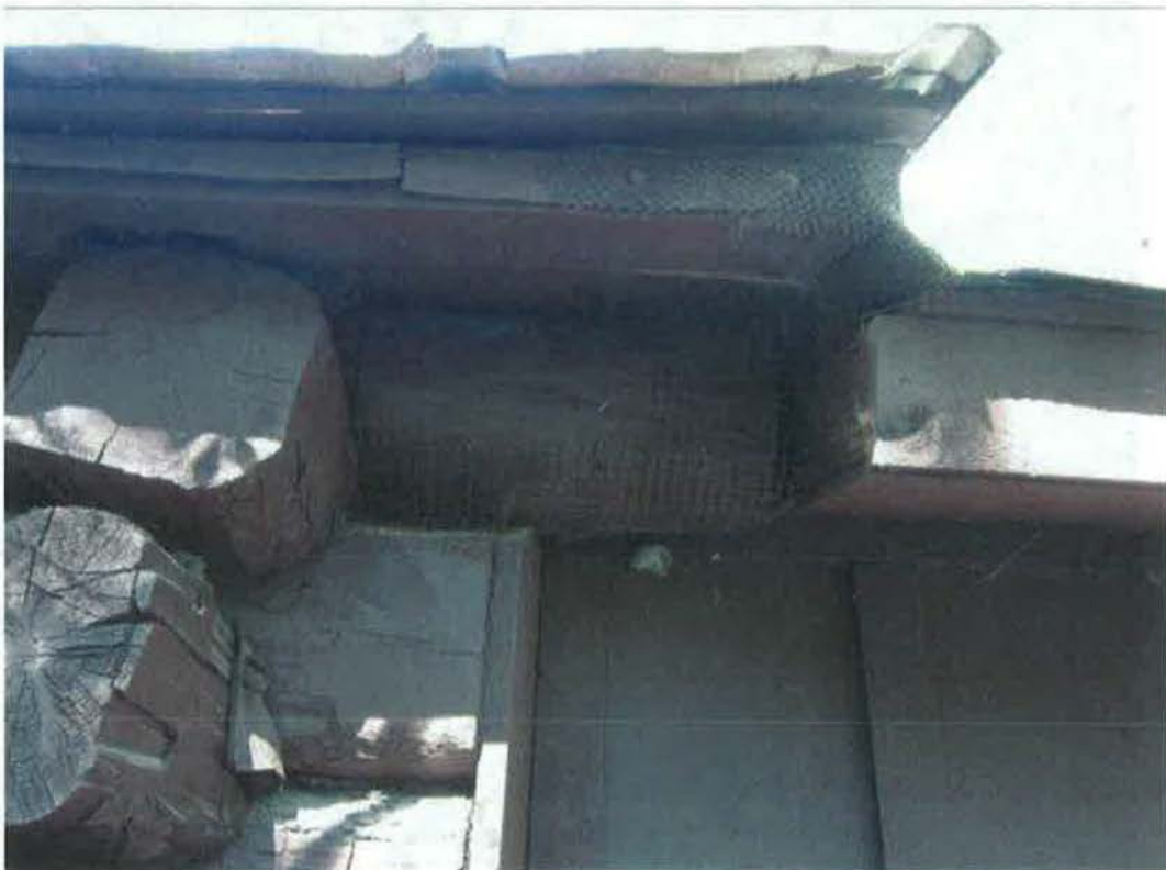
Figure 67- Connection detail at NE corner of original building and SE corner of addition. (NPS Photo, August 2012).
