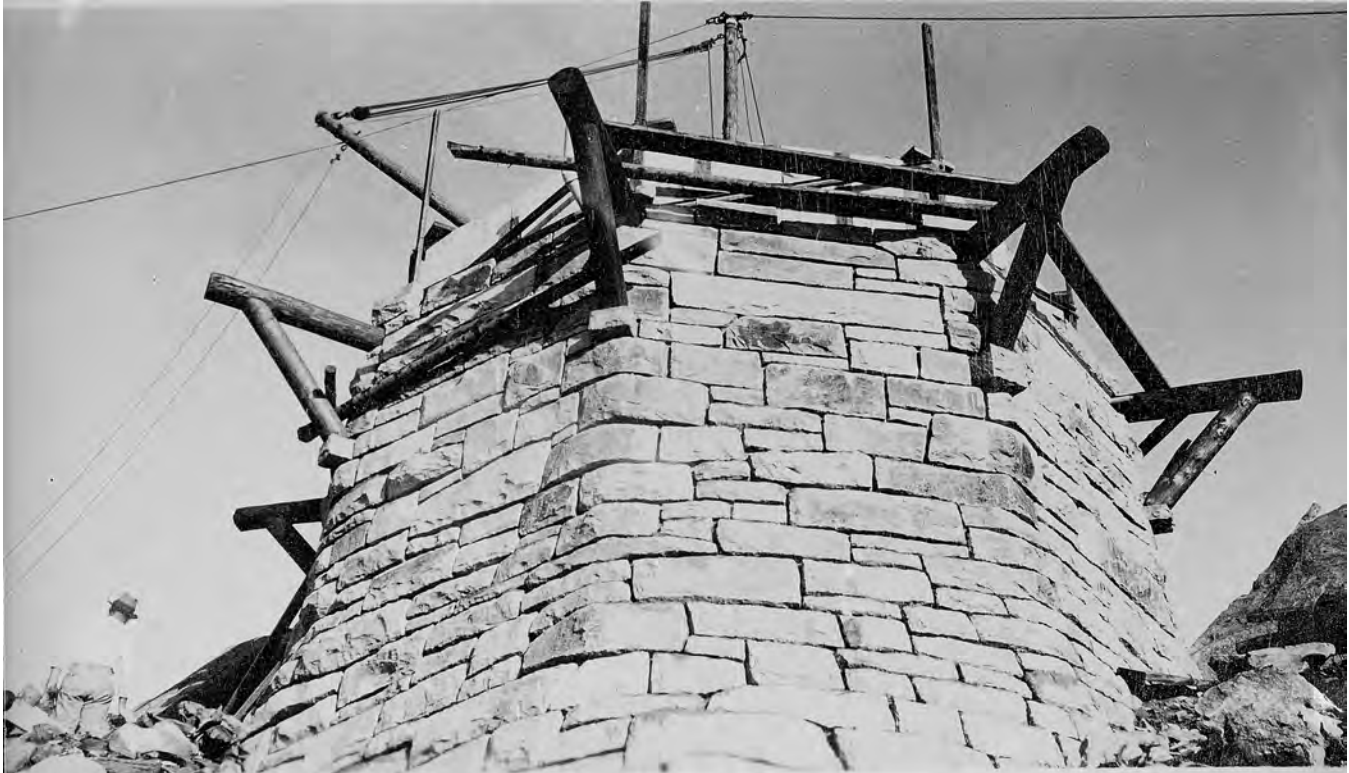
Figure 7. Photograph of Mount Cammerer Fire Lookout under construction, supports for catwalk in place, 1937 (source: GSMNP, Collection Preservation Center, Townsend Tennessee).
