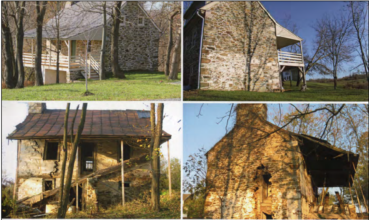
Figure 1. Amos Goodin House, “After and Before, Restoration; photos taken in 2015 (top) and 2010 (bottom). Photos by Matthew Parse.
