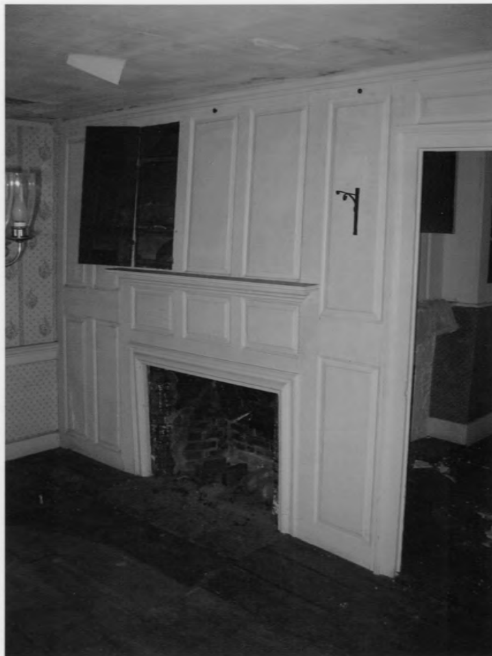
The Elam Ives House Hamden, New Haven County, Connecticut Photograph 5 The paneling in the northeast room April 2007 James Sexton
