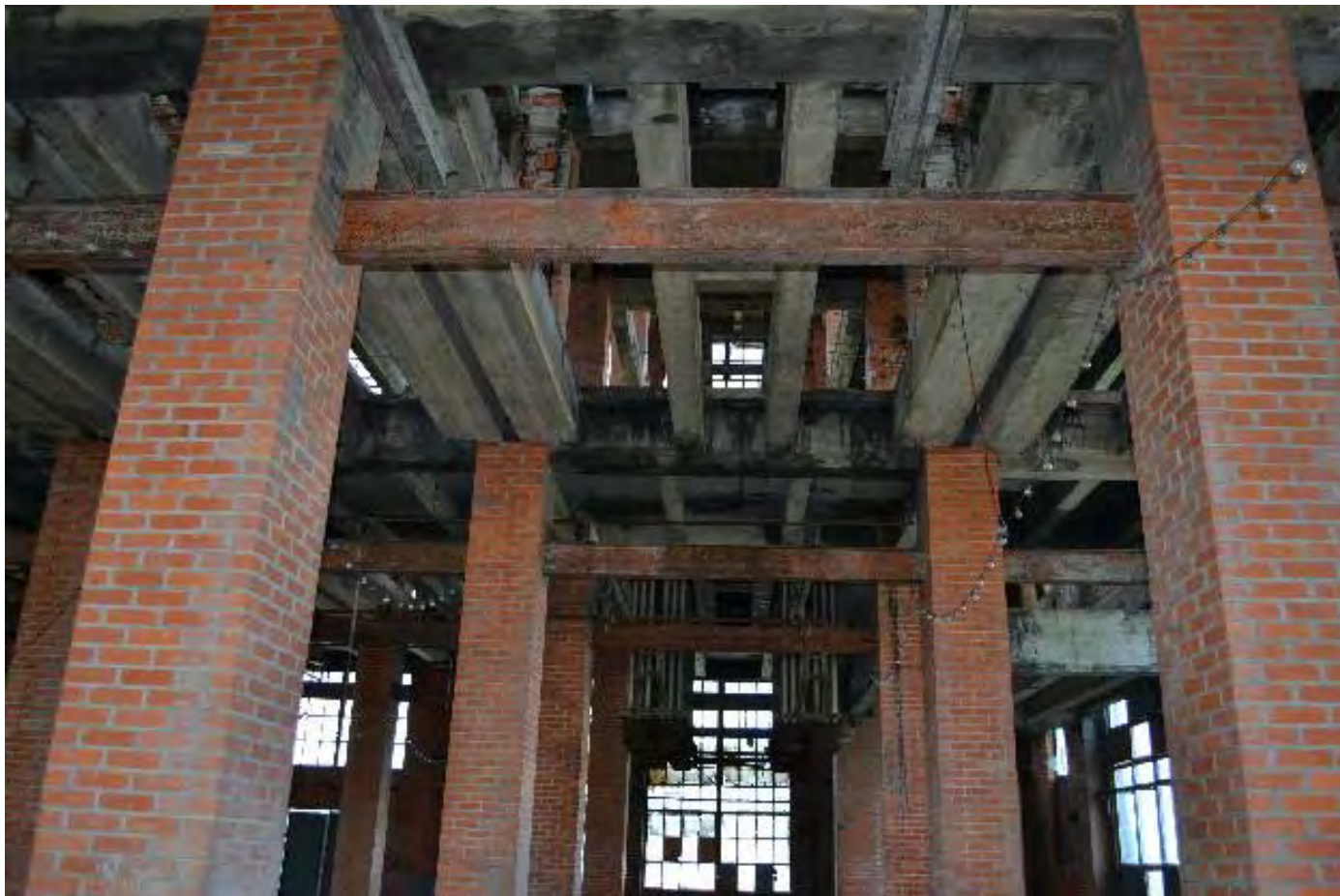
Photo 22 - Char House (Resource ID 1), interior, missing flooring visible, view north
