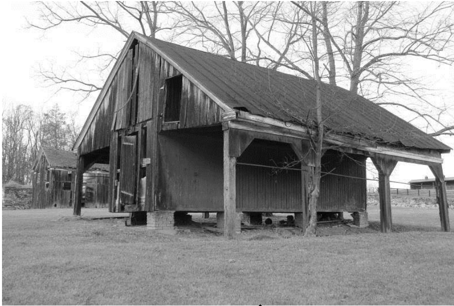
WV_Jefferson County_Wild Goose Farm_0035 Wagon shed/corn crib, south and east elevations, view NW
