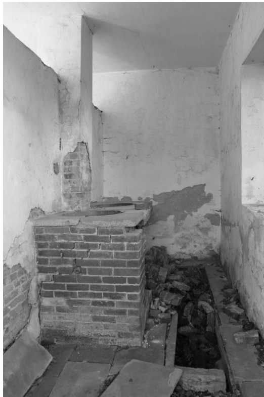
WV_Jefferson County_Wild Goose Farm_0019 Springhouse, interior view of wash room, view W
