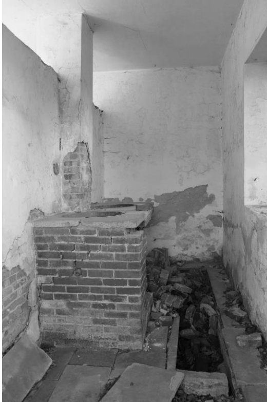
WV_Jefferson County_Wild Goose Farm_0019 Springhouse, interior view of wash room, view W
