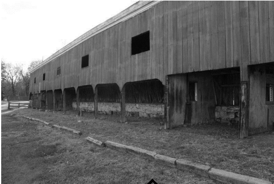
WV_Jefferson County_Wild Goose Farm_0033 Shed attached to barn, east elevation, view S
