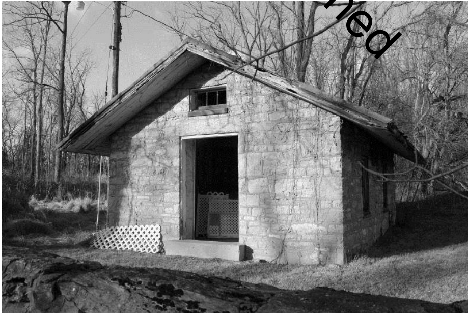
WV_Jefferson County_Wild Goose Farm_0027 Pump house, south and east elevations, view NW
