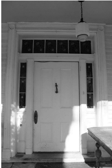
WV_Jefferson County_Wild Goose Farm_0006 Mansion exterior, south elevation, main entrance, view N
