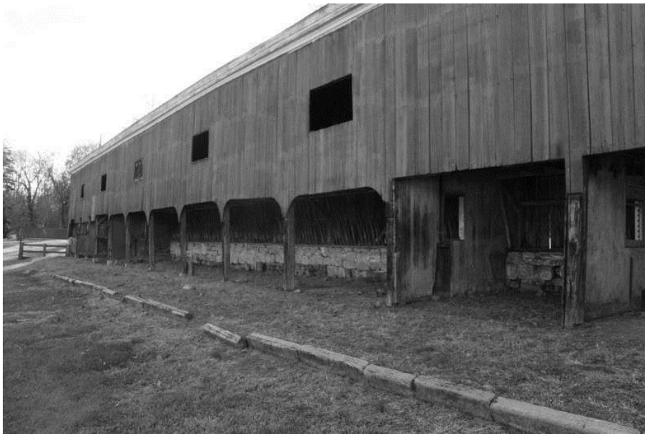
WV_Jefferson County_Wild Goose Farm_0033 Shed attached to barn, east elevation, view SW
