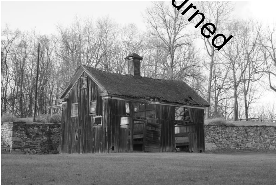
WV_Jefferson County_Wild Goose Farm_0036 Poultry house, south and east elevations, view NW
