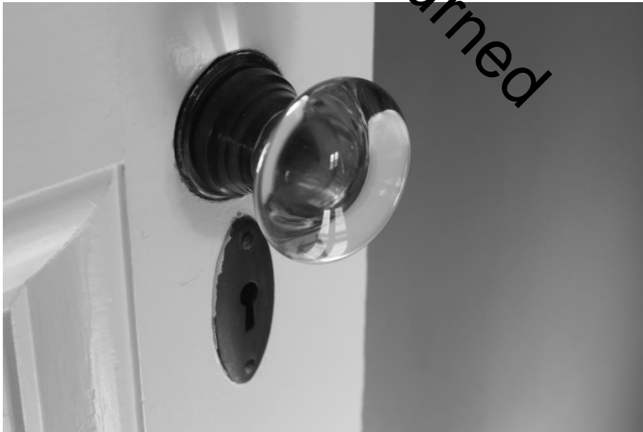
WV_Jefferson County_Wild Goose Farm_0011 Mansion interior, first floor, detail of interior door knob and lock
