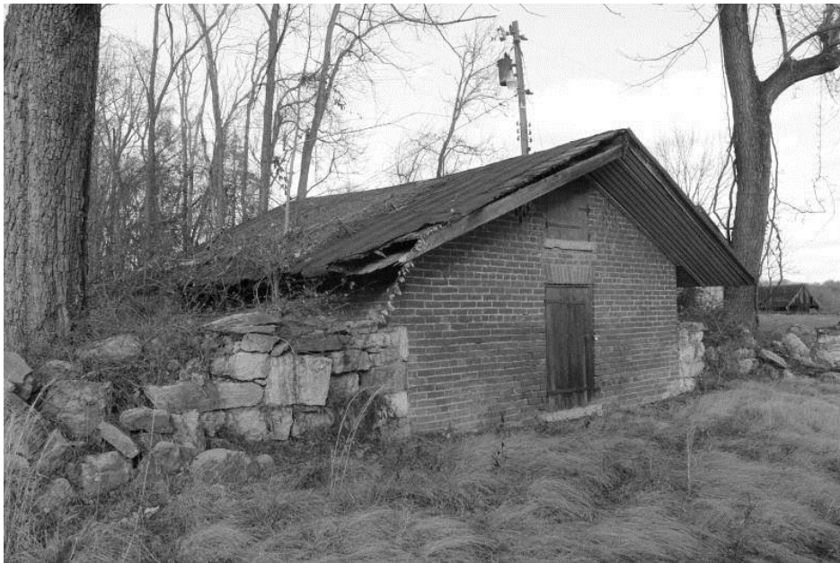
WV_Jefferson County_Wild Goose Farm_0026 Ice house, west and south elevations, view NE
