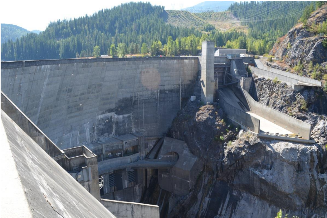
Photo 6 of 25: (WA_PendOreille_BoundaryDam_006) Boundary Dam, Left Spillway, Sluice Gates on downstream face, camera facing SW from dam crest at right abutment (A)
