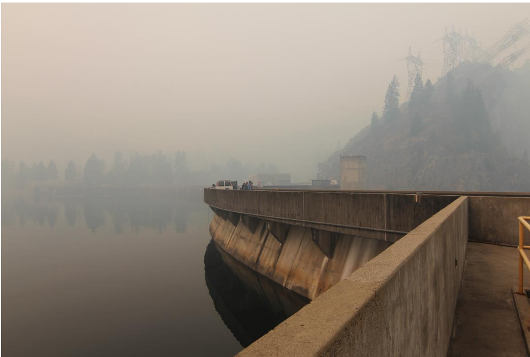
Photo 10 of 25: (WA_PendOreille_BoundaryDam__0010) Boundary Dam, Dam Crest, camera looking W, toward Forebay (K)
