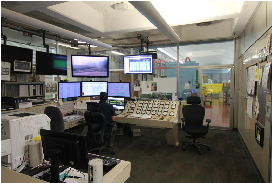
Photo 16 of 25: (WA_PendOreille_BoundaryDam__016) INTERIOR: Boundary Powerhouse Control Room, camera-looking E, toward main floor of the Machine Hall (K)
