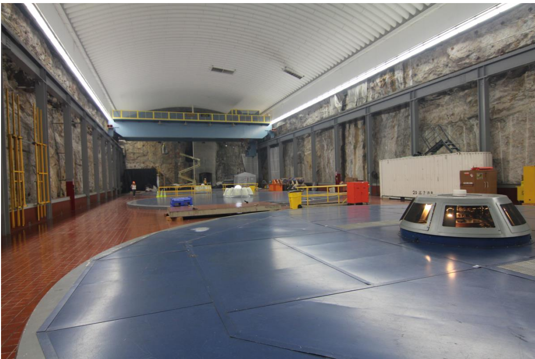
Photo 15 of 25: (WA_PendOreille_BoundaryDam_015) INTERIOR: Boundary Powerhouse/Machine Hall, Units 54, 55 and 56, camera looking E (K)
