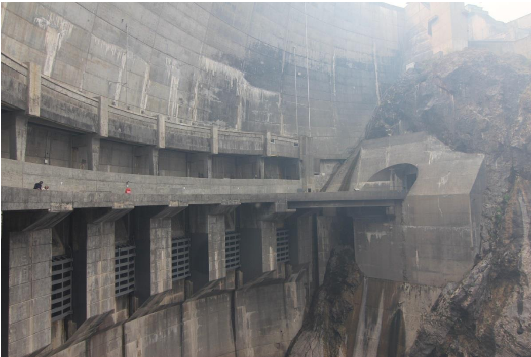
Photo 9 of 25: (WA_PendOreille_BoundaryDam__009) Boundary Dam, downstream face showing sluice gates, cantilever roadway, camera looking SW from Right Abutment at roadway level (K)
