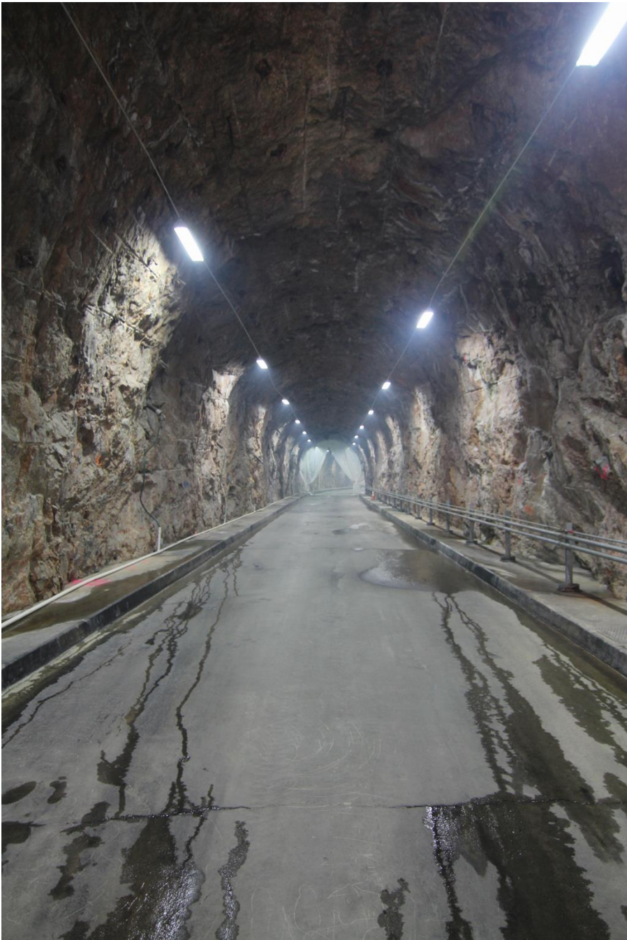
Photo 12 of 25: (WA_PendOreille_BoundaryDam_012) INTERIOR: Dam Access Tunnel, camera looking SE from near entry (K)
