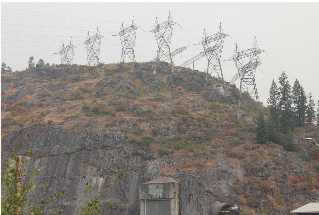
Photo 22 of 25: (WA_PendOreille_BoundaryDam__022) Boundary Dam Transmission Line, camera looking N from Forebay (K)
