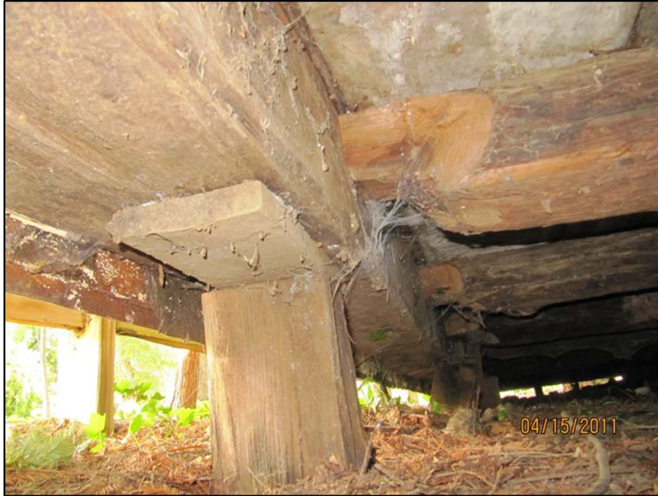
Figure 21. Cunningham House original foundation showing mortise and tenon floor joists, view to southeast, 2011 (Photographer Steve Lehmann)
