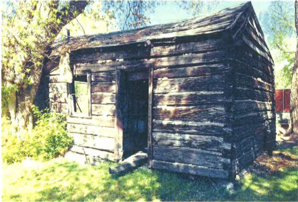
E01 Front (West) elevation of the cabin 04/22/2016 Hawk Log Cabin, 458 North 300 West, Salt Lake City, Utah 84103
