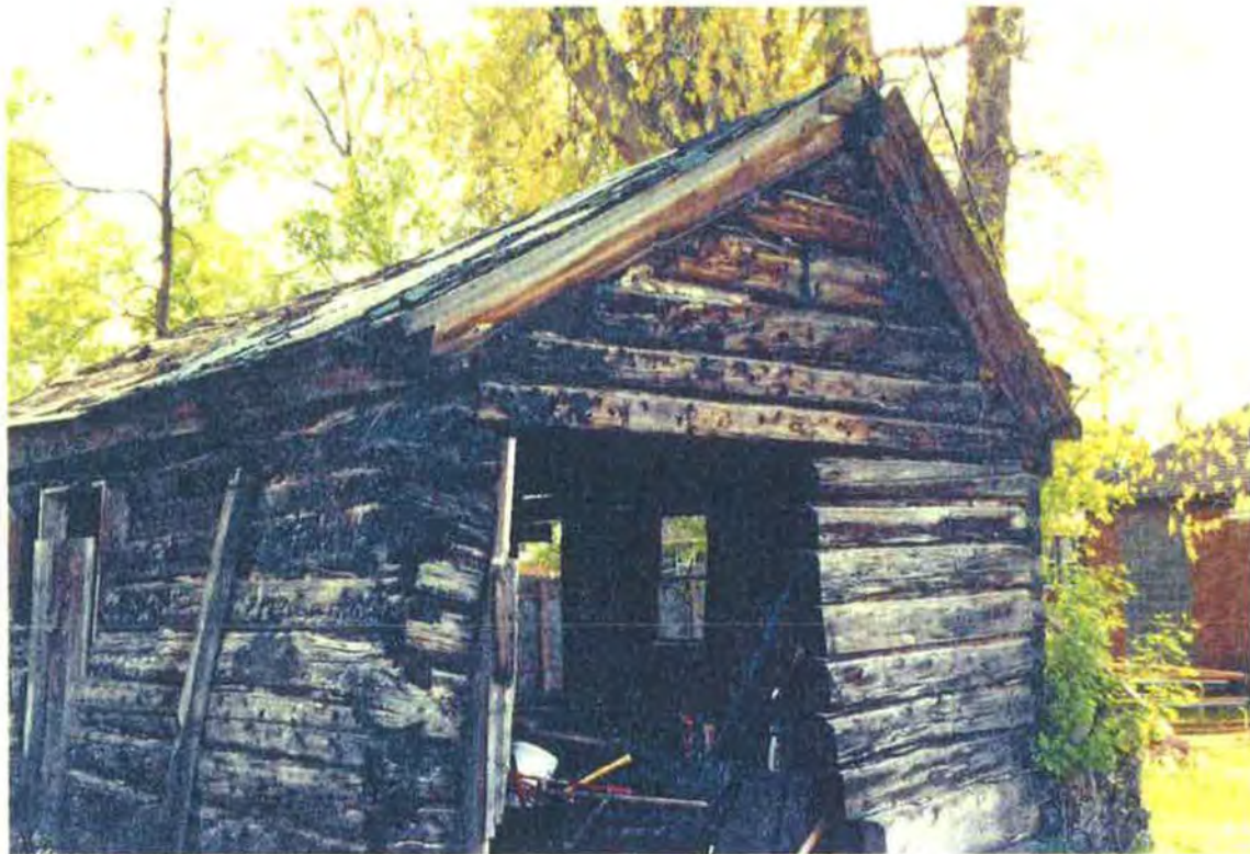
E04 Side (North) elevation of the cabin 04/22/2016 Hawk Log Cabin, 458 North 300 West, Salt Lake City, Utah 84103
