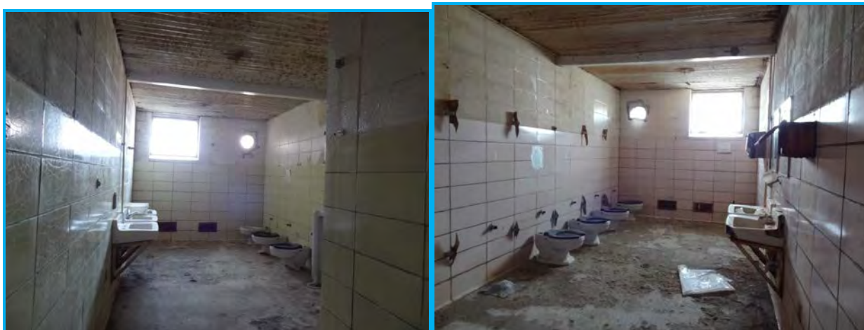
Figure 29. Boys' (left) and girls' (right) bathrooms. Camera facing northwest. Photographed by the author, December 15-16, 2016.
