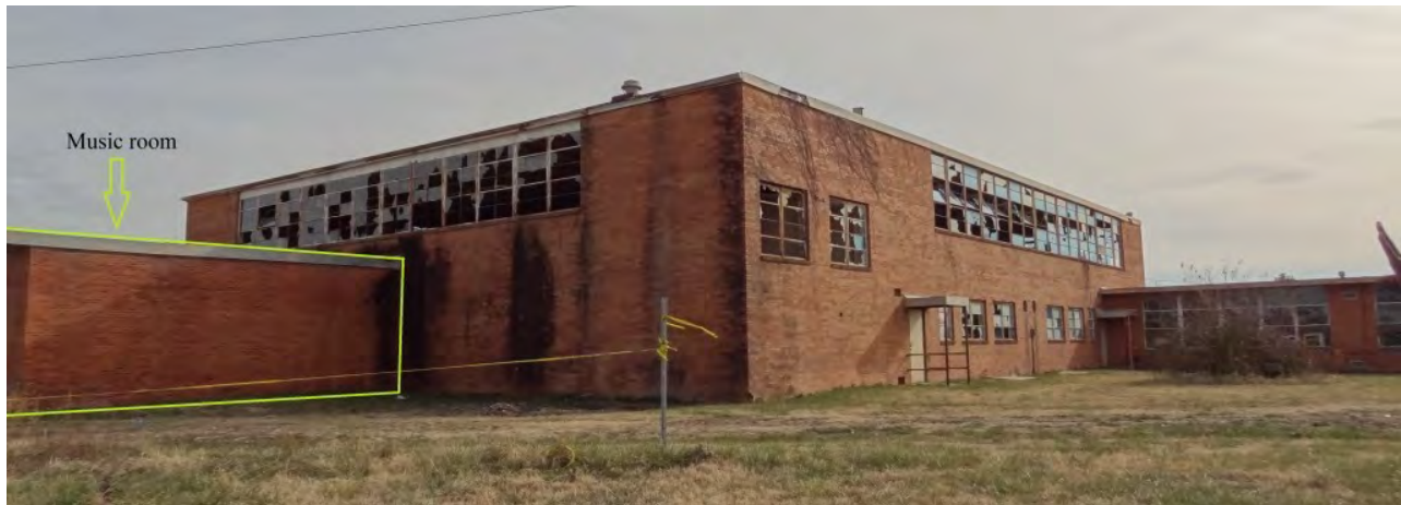
Figure 18. The west elevation of the music room, the north and west elevations of the gymnasium, and a portion of the one story western section of the high school (on the right). Facing southeast. Photographed by the author, December 15-16, 2016.
