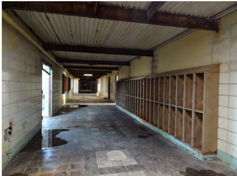
Figure 27. High school double-loaded corridor. Note wall tiling and lockers still largely intact. All lighting is from the expanses of windows located in the classrooms. Camera facing northeast. Photographed by the author, December 15-16, 2016.
