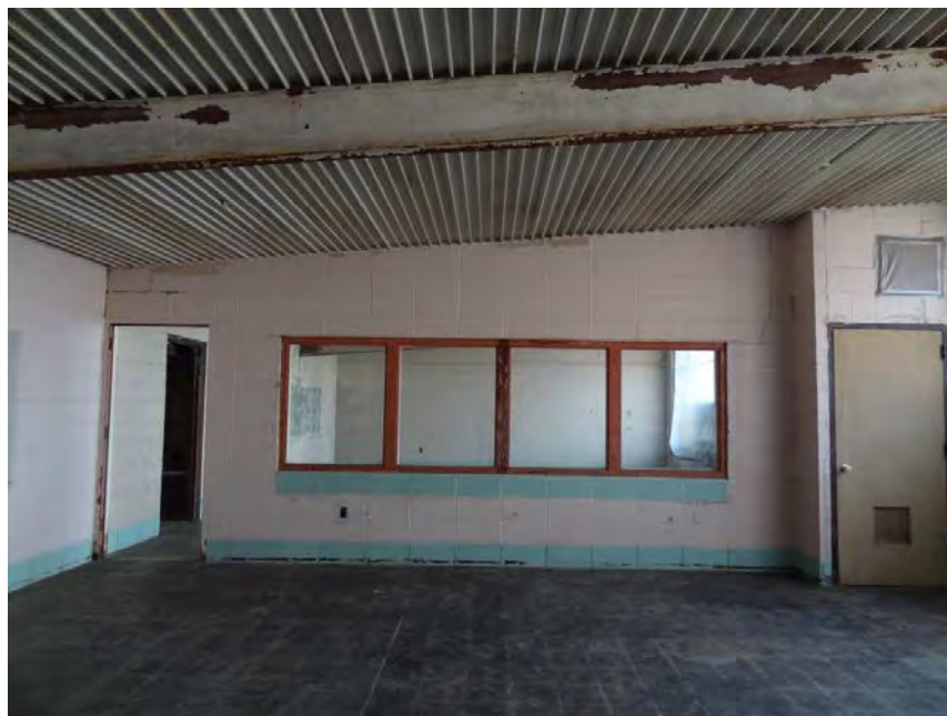
Figure 32. Shared classroom wall with windows still intact. Camera facing southwest. Photographed by the author, December 15-16, 2016.
