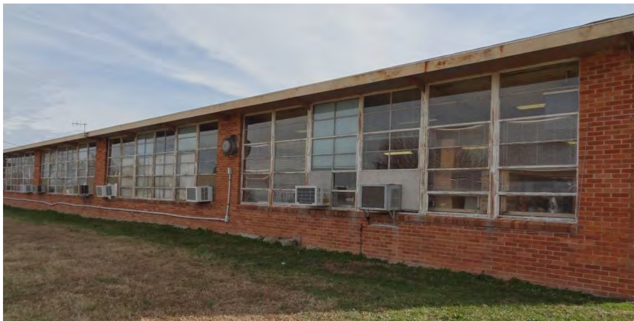
Figure 25. The taller eastern half of the north elevation of the elementary school building. Camera facing southeast. Photographed by the author, December 15-16, 2016.
