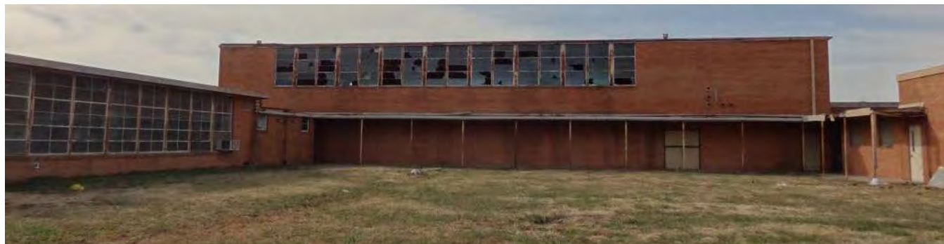
Figure 15. Northern elevation of east end of high school and eastern elevation of the two-story gymnasium. Camera facing southwest. Photographed by the author, December 15-16, 2016.
