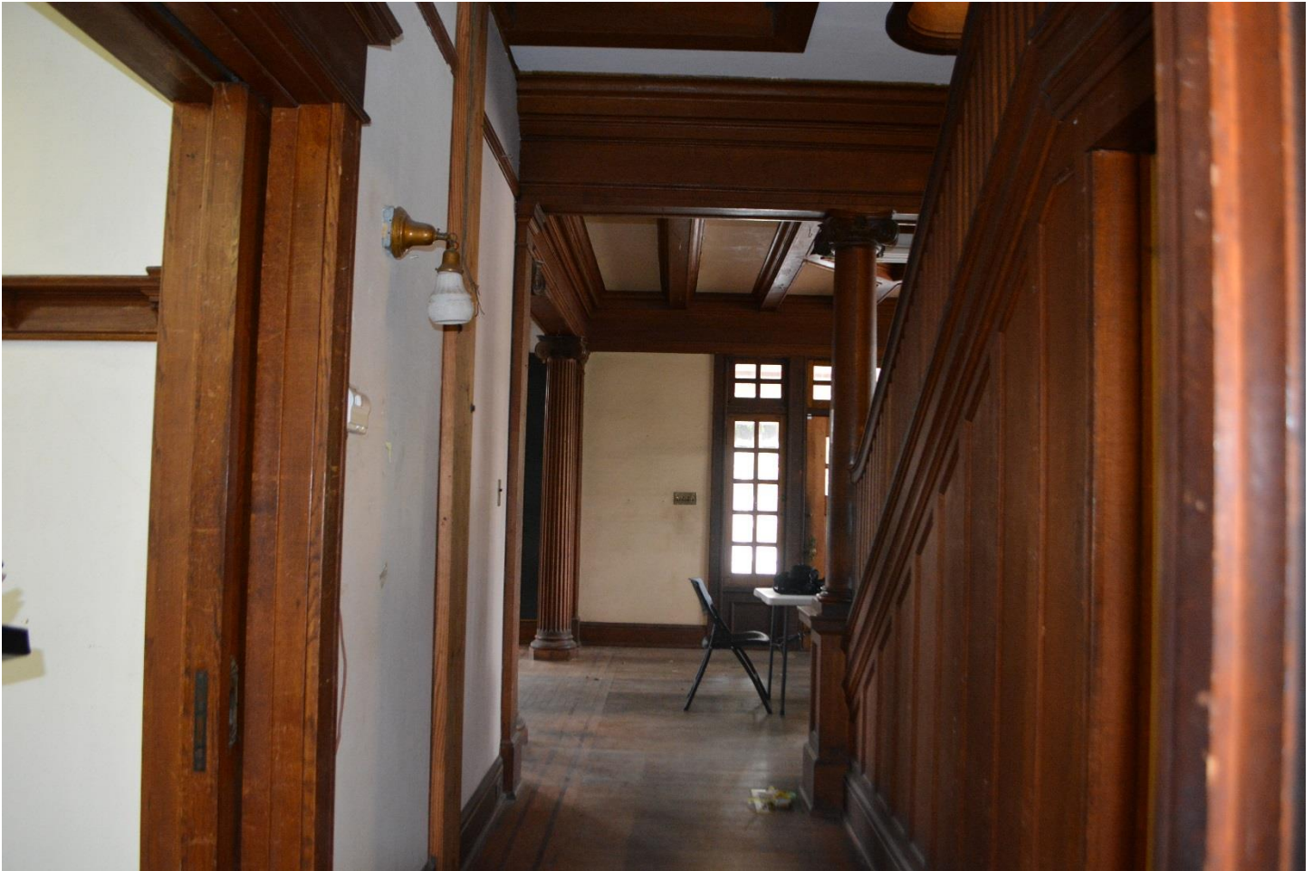
Photo 11 - Interior, first floor stair hall view south. The unfinished wood on the wall and the change in ceiling materials above indicates this as the elevator's original location.
