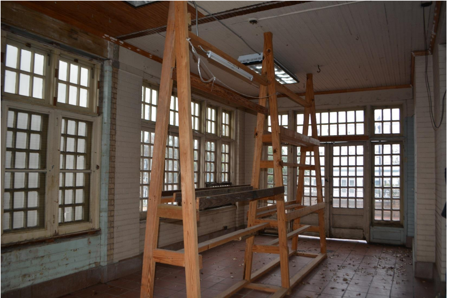
Photo 10 - Interior, first floor east porch, view southeast. A visible line on the wall and ceiling shows where the room was once subdivided.
