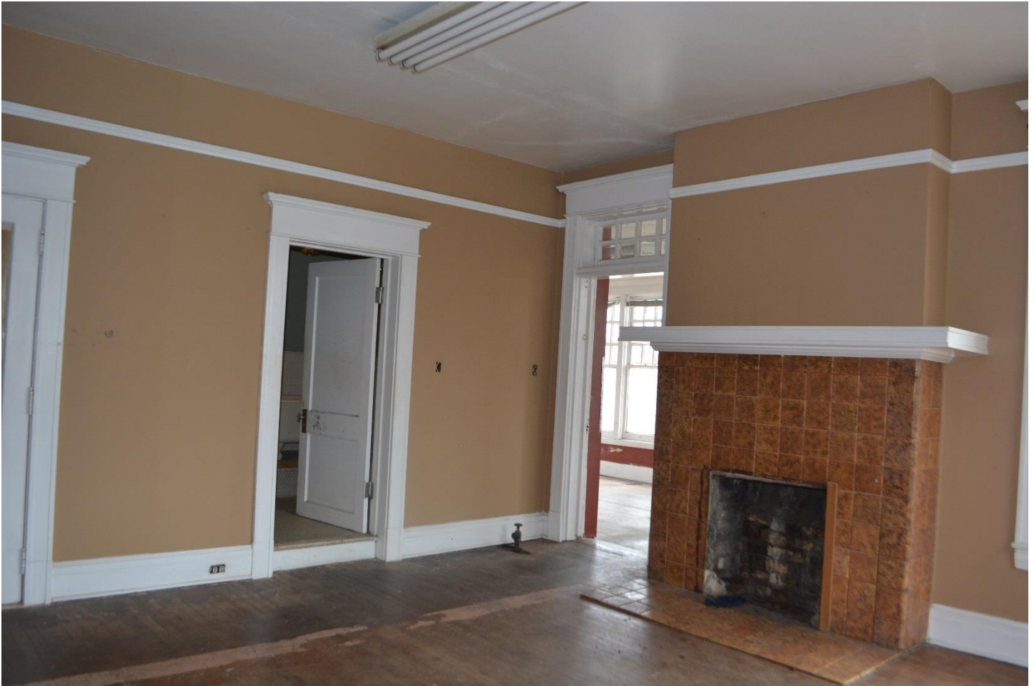
Photo 12 – Interior, second floor bedroom with fireplace, view northeast. A line on the floor indicates where there may once have been a wall to create a hallway to the porch (background).
