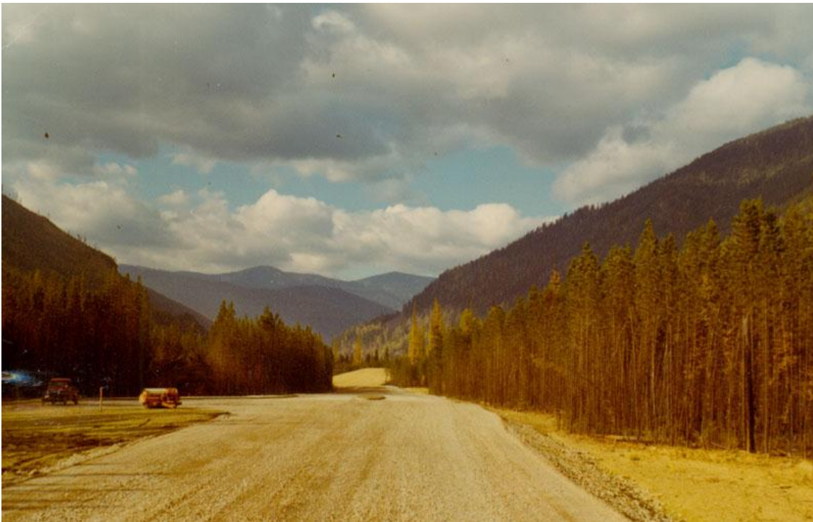
Figure #3: Entrance plaza area near west end of the Camas Road, construction view, with curbing and traffic island in place.
