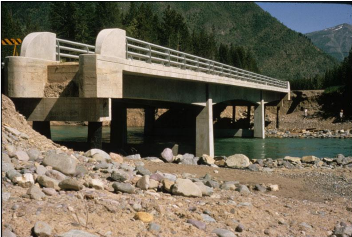
Figure #5: McDonald Creek Bridge, showing bank erosion caused by the June 1964 flood.
