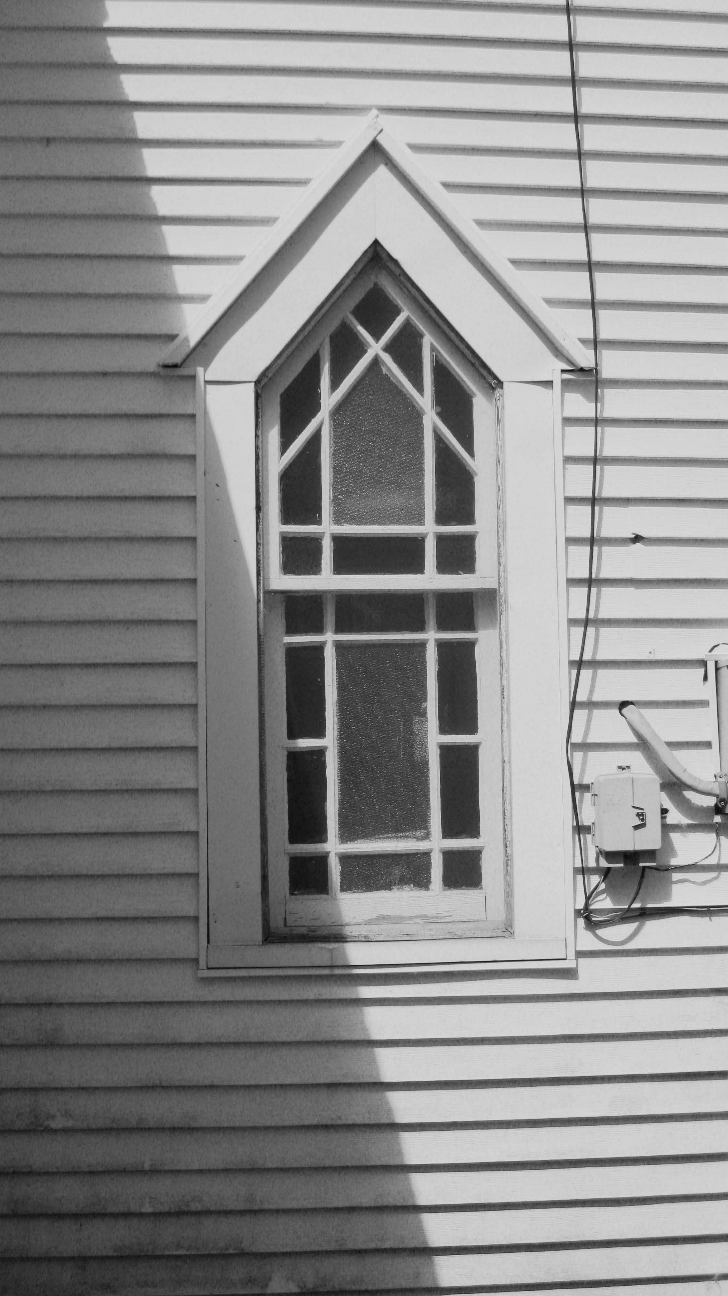
DE_Kent County_St. Paul A.M.E. Church c. 1948 stained glass apse window reinstalled in south elevation of expanded altar area 06 of 13
