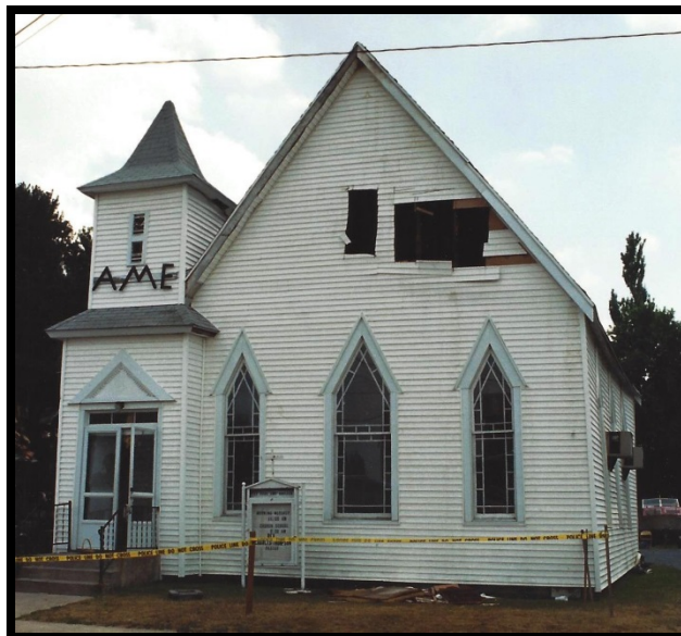
Fire and smoke damage caused by a fire in neighboring house in July of 1993. Fire fighters cut smoke ventilation holes in main façade.
