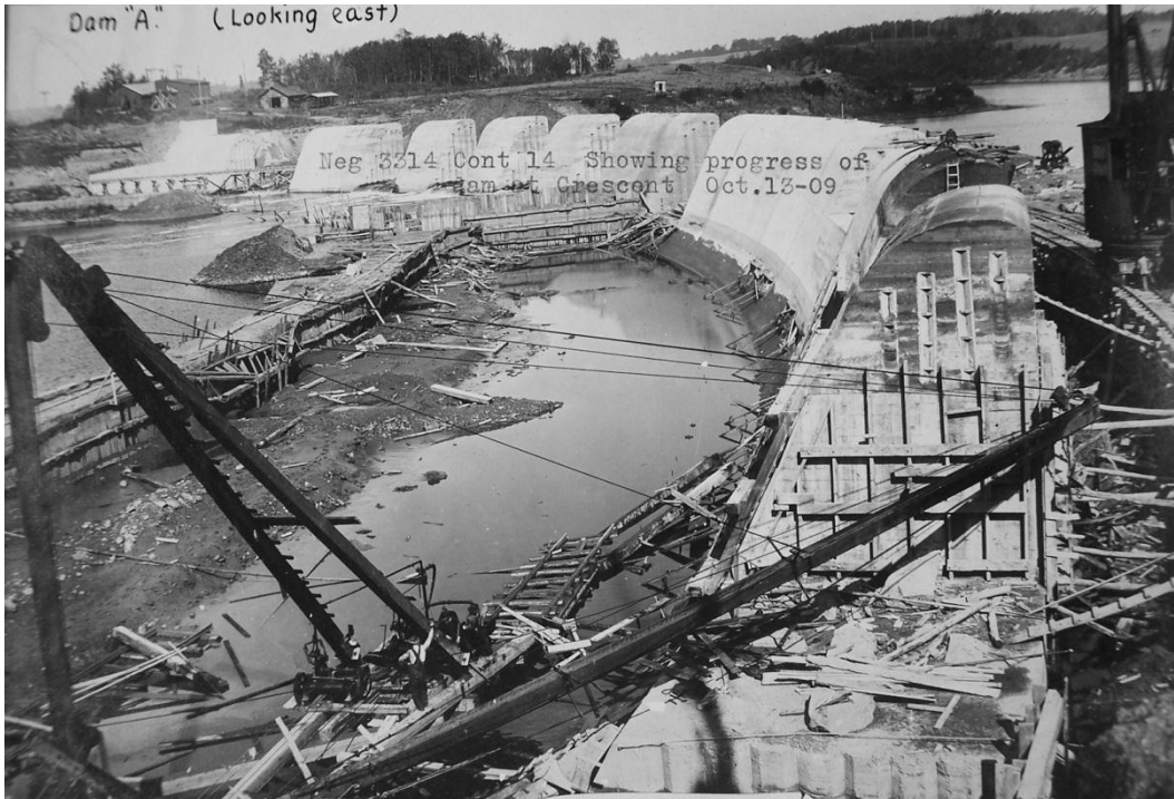
Figure 32 - Erie Canal/Mohawk River, Crescent Dam, towns of Waterford, Saratoga County and Colonie, Albany County, October 13, 1909 (contract 14) View looking from Waterford toward Colonie
