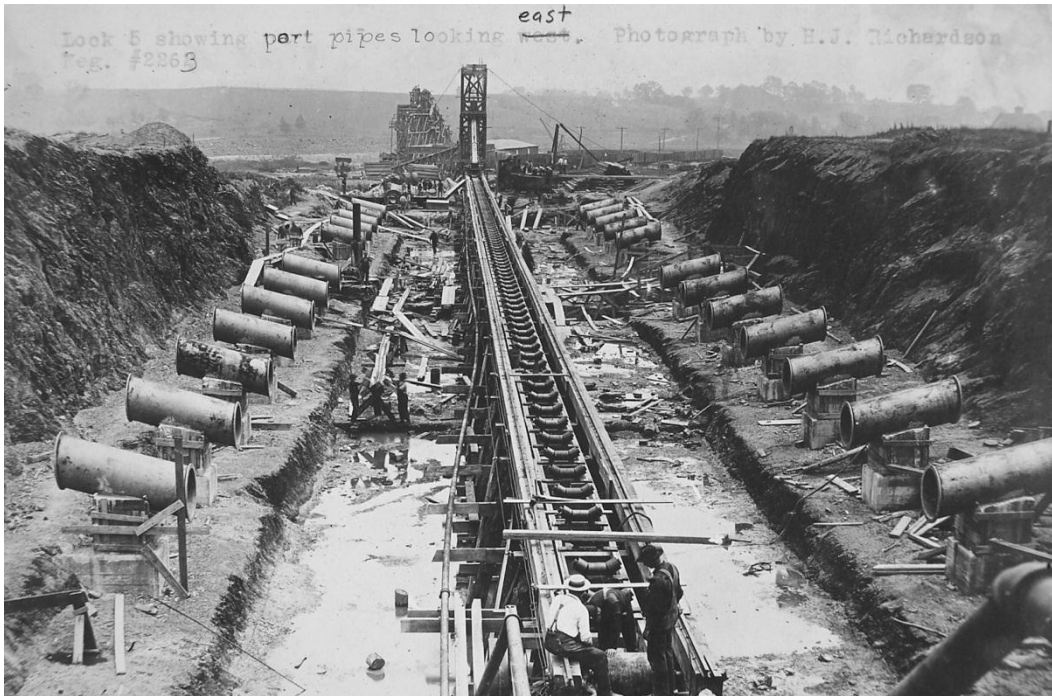
Figure 11 - Erie Canal, Lock E5, Waterford, Saratoga County – lock filling tubes placed before first concrete pour, August 1907 (Contract 11)
