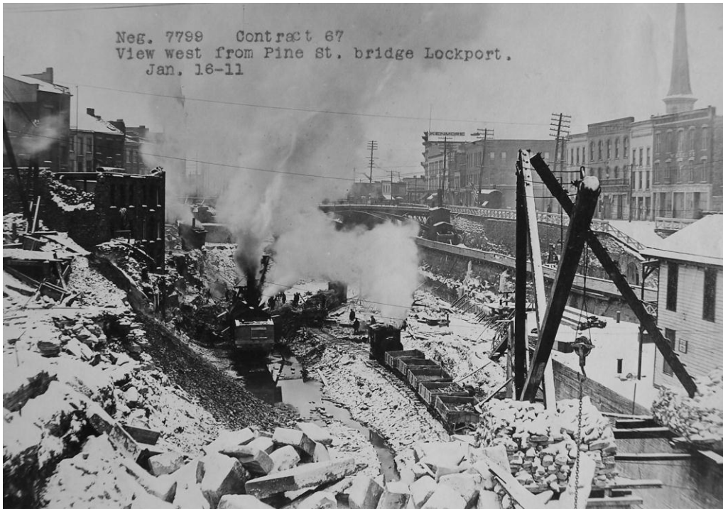
Figure 25 – Erie Canal, excavation above Lock E35, Lockport, Niagara County, January 16, 1911 (Contract 67) View looking west from Pine Street bridge.
