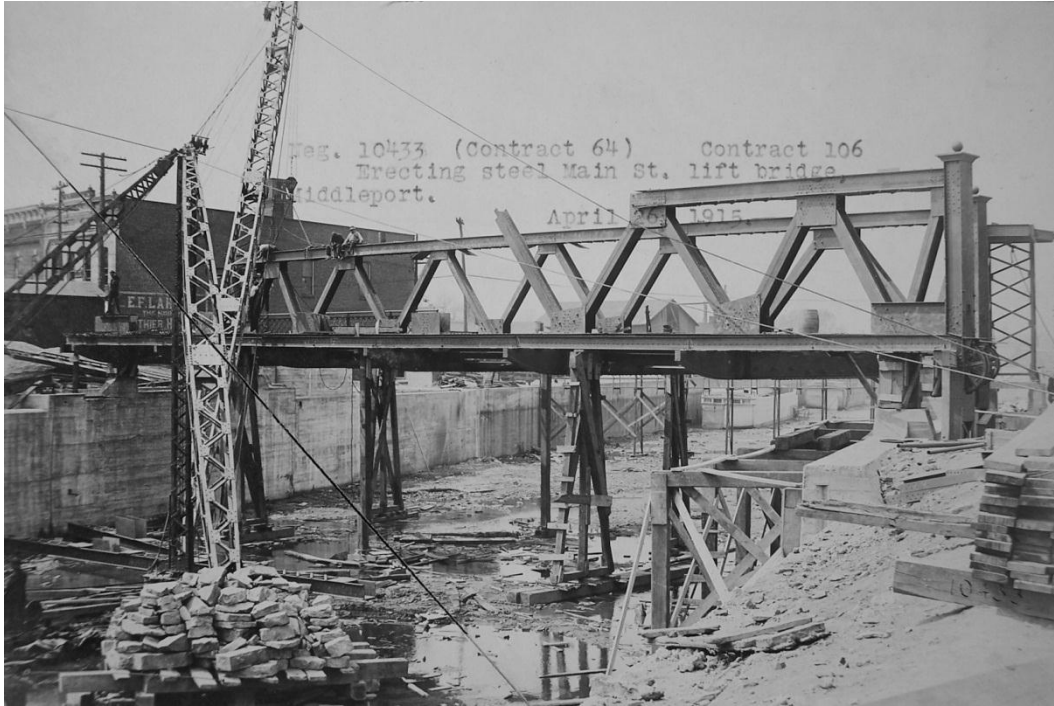
Figure 42 – Erecting steel, Main Street lift bridge over Erie Canal, Middleport, Niagara County, April 26, 1915 (Contract 67)
