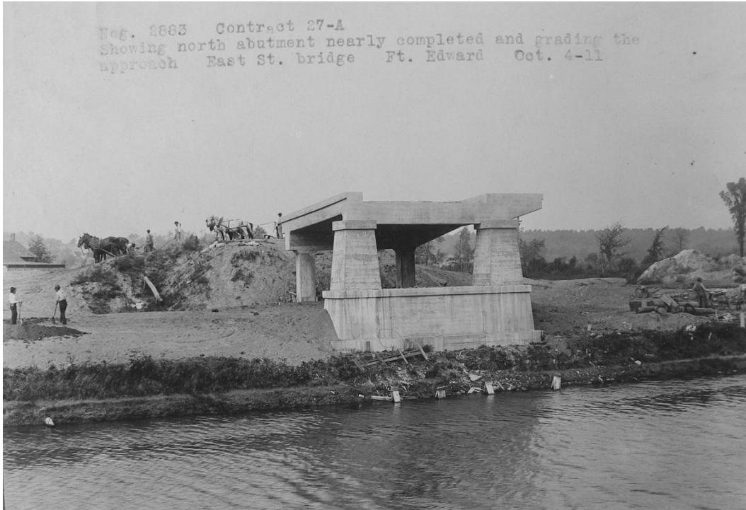
Figure 38 – East Street Bridge over Champlain Canal, Fort Edward, Washington County, October 4, 1911 (Contract 27-A) The State Engineer's office developed this design for reinforced concrete piers and approach slabs that was widely used along land-cut sections of the Barge Canal. Reportedly, it cost about 25% less than conventional abutments.
