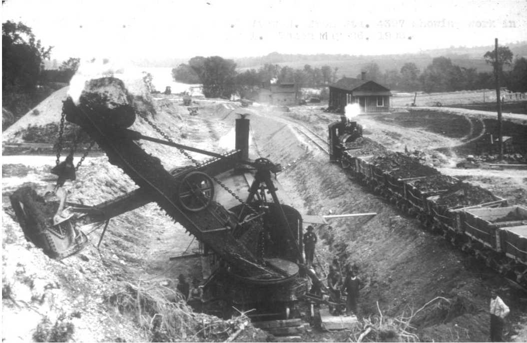
Figure 6 – Erie Canal, excavator working on the “Anthony Cut” west of Oneida Lake, Onondaga County, May 26, 1908 (Contract 12)
