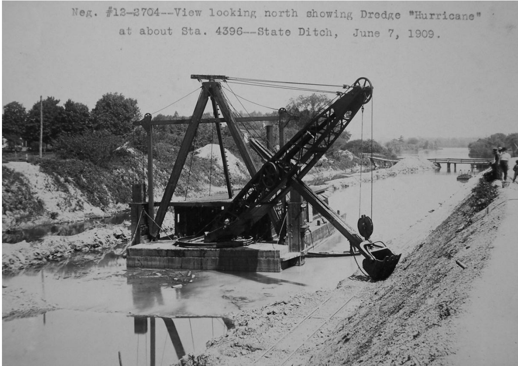
Figure 8 – Erie Canal, Dipper Dredge Hurricane widening the “State Ditch” west of Baldwinsville, Onondaga County, June 7, 1909 (Contract 5)
