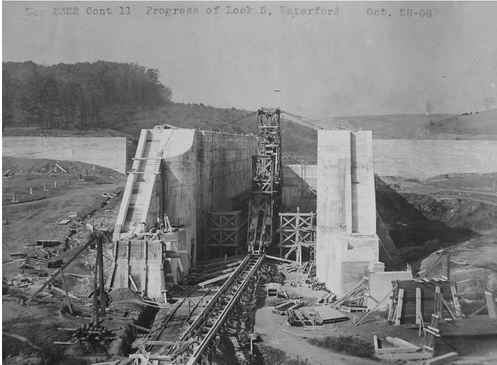
Figure 13 – Erie Canal, Lock E5, Waterford, Saratoga County –October 28, 1908 (Contract 11) Concrete lock walls and core for earthen dam nearly complete. Lock floor remains to be poured.
