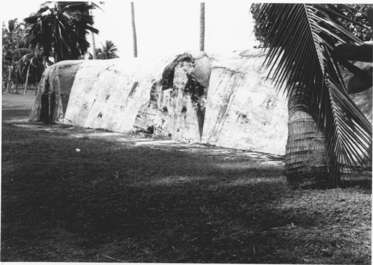
4. Partly-demolished Japanese air raid shelter on Roi. This standard design may yet be found on other Pacific Islands, including two survivors on adjacent Namur.
