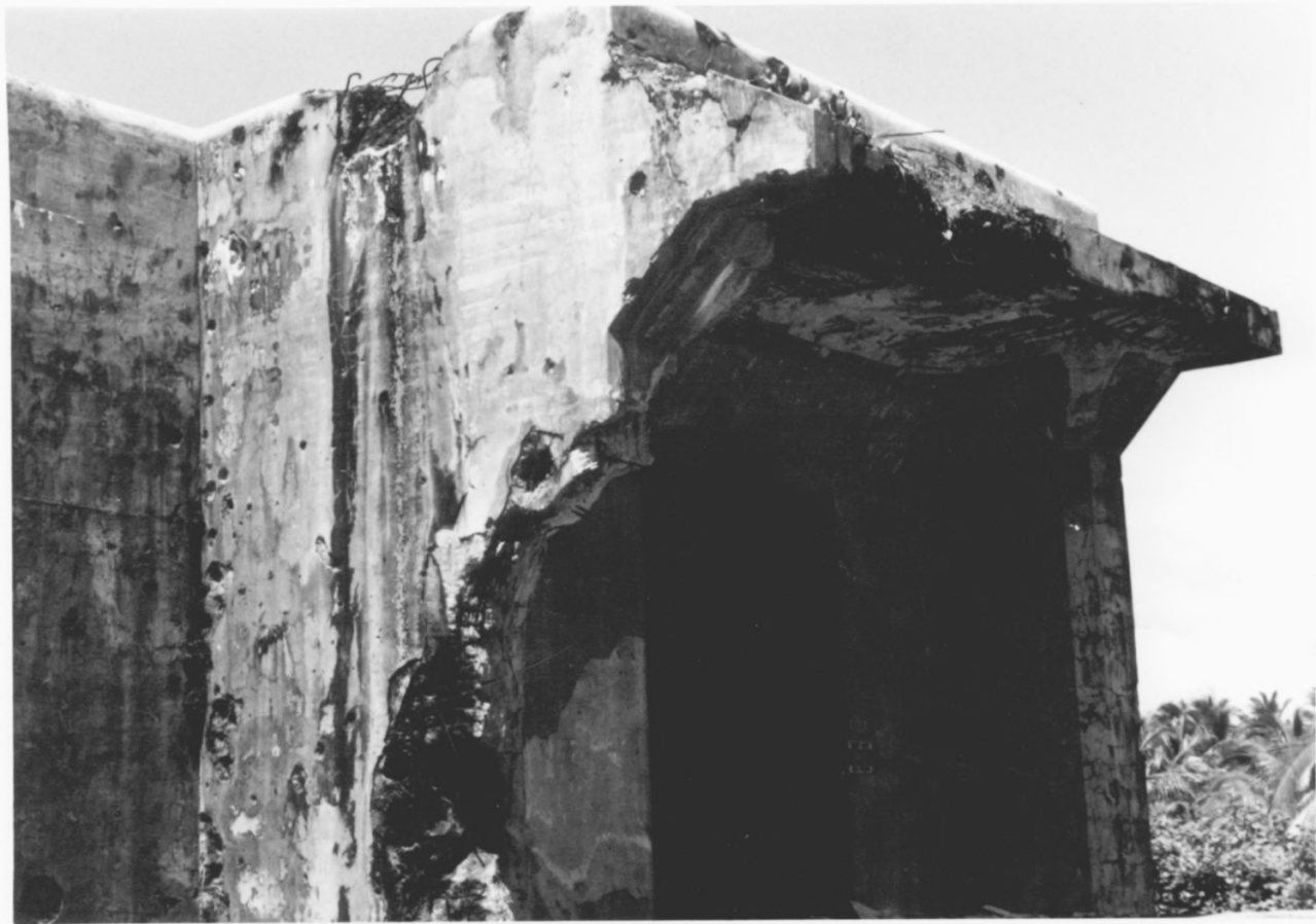
9. The same magazine today without its steel doors. Although not visible in this photograph, the hole leading under the structure is extant.
