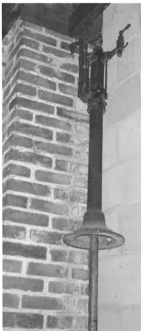
Cast iron pump leaning against wall on 2nd floor
