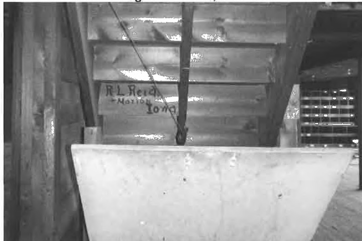
Detail of graffiti on backside of stairs to 3rd floor
