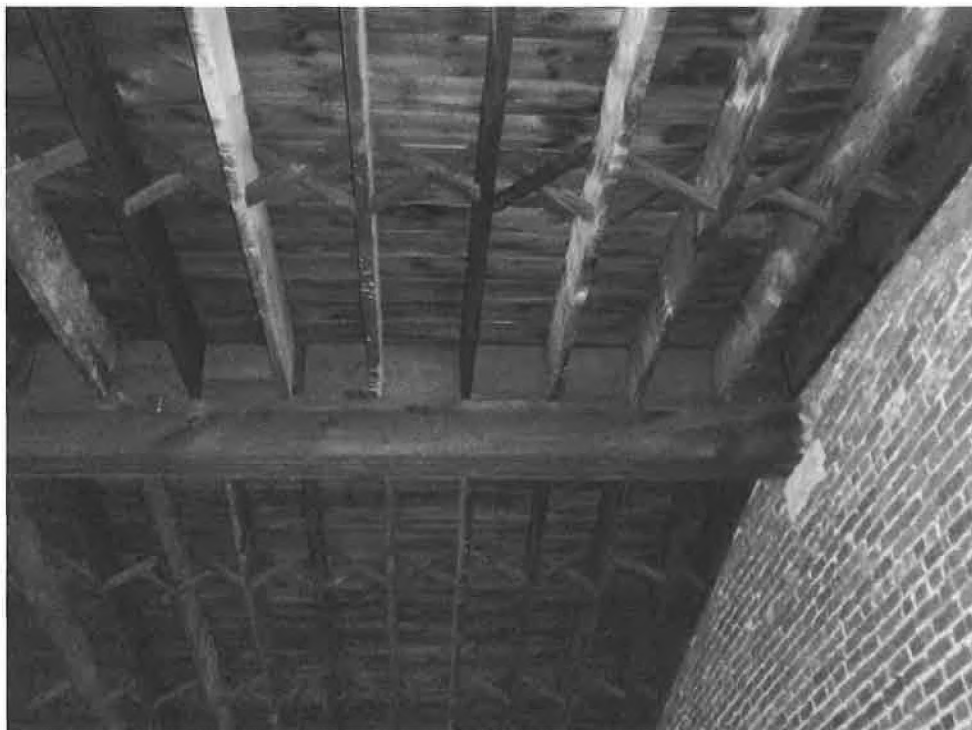
Detail of rafters and framing on 3rd floor, view to NNW at east end wall
