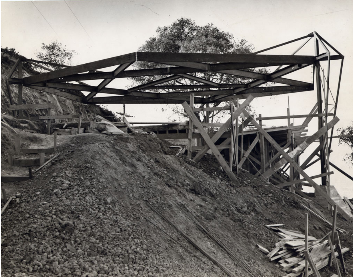
View of prefabricated roof structure, facing southeast (© The John Lautner Foundation, courtesy of Frank Escher, 1948)
