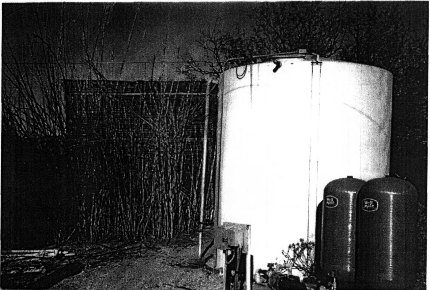
PHOTO #36 (Neg # DWR-2-3): Pumphouse (l) and storage tank (r) looking NW (ineligible)
