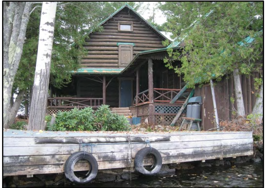
Figure 5: East elevation, showing main section and kitchen with attached shed (at right) and dock, 2016
