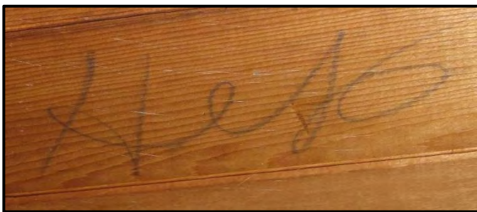
Figure 15. “Hess” on ceiling boards, second floor, Dollar Island Camp, 2016.
