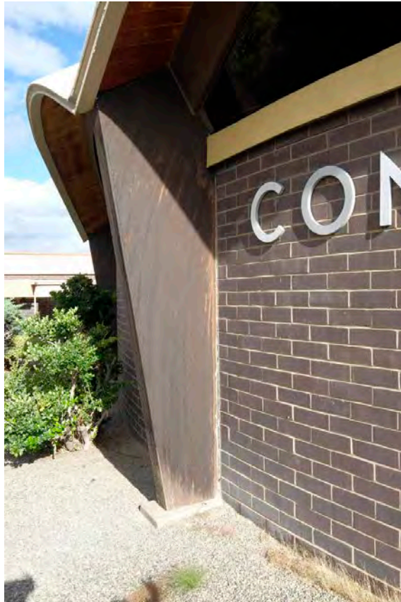
5. Laminated timber arch leg (detail) and Summit utility brick, photographer facing southwest.
