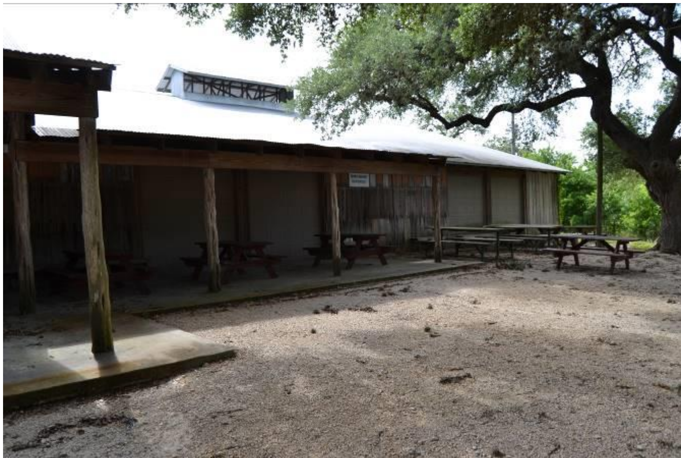
Photo No. 10. View of 1951 rear addition on side east façade of Anhalt Hall, view facing northwest.
