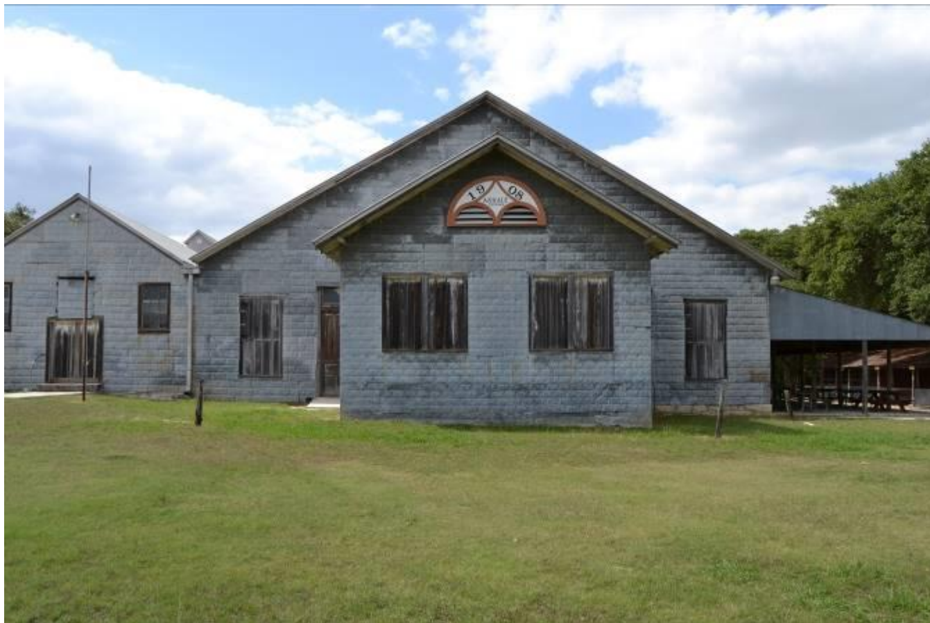
Photo No. 7. View eastern half of main south façade of Anhalt Hall, view facing north.
