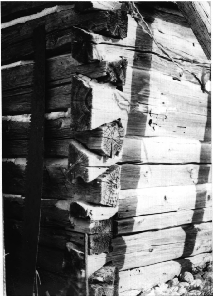
Detail of Log Cabin (HS 14-104A), west corner Manitou Camp Manitou Island, WI
