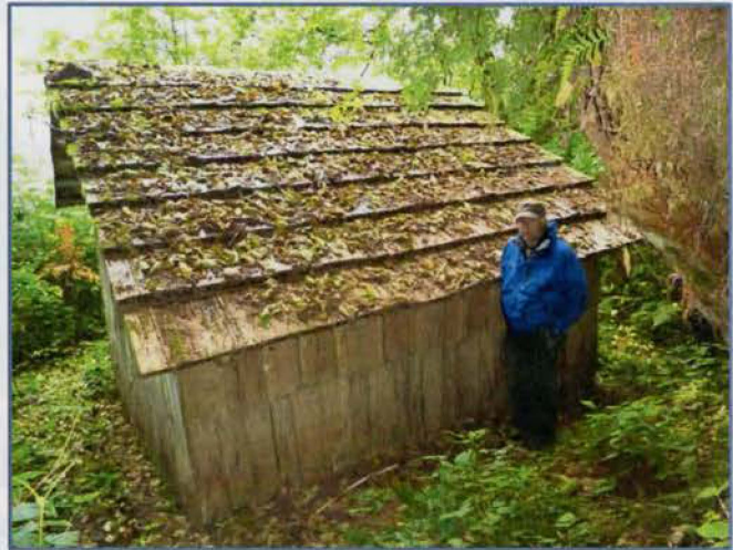
Figure 7 Windfall Shelter West Elevation with Wilderness Ranger Don MacDougall Sept 23, 2010 (FS Photo P1010648.JPG)
