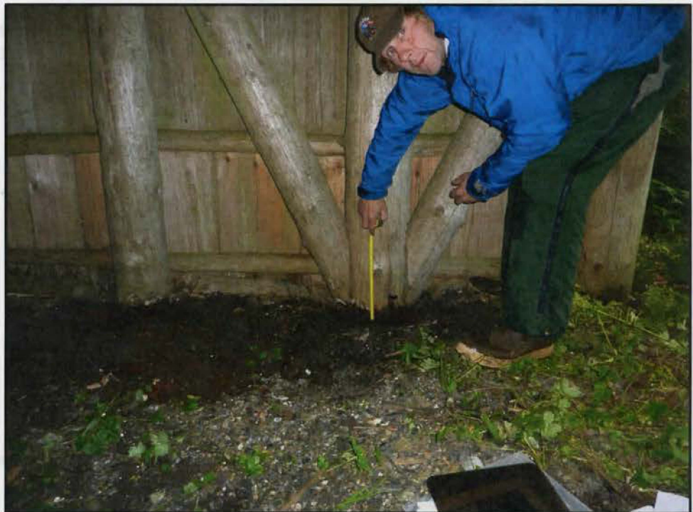
Figure 8: Wilderness Ranger D. MacDougall Assessing Condition of Posts on North Elevation (FS photo P1010643.JPG 09/23/2010)
