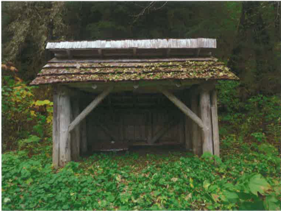
Photo taken October 2009 prior to the shelter move. Front facade of the shelter, shown in its original location within the forest fringe.
