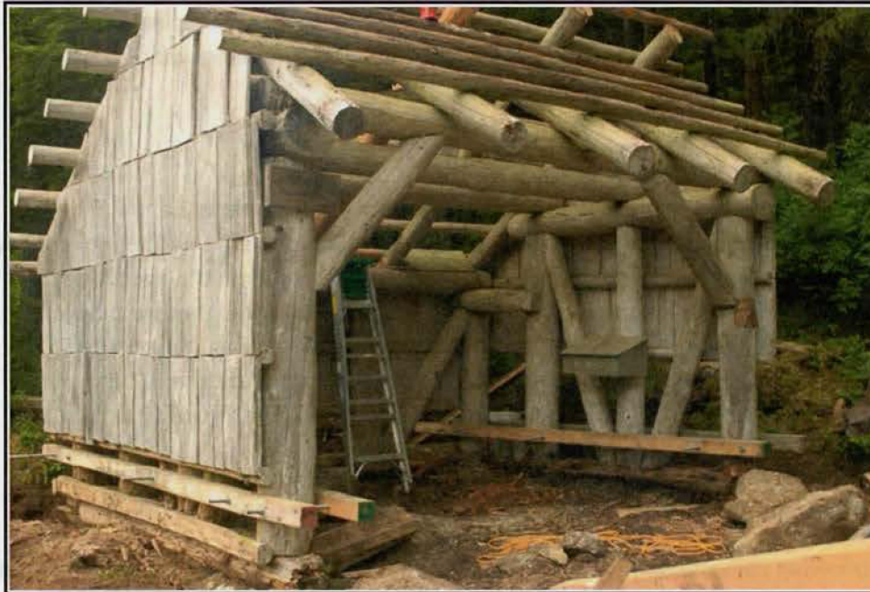
Figure 13: Davidson Lake Shelter During Rehabilitation Project. Photo taken by R. Marek August 13, 2010 (USFS Photo #DSC_0045)
