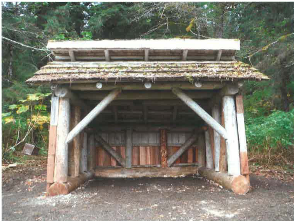
Photo taken September 2014 following the shelter move. Front facade of the shelter, moved forward from within the forest fringe to the more exposed beach location.
