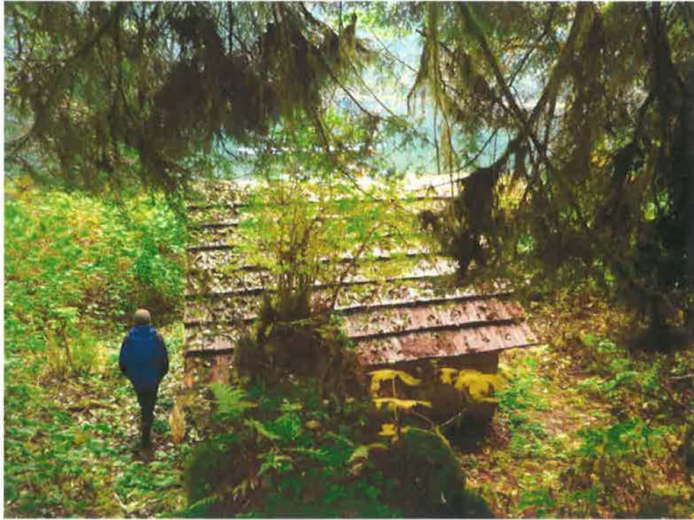
Photo taken October 2009 prior to the shelter move. View of the rear façade of the shelter in its original location.
