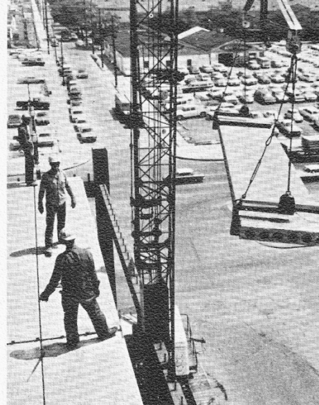
Men wait atop concrete decks to guide floor plank into position on steel beams.
