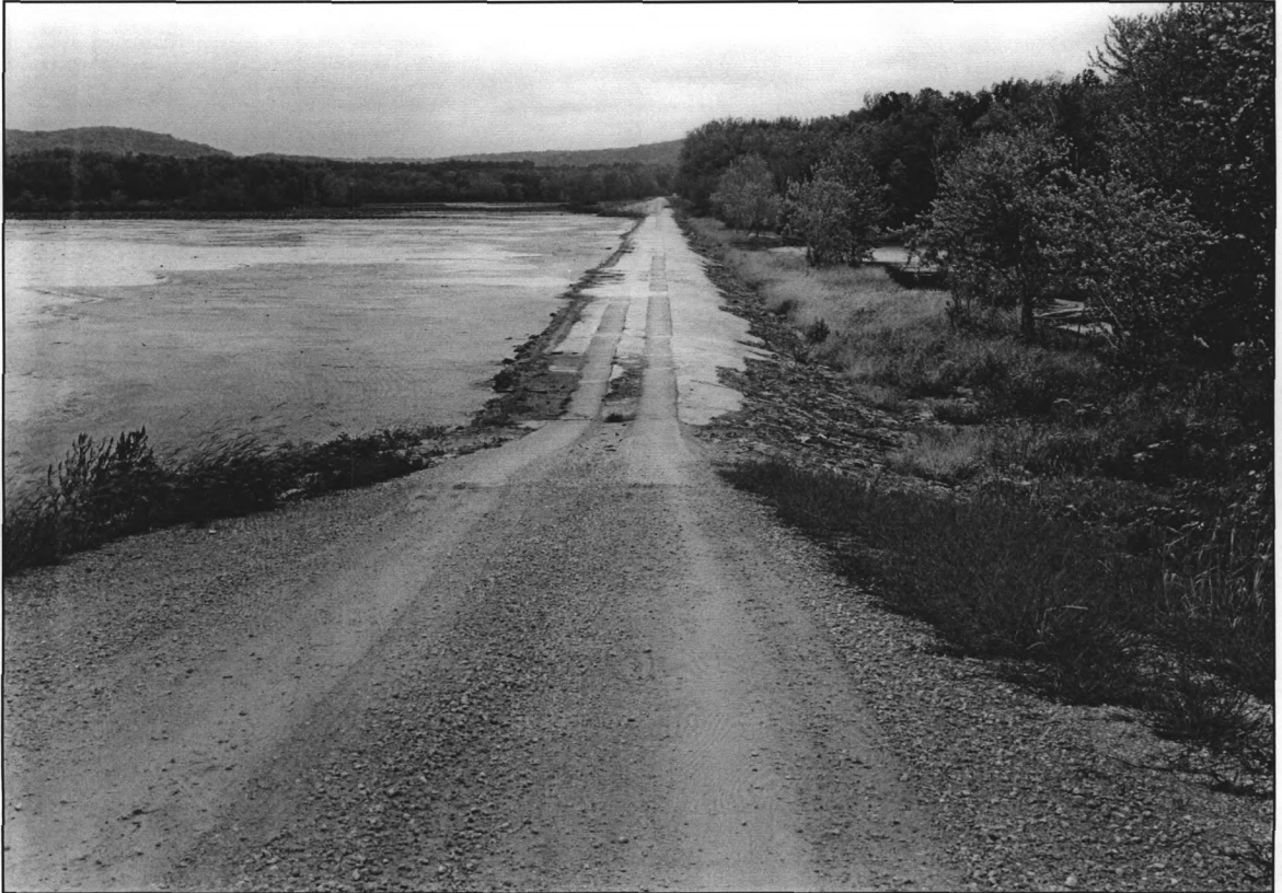
PHOTO 4. Detail of the Stationary Section of Dam No 12. Concrete covered ogee spillway submersible earth- and sand-filled dike, which is the middle of the five dikes which make up the stationary portion of the dam. Photographer: Peter A. Rathbun Date of Photograph: September 1987 Location of Original Negative: IA-24-5, HAER, IOWA, 49-BEL,1- HAER Collection, Prints and Photographs Division, Library of Congress, Washington, D.C. View: From east end of first dike in the series, looking northeast
