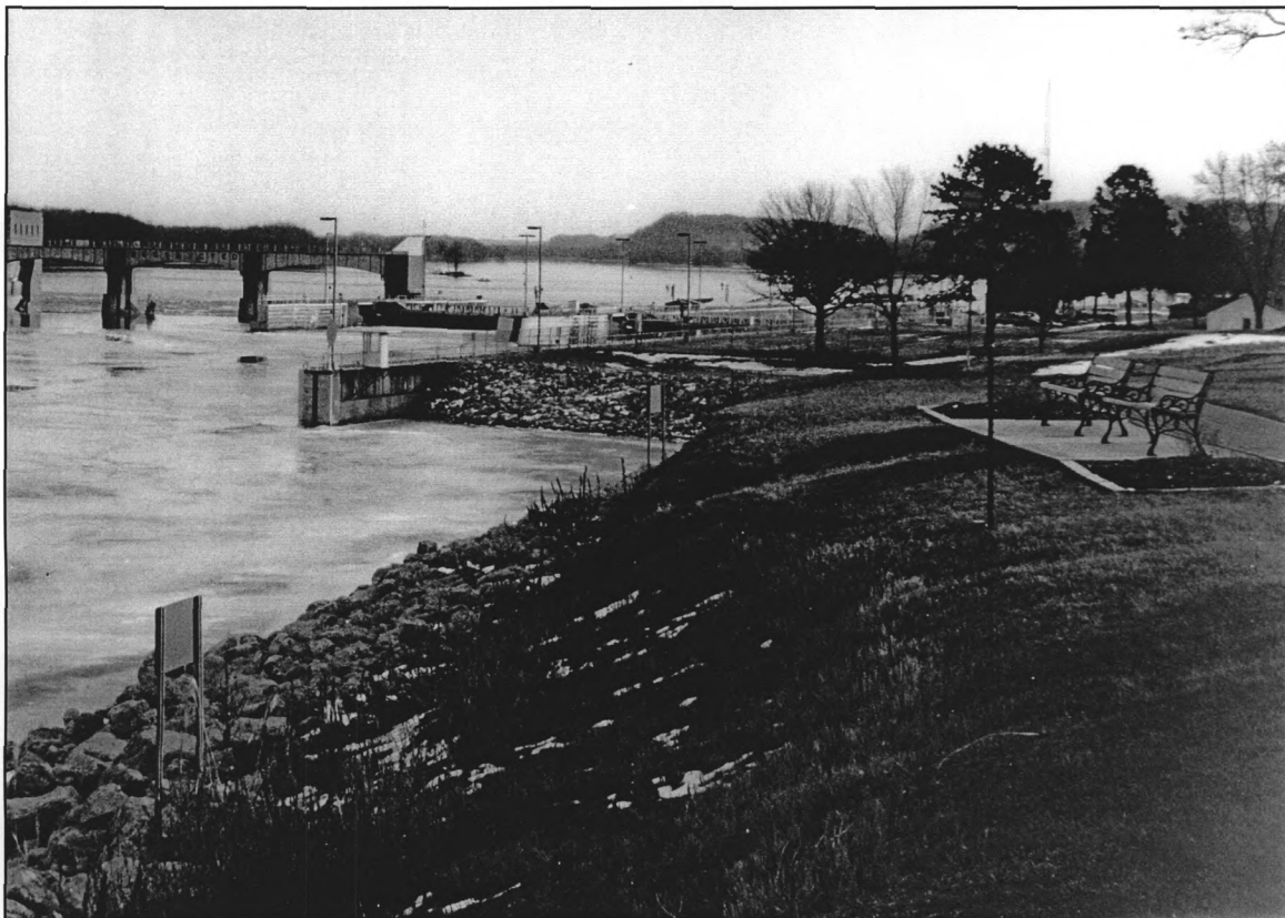
PHOTO 6. Upper Approach Mooring Levee with Recently Repaired Upstream End of the Guide Wall Extension to the Lock and the Moveable Section of the Dam in the Background. New rock surface on the levee visible. Photographer: Mary Yeater Rathbun Date of Photograph: February 1998 Location of Original Negative: URM-NATIONAL REGISTER, roll #1, frame 24, Environmental Impact Section, Planning Division, Rock Island District, U.S. Army Corps of Engineers, Rock Island, IL. View: From village's riverside park, looking southeast
