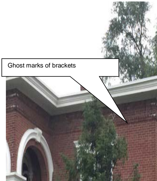
Figure 10. Overhang with ghost marks of brackets
