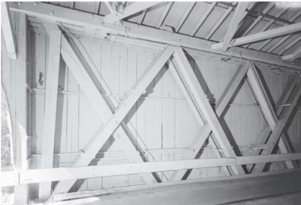
Figure 5.43 The Powder Works Bridge, built in 1872 by the Pacific Bridge Company, is a 180-foot Smith “triple truss” (Wilson type 4). One set of diagonals is sandwiched between and offset from two other sets of web members, connecting to four-piece chords. The image also shows the extra, inclined compression brace on the end panel, common to most Smith trusses (a block of wood obscures the notched joint). Note Smith-type castings fitted over notched joints in upper lateral braces. HAER CA-313-8, Jet Lowe, photographer, 2004.
