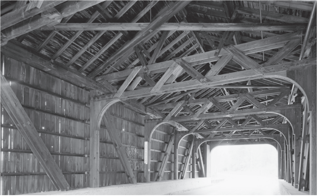
Figure 0.46 The original Hancock-Greenfield Bridge in Hillsborough County, New Hampshire, was destroyed by a flood in 1936. New Hampshire Highway Department engineer Henry B. Pratt Jr. designed a replacement covered bridge that met modern regulations with the use of steel timber connectors manufactured by the Timber Engineering Company (TECO), which allowed the bridge to handle heavier loads. Constructed in 1937 by Hagan Thibodeau Construction using federal funds, this modern TECO truss has the distinction of being the first permanent highway span in the United States to use timber connectors. HAER NH-42-7, Jet Lowe, photographer, 2003.
