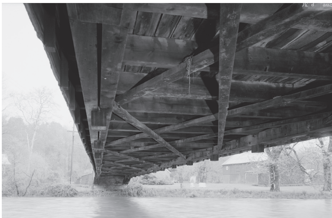
Figure 6.2 Top: 6.2a) Pine Grove Bridge (1884) once illustrated the general pattern of X-braced floor framing found in covered bridges in Lancaster County, Pennsylvania. Since the decking and stone abutments have been replaced by steel beams and concrete, these floor details no longer exist. HAER PA-586-2, Jet Lowe, photographer, 2002. Above: 6.2b) On the other hand, Dreibelbis Station Bridge (1869) retains the three-panel-long latticed style floor framing typical of covered bridges erected in Berks County, Pennsylvania. HAER PA-587-7, Jet Lowe, photographer, 2002.
