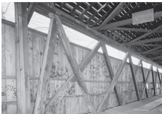
Figure 5.41 Kidd's Mill Bridge (1868) is a 122-foot-long Smith "double truss" (Wilson type 2). Note the steeply inclined extra brace at the end panel, with a lightning bolt shaped notch. HAER PA-622-5, Jet Lowe, photographer, 2006.
