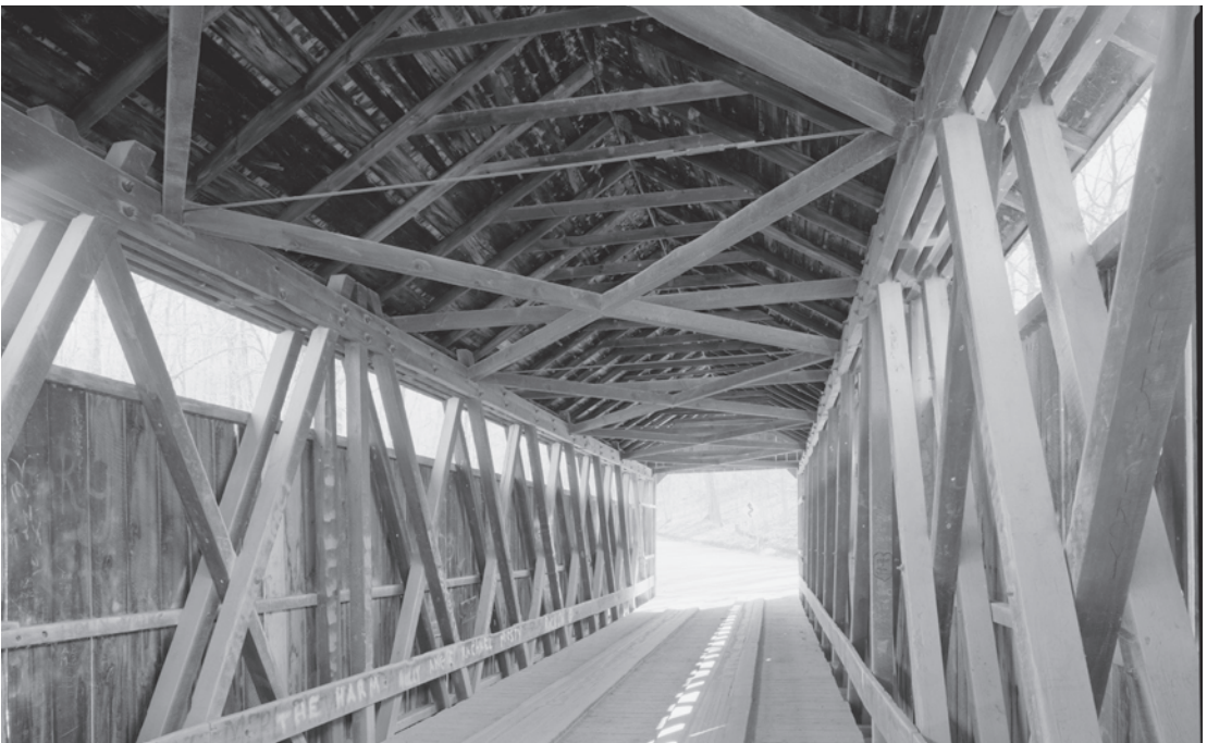
Figure 0.43 White's Bridge (1869) in Kent County, Michigan, was the best surviving example of this truss patented in 1857 by Josiah Brown before it was lost in a fire in 2013. The regional Brown truss featured paired braces and single counters notched and bolted at the chords. HAER MI-331-8, Jet Lowe, photographer, 2004.
