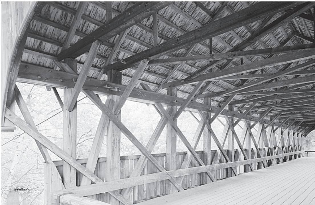
Figure 6.4 Sunday River Bridge (1872) in Oxford County, Maine, is a good example of the Paddleford truss, which became the dominant regional truss in parts of New Hampshire, Maine, and Vermont in the late-nineteenth century. HAER ME-69-11, Jet Lowe, photographer, 2003.
