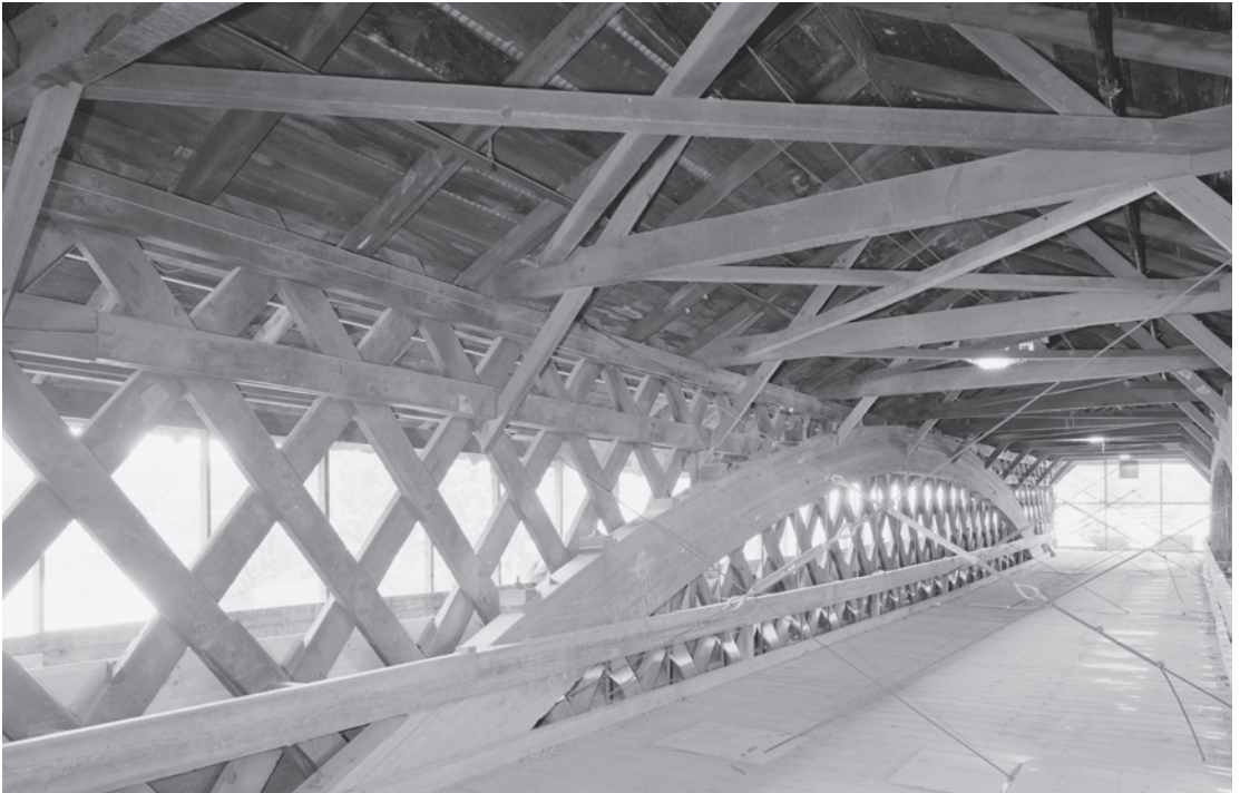
Figure 0.14 Built in 1829, the Bath-Haverhill Bridge in Grafton County, New Hampshire, is the oldest existing Town lattice bridge in the country. The laminated arches were added in 1922 to increase load capacity. HAER NH-33-14, Jet Lowe, photographer, 2003.
