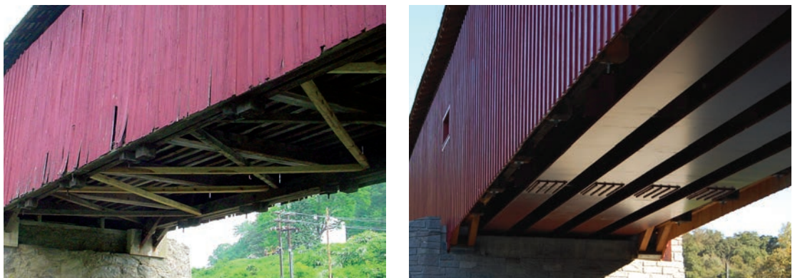
Figure 7.14 In 2002, the HAER documentation team found the original lower chord, lateral bracing, and stone abutments of Pine Grove Bridge in Lancaster County, Pennsylvania, as constructed by Elias McMellen in 1884, still intact. While the Pennsylvania Department of Transportation saved the Burr-arch trusses in 2008, they unfortunately replaced the lower timbers with steel I-beam and removed all of the stonework, constructing new concrete abutments with a form liner surface treatment. Top: 7.14a) HAER field photo, 2002; Above: 7.14b) Tom Vitanza, photographer, 2009.
