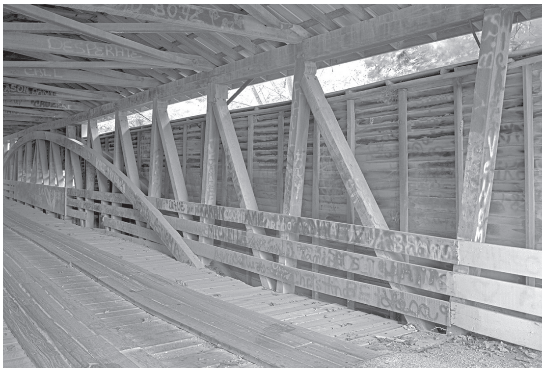
Figure 6.5 Huffman Mills Bridge (1864) in Perry and Spencer counties, Indiana, is a Burr-arch truss with the flared-post style used in the Wernwag tradition. Joseph D. Conwill, photographer, 2003.
