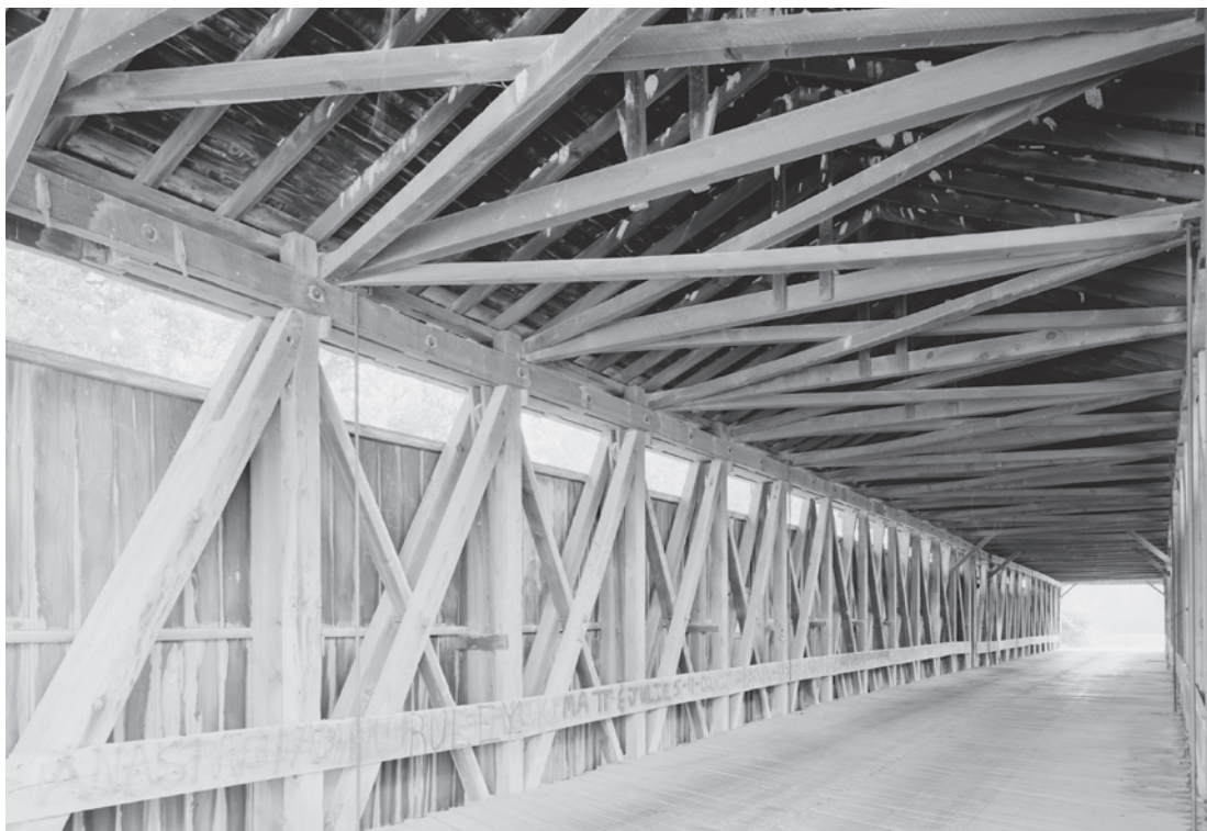
Figure 0.24 The Eldean Bridge (1860) in Miami County, Ohio, is one of the few remaining Long trusses that still retain their adjustable wooden wedges at the counterbrace panel points for prestressing. The designer of the truss, Col. Stephen Long, is credited with introducing mathematical theory to American bridge design. HAER OH-122-10, Jet Lowe, photographer, 2002.
