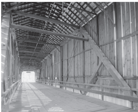
Figure 5.37 A 128-foot-long Pratt truss can be found in the center span of the Honey Run Bridge (ca. 1886), Butte County, California. HAER CA-312-5, Jet Lowe, photographer, 2004.
