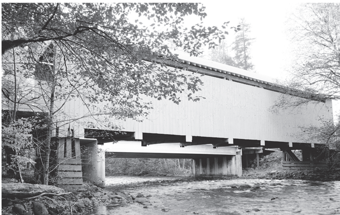
Figure 6.3 Top: 6.3a) The sides of the Howe trusses in Linn County, Oregon, as in Short Bridge (1945), were left open. HAER OR-120-6, Jet Lowe, photographer, 2004. Above: 6.3b) Covered bridges in Lane County, Oregon, like Horse Creek Bridge (1930, moved 1990), were covered nearly to the top chord. HAER OR-15-2, James Norman, photographer, 1987.
