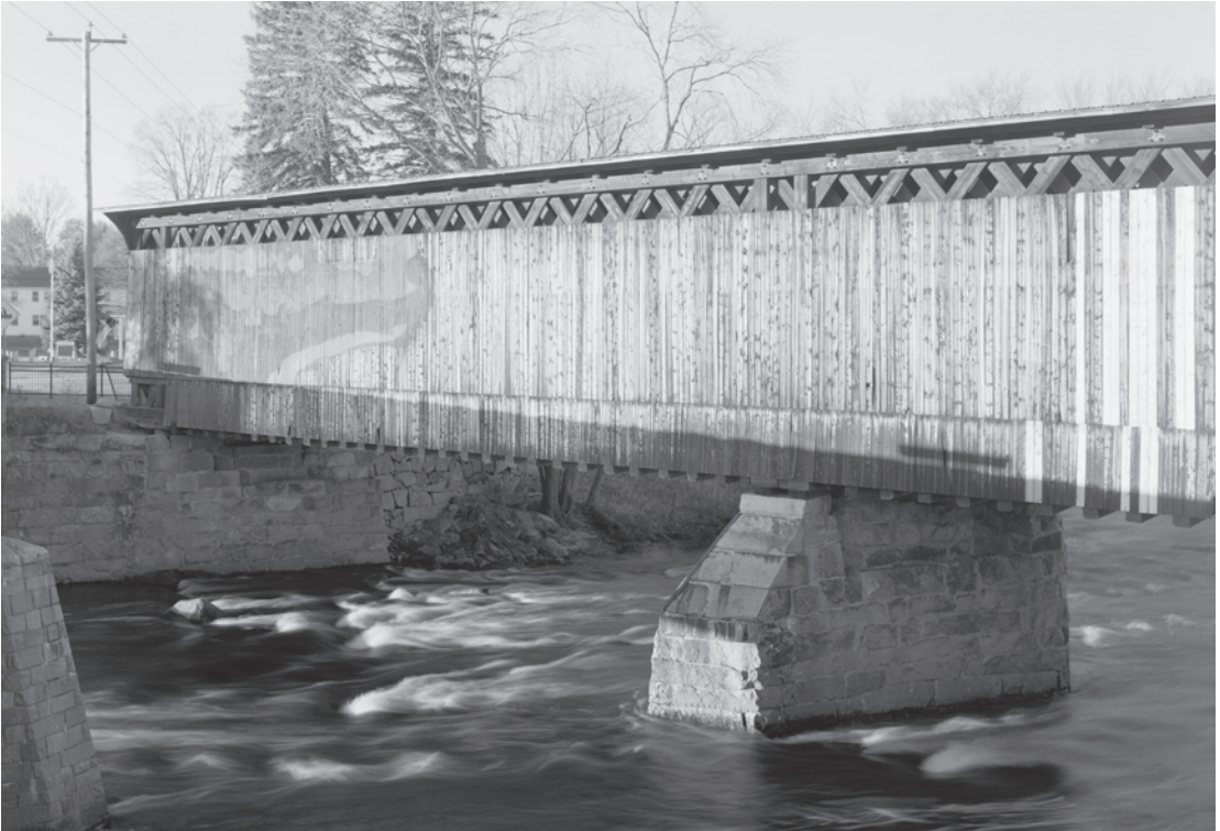
Figure 0.20 The two-span, double-web Town lattice Contoocook Railroad Bridge (1889), which spans the Contoocook River in Merrimack County, New Hampshire, was built under the supervision of J. P. Snow of the Boston and Maine Railroad. HAER NH-38-9, Jet Lowe, photographer, 2003.
