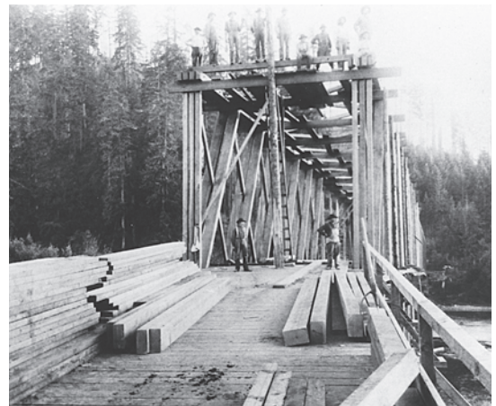
Figure 6.9 With its Howe trusses fully erected, the Hendricks Bridge was nearing completion when this photograph was taken in 1907. Courtesy of Bill Cockrell Collection.
