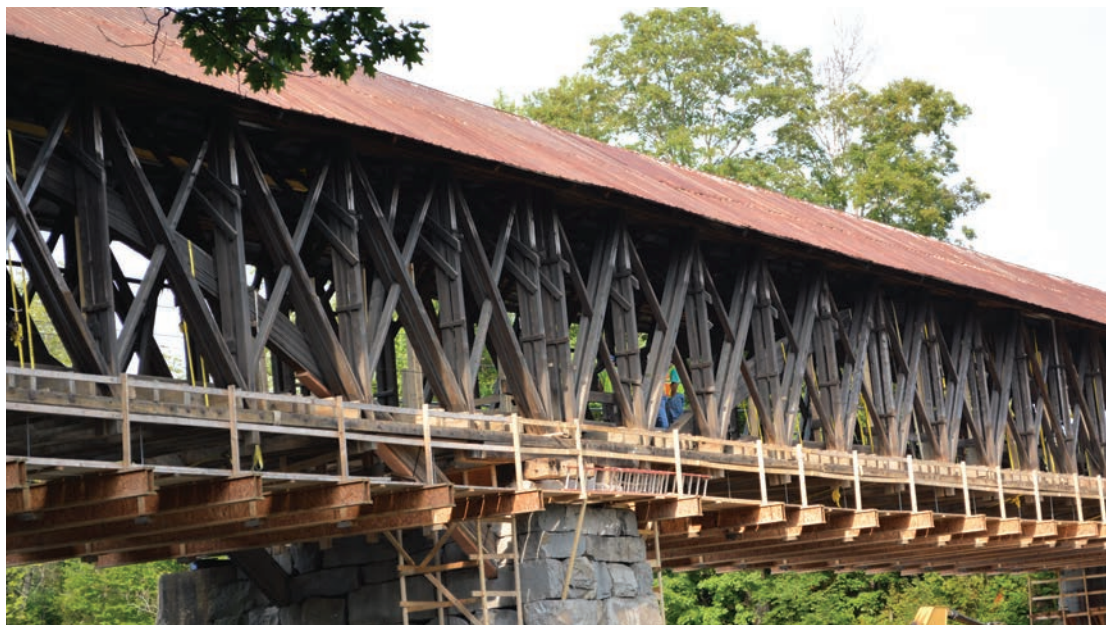
Figure 2.4 The rehabilitation of the Long truss on the Blair Bridge (1869) in Grafton, New Hampshire, required the use of staging, a technique discussed in the forthcoming “Guidebook for Restoring Structural Integrity of Covered Bridge Members.” Ron Anthony of Anthony & Associates, Inc., photographer, 2012.
