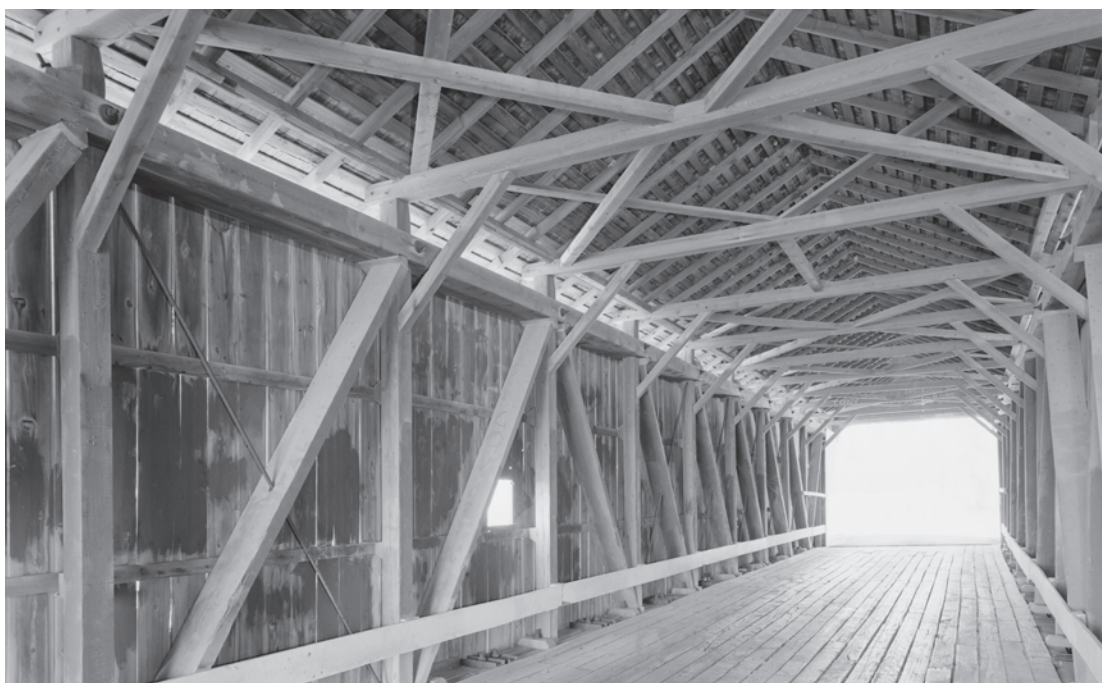
Figure 0.41 Harshman Bridge (1894) is one of seven surviving Childs trusses built by Everett Sherman in Preble County, Ohio, in the 1880s and 1890s. Horace Childs, a nephew and agent of Stephen Long, patented the design in 1846. HAER OH-126-10, Jet Lowe, photographer, 2004.
