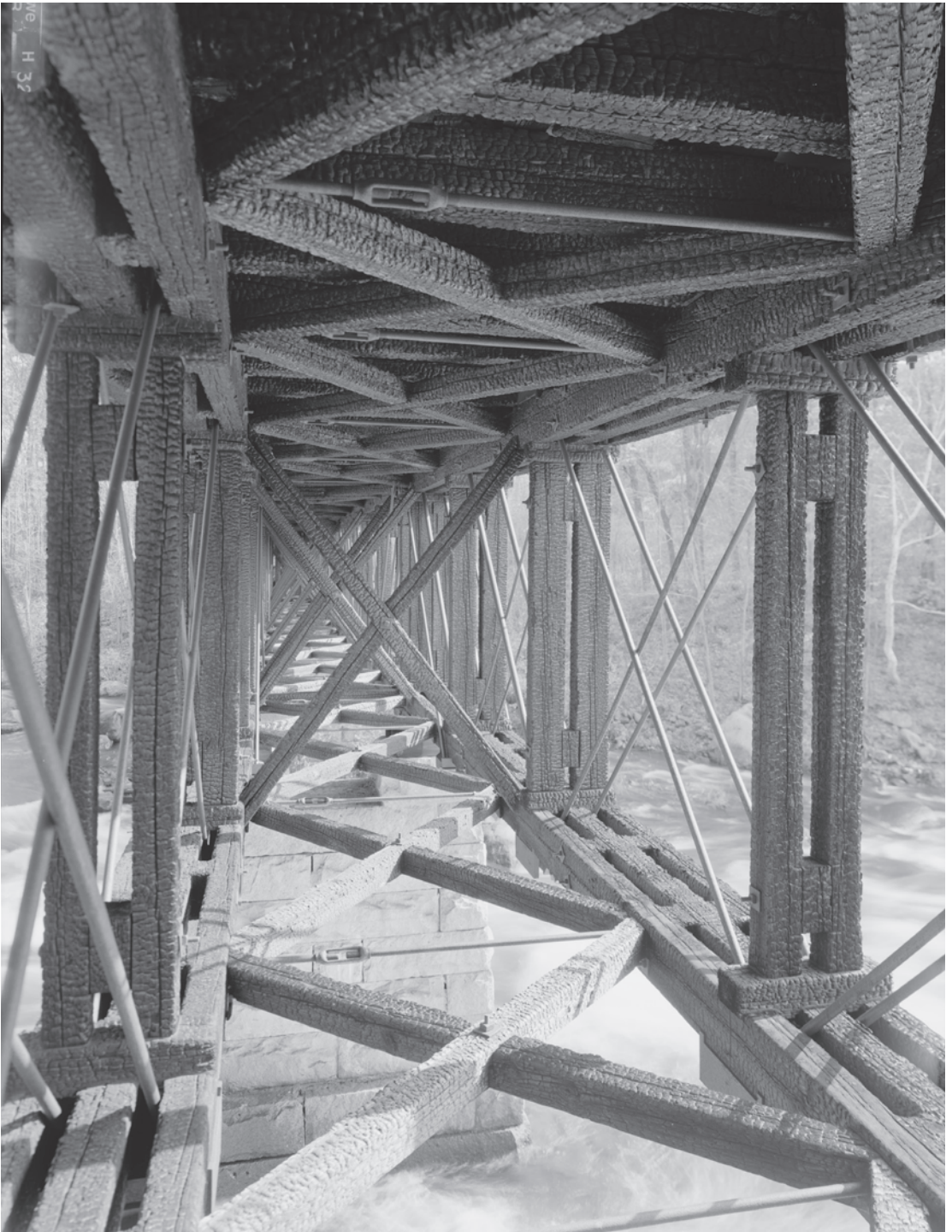
Figure 0.34 Although burned by arsonists in 1980, the Sulphite Railroad Bridge (1896) in Merrimack County, New Hampshire, survives as an example of a wood and iron Pratt deck truss. Patented by Thomas and Caleb Pratt in 1844, the Pratt truss reversed the configuration of the Howe truss, placing the short web members in compression and the long web members in tension, which reduced the danger of structural failure through buckling. Few timber Pratt-truss bridges were built, but the type was successfully adapted to iron and steel. By the late nineteenth century, the all-metal Pratt truss was the standard American truss for moderate railroad and highway spans. HAER NH-36-7, Jet Lowe, photographer, 2003.
