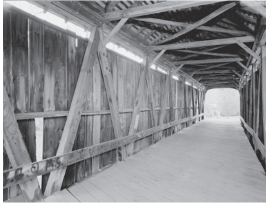
Figure 5.40 The 83-foot-long Salt Creek Bridge (1876) uses a single-web Smith truss with all inclined posts and braces in a single plane. HAER OH-127-9, Jet Lowe, photographer, 2004.
