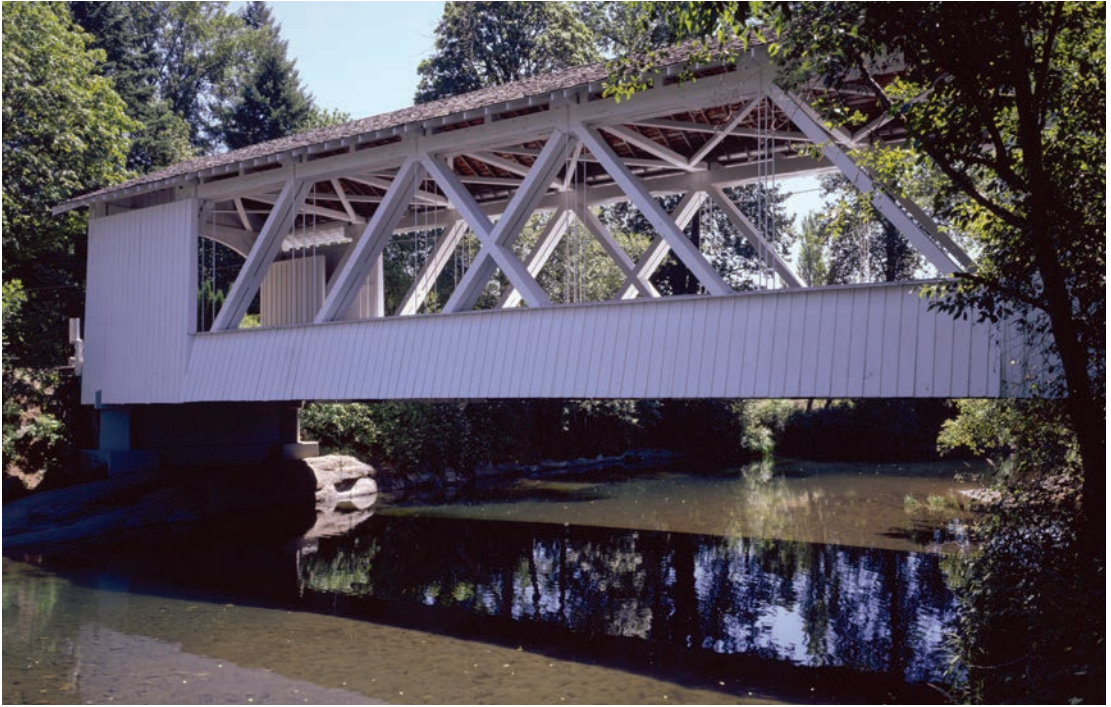
Figure 3.23 Built by the Linn County Engineering Department in 1941, Larwood Bridge is one of the best surviving examples of Oregon's standard-plan Howe trusses. HAER OR-124-13, Jet Lowe, photographer, 2004.
