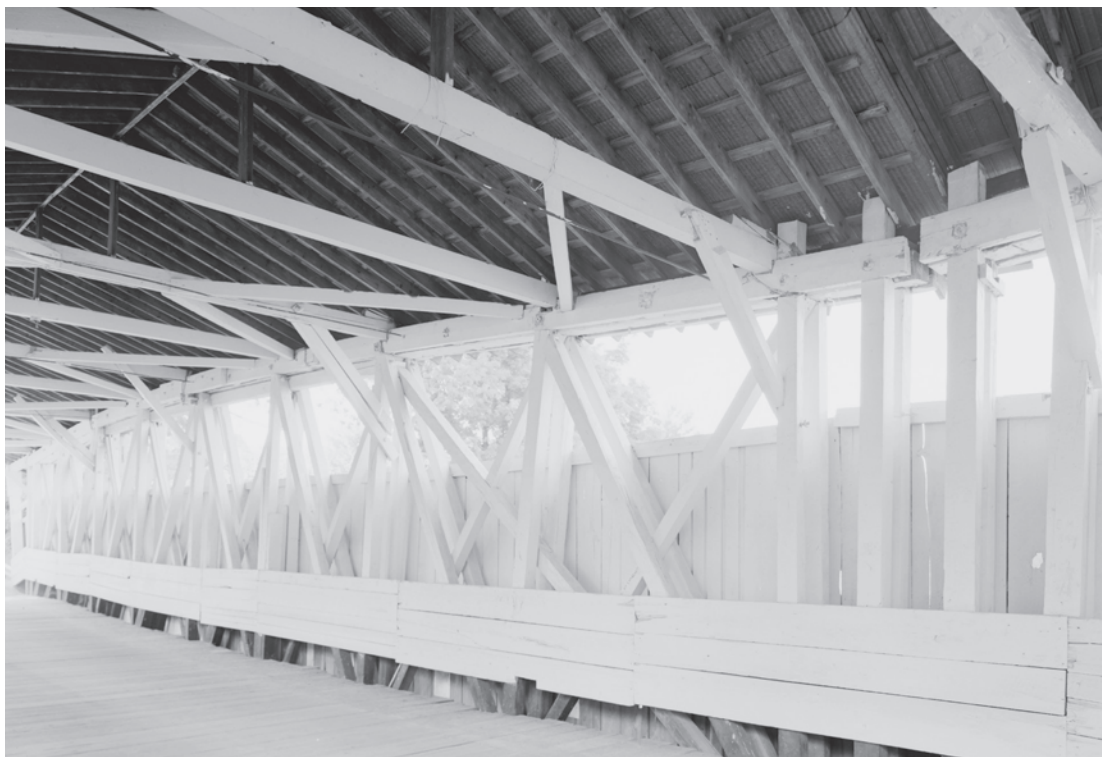
Figure 0.40 Patented by Daniel McCallum in 1851, the McCallum truss featured an arched upper chord and prestressed counterbraces and was used on North American railroads during the 1860s. The Powerscourt Bridge (1861), crossing the Chateaugay River in Huntingdon County, Quebec, is the only surviving example of this truss type. HAER NY-332-8, Jet Lowe, photographer, 2003.
