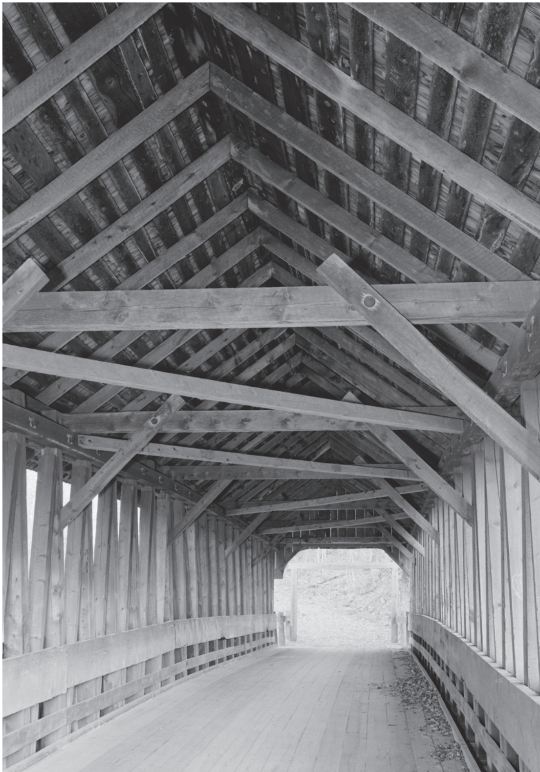
Figure 0.8 Kenyon (Blacksmith Shop) Bridge, a 96-foot-long multiple-kingpost truss in Sullivan County, New Hampshire, was constructed by James Tasker in 1882. HAER NH-40-4, Jet Lowe, photographer, 2003.
