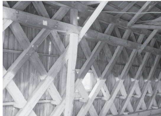
Figure 5.17 A detail of the squared-timber lattice truss on Bela Fletcher and James Tasker’s Cornish-Windsor Bridge (1866). The 6 x 8-inch timbers were connected at each joint by a notch and a single bolt instead of a pair of tree-nails. HAER NH-8-10, Jet Lowe, photographer, 1984.
