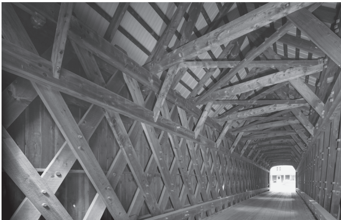
Figure 0.22 The interior view of Milton and Arnold Graton's Hall Bridge (1982) in Windham County, Vermont, showcases the twentieth-century craftsmen's knowledge of traditional timber framing and detailing in constructing a modern authentic covered bridge. HAER VT-40-11, Jet Lowe, photographer, 2009.
