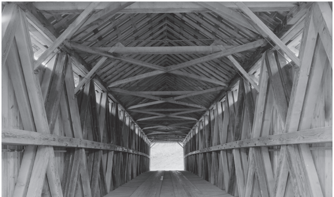
Figure 0.45 The Bennett's Mill Bridge (1875) in Greenup County, Kentucky, was the sole surviving historic Wheeler truss until it was rebuilt in 2004. Isaac Wheeler's truss design, featuring paired tension members, double-offset compression members, and an intermediate chord, was briefly popular in the Sciotoville, Ohio, area from 1870 to 1875. HAER KY-49-9, Jet Lowe, photographer, 2004.
