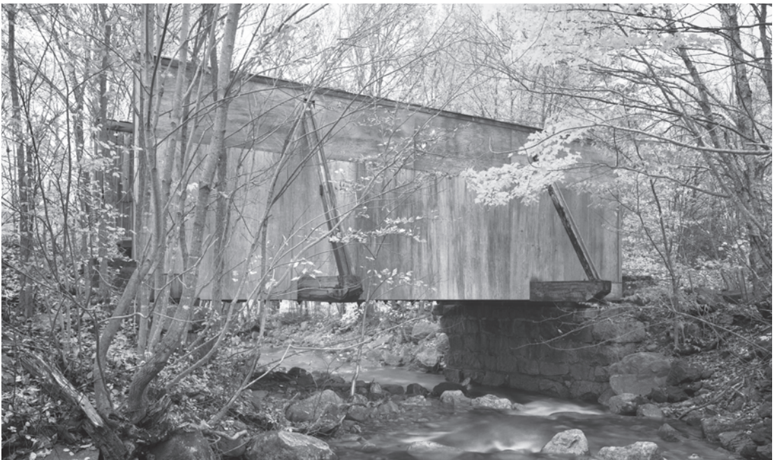
Figure 0.31 The 36-foot-long Snyder Brook Bridge (1918) in Coos County, New Hampshire, is a rare surviving Howe boxed pony truss (with supplemental outriggers), a once common bridge type built for short spans by the Boston and Maine Railroad. HAER NH-49-4, Jet Lowe, photographer, 2009.
