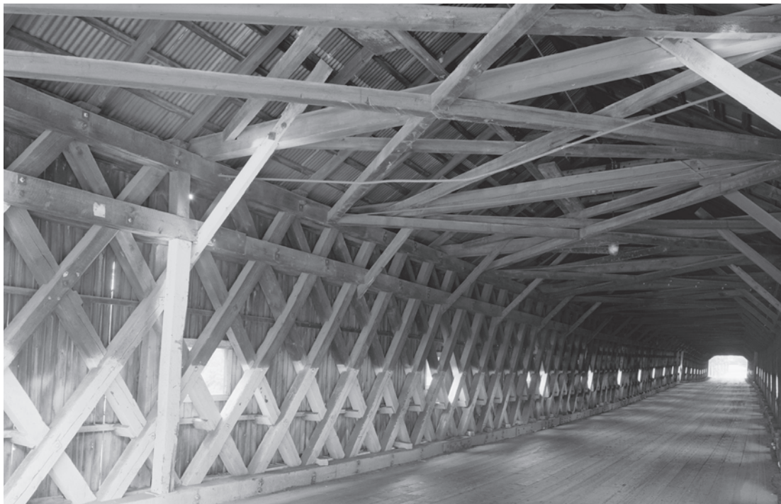
Figure 0.18 The Cornish-Windsor Bridge (1866) across the Connecticut River between Sullivan County, New Hampshire, and Windsor County, Vermont, is a notched Town lattice truss built by James Tasker and Bela Fletcher. With two spans of over 200 feet each, it is one of the longest historic covered bridges in the country. HAER NH-8-10, Jet Lowe, photographer, 1984.
