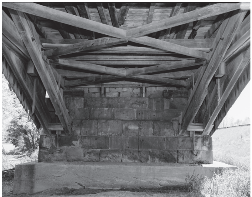
Figure 6.11 A view underneath West Union Bridge (1876) in Parke County, Indiana, shows how J. J. Daniels played his arches around the bottom chords of the trusses. HAER IN-105-9, James Rosenthal, photographer, 2004.
