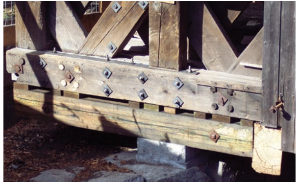
Figure 7.10 The replacement bed timbers installed on Contoocook used a bolted coupling splice inspired by a technique developed for similar structures by Snow and Fletcher in the 1930s. Note the granite pedestal supporting the corbel. Will Truax, photographer, 2007.
