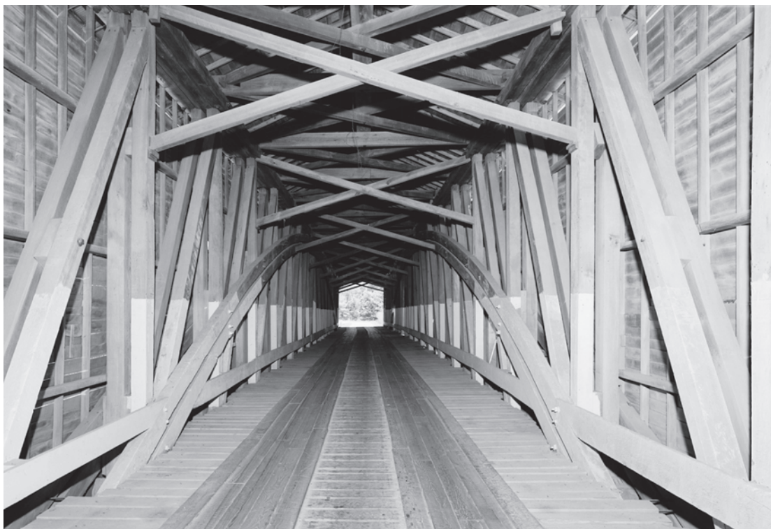
Figure 0.12 Built by Indiana master builder J. J. Daniels, Jackson Bridge (1861) in Parke County, Indiana, is a Burr-arch truss with paired diagonals, posts, and arches. With a span of 207 feet, the Jackson Bridge is the nation's longest single-span wood truss that still carries vehicular traffic. HAER IN-48-7, James Rosenthal, photographer, 2004.
