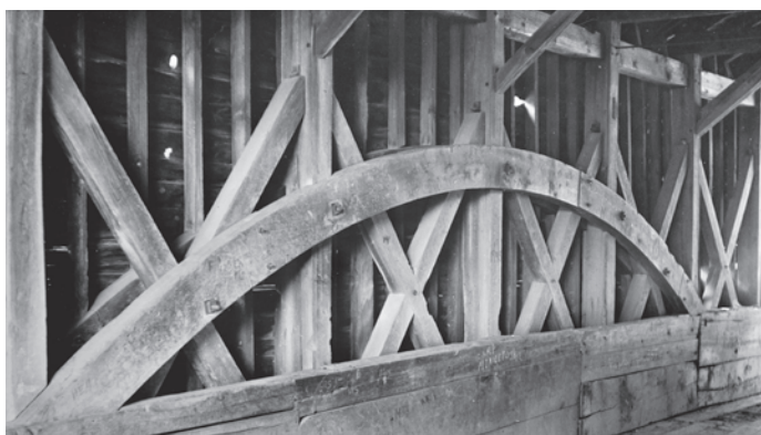
Figure 3.2 A testament to the value of covering timber bridges, Hyde Hall Bridge (1825) in Otsego County, New York, is believed to be the oldest extant covered bridge in the nation. It is one of several covered bridges in the United States that are nearing the two-century mark. HABS NY-263-2, unknown photographer, ca. 1958.
