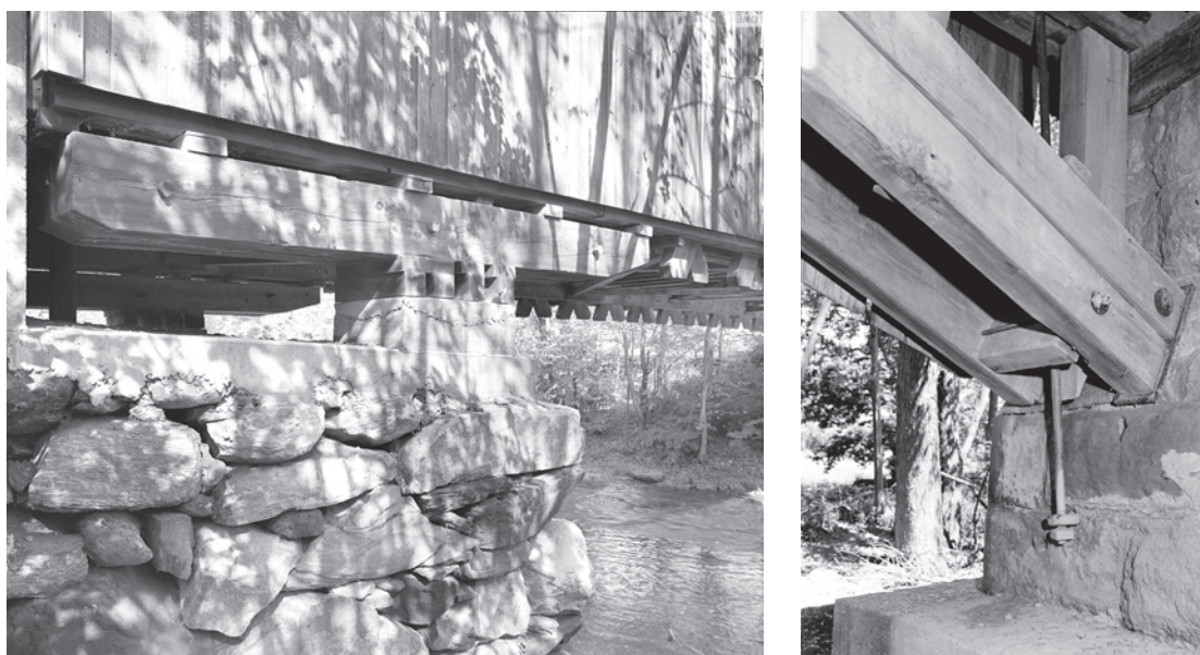
Figure 4.28 Examples of bolster beams and skewbacks. Left: 4.28a) Bolster beam detail on Hall Bridge, Windham County, Vermont, installed by Graton Associates in 1982. HAER VT-40-7, Jet Lowe, photographer, 2009. Right: 4.28b) Cast-iron skewback and rod tying the Burr arch into the limestone abutment of J. J. Daniels's West Union Bridge (1876), Parke County, Indiana. The arches bear on an inclined bearing surface called a skewback. HAER IN-105-11, James Rosenthal, photographer, 2004.
