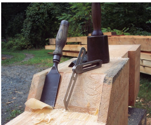
Figure 6.22 Top: 6.22a) The work done by Tim Andrews during the rehabilitation of Gilpin's Falls Covered Bridge in Cecil County, Maryland, carefully ensured the preservation of historic details. Above: 6.22b) Traditional timber-framing tools used in carving out the step in a vertical post on the Gilpin's Falls project include (left to right): a framing chisel, a corner chisel, a ca. 1930 line bevel, and a urethane carver's mallet. Will Truax, photographer, 2009
