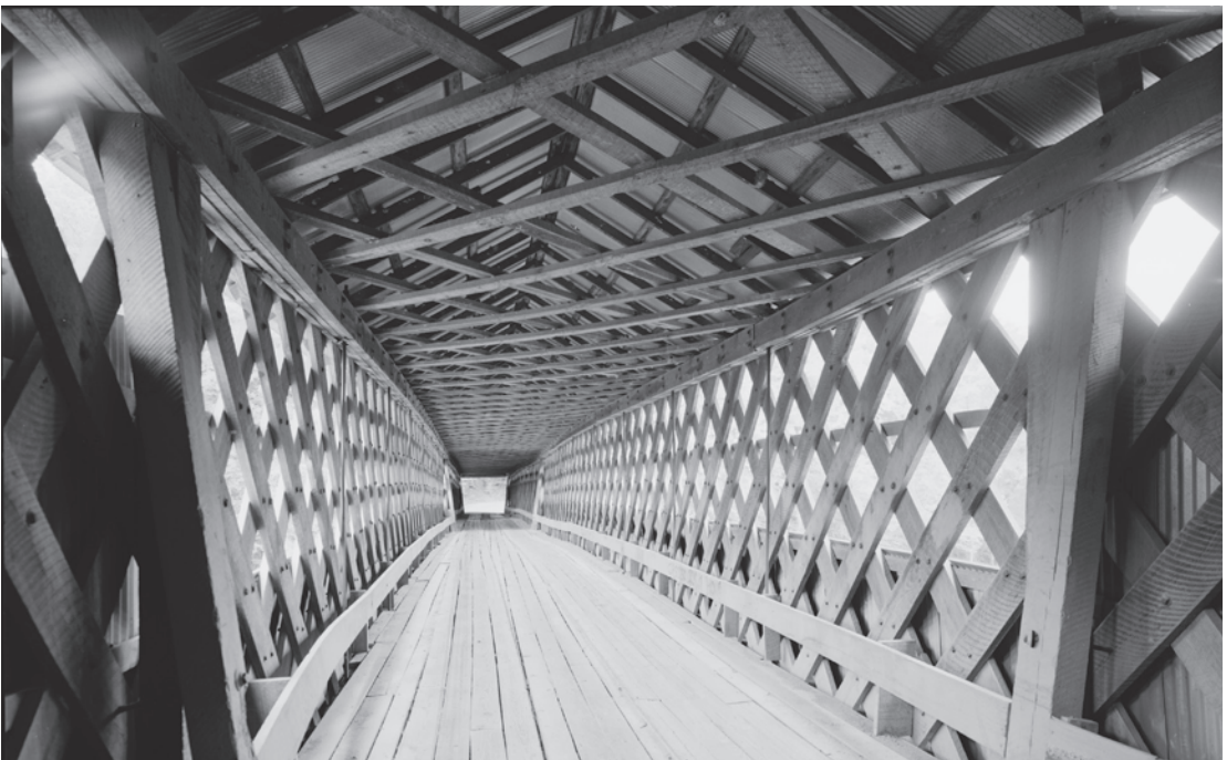
Figure 0.21 The 320-foot-long, three-span Swann Bridge (1933) features upper lateral bracing in a lattice web above its Town lattice trusses. One of three surviving wood bridges built in Blount County, Alabama, during the 1930s, it represents one of the last regions of covered bridge construction in the country. HAER AL-201-10, Jet Lowe, photographer, 2002.
