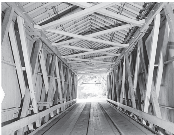
Figure 6.12 Powder Works Bridge (1872) in Santa Cruz County, California, is an excellent example of the early work of the Pacific Bridge Company and of the Smith type 4 triple-web truss. HAER CA-313-10, Jet Lowe, photographer, 2004.
