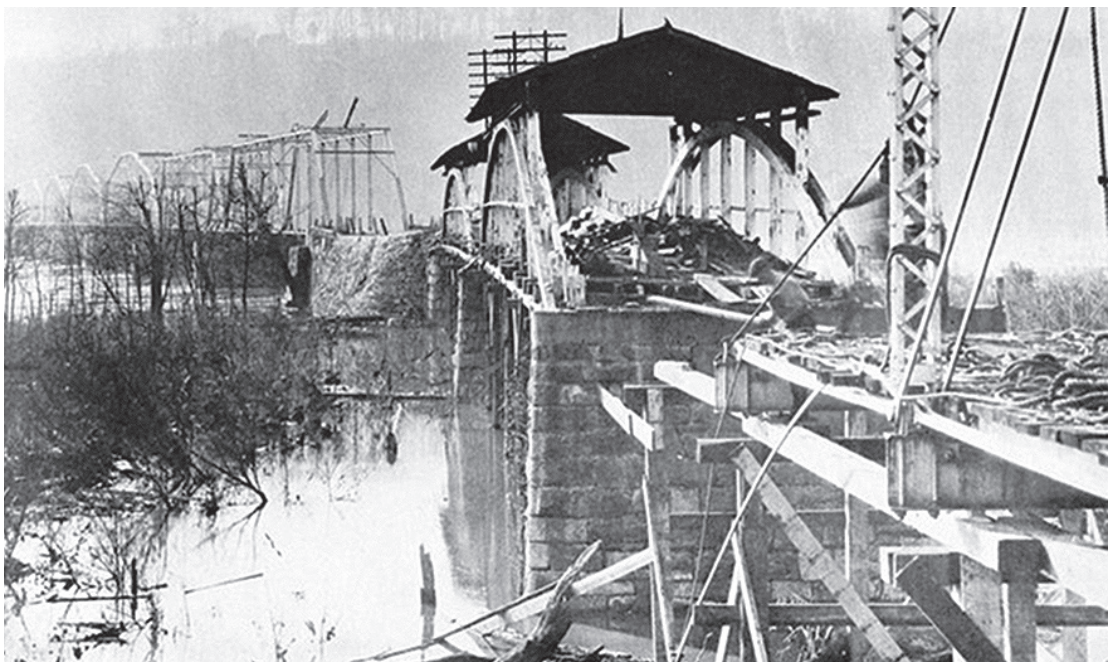
Figure 7.2 Built in 1859, the ten-span Conowingo Bridge crossed the Susquehanna River in Maryland. This photograph from ca. 1925 shows the new steel trusses being constructed in the background while the original wooden Burr-arch trusses are being dismantled. Courtesy of Richard Sanders Allen Collection, National Society for the Preservation of Covered Bridges.
