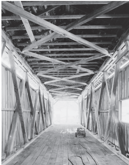
Figure 5.42 Cataract Bridge (1876) is a 140-foot Smith "double-truss" (Wilson type 3). The truss, the portal bracing, and the lateral bracing between the upper chords were all patented by Robert Smith. Note how both tension and compression diagonals are notched into the chords at midspan. HAER IN-104-6, James Rosenthal, photographer, 2004.
