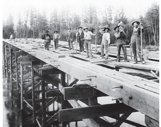
Figure 6.8 Construction of the Hendricks Bridge in 1907 began by laying out the bottom chords on the falsework. Courtesy of Bill Cockrell Collection.
