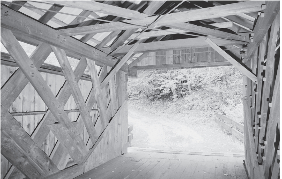
Figure 0.15 The Beaverkill Bridge (1865) is distinctive for its fan-like radiating planks at the ends of the lattice trusses. Carpenter John Davidson built this regional variation of the Town lattice in Sullivan County, New York, where two other examples survive from the 1860s. HAER NY-329-5, Jet Lowe, photographer, 2003.
