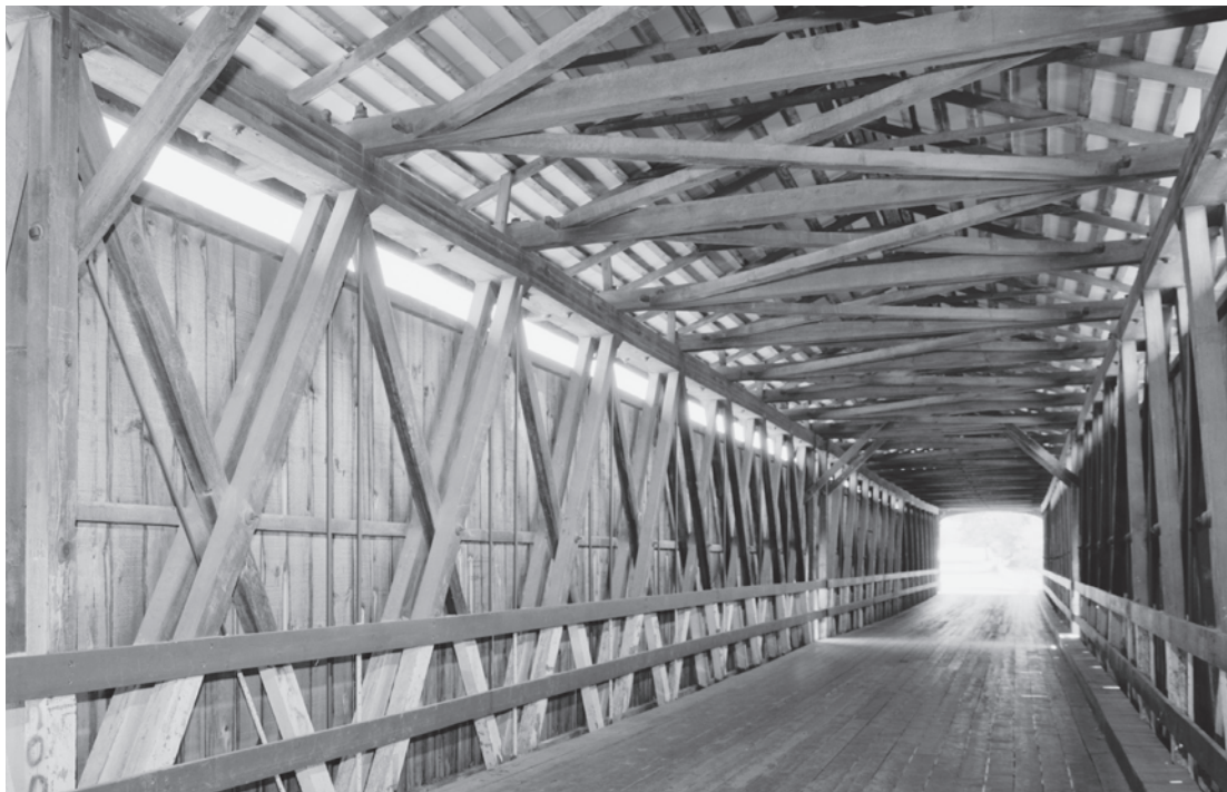
Figure 0.26 Knight's Ferry Bridge (1863) in Stanislaus County, California, is a 379-foot-long, four-span Howe truss built as a major crossing on the Stockton to Sonora Road. Its high integrity as one of the best remaining examples of a wood and iron Howe truss contributed to its designation as a National Historic Landmark in 2012. HAER CA-314-8, Jet Lowe, photographer, 2004.
