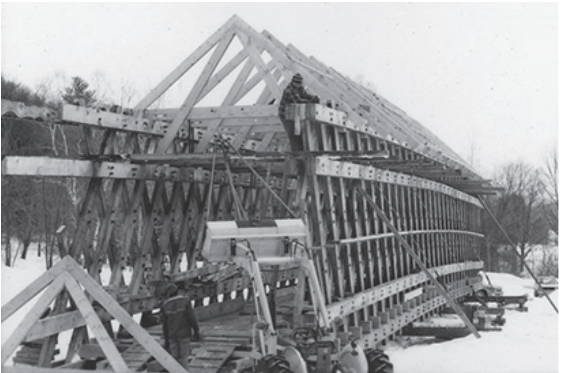
Figure 6.6 Arnold Graton erected a replacement for the Hall Bridge across Saxtons River in Windham County, Vermont, in 1982. Using traditional techniques, Graton Associates developed rough specifications from the original 1867 bridge and then framed it in a nearby field using traditional joinery and treenails. A team of oxen hauled the completed structure out across the river, and the bridge opened to traffic on September 6, 1982. Jack Peters, photographer, 1982. (See "Hall Bridge," HAER VT-40 for additional information.)
