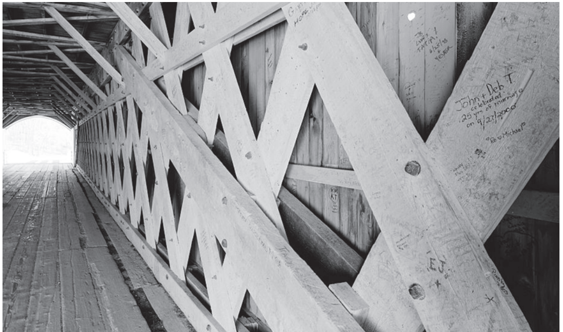
Figure 3.22 Roseman Bridge (1883) is one of nineteen covered bridges built in Madison County, Iowa, in the nineteenth century and one of only five that survive. Prominently featured in the 1995 movie adaptation of Robert James Waller’s romantic novel, The Bridges of Madison County , the bridge has since become a popular wedding venue. HAER IA-95-5, Jet Lowe, photographer, 2004.
