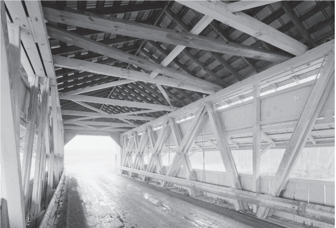
Figure 0.42 Pottersburg Bridge (1872) is one of five surviving Partridge trusses. A prolific builder based in Union County, Ohio, Reuben Partridge patented a truss design similar to the Smith truss. HAER OH-125-9, Jet Lowe, photographer, 2003.
