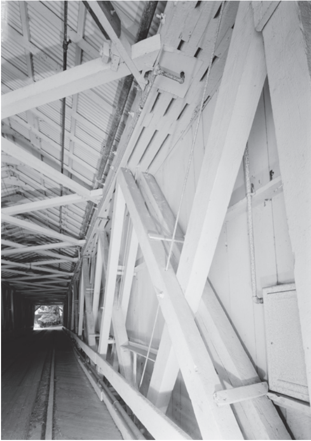
Figure 0.36 The Powder Works Bridge (1872) in Santa Cruz County, California, is a triple-web Smith truss built by William Gorrill's Pacific Bridge Company, which introduced the Smith patent to the northwestern part of the country and built several wooden bridges in California and Oregon in the 1870s. HAER CA-313-9, Jet Lowe, photographer, 2004.
