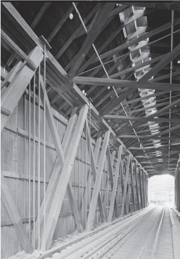
Figure 0.30 Clark's Railroad Bridge (1904) in Grafton County, New Hampshire, which was originally located upstate in Coos County on an important link on the granite-hauling Barre Branch Railroad, features substantial Howe trusses. Today it remains active on the steam excursion line at Clark's Trading Post. HAER NH-39-8, Jet Lowe, photographer, 2003.
