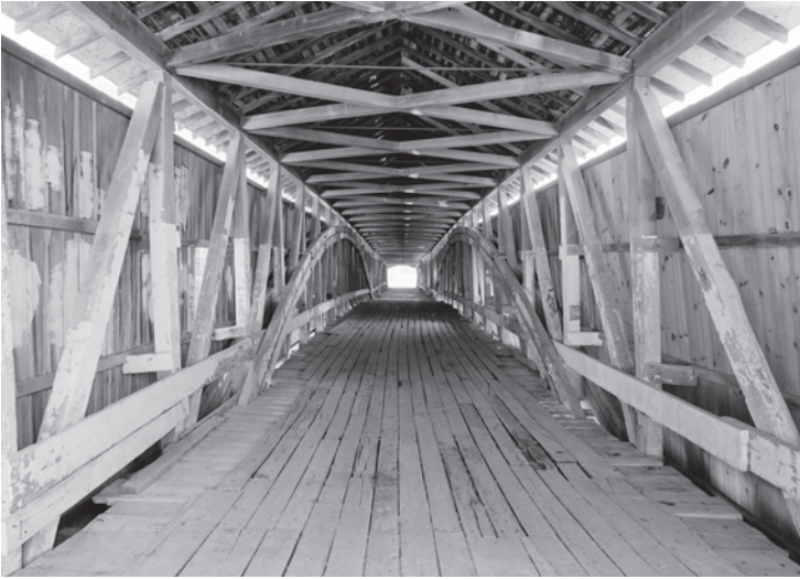
Figure 4.21 To transfer horizontal or lateral wind forces to the abutments, designers conceptualized and designed horizontal trusses and two-dimensional, or plane , frames as shown here. The horizontal trusses are at the plane of the floor and at the plane defined by the two top chords. For pony-type bridges, it was not possible to carry wind load and stabilize the top chord through a horizontal truss, so outriggers were installed. Examples of bracing include Top Left: 4.21a) horizontal lateral bracing to resist wind on the West Union Bridge (1876), Parke County, Indiana, HAER IN-105-13, James Rosenthal, photographer, 2004; Middle: 4.21b) Portal frames to transfer loads taken by the top chord on the Flint Bridge (1874), Orange County, Vermont, HAER VT-29-5, Jet Lowe, photographer, 2003; Bottom L: 4.21c) outriggers to stabilize top chords on the Beaverkill Bridge (1865), Sullivan County, New York, HAER NY-329-10, Jet Lowe, photographer, 2003.
