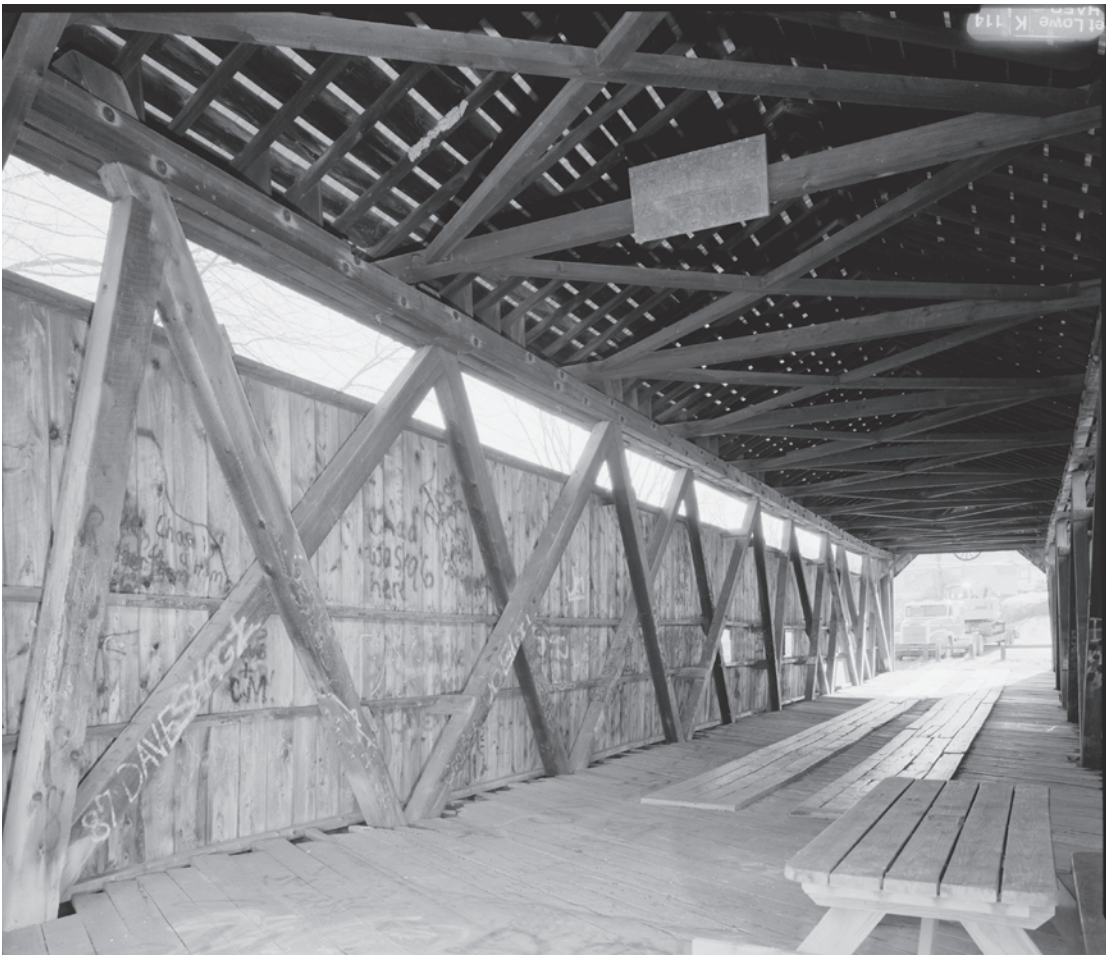
Figure 0.35 This end panel of Kidd's Mill Bridge (1868) in Mercer County, Pennsylvania, shows the extra, steeply inclined compression brace common to trusses patented by Robert W. Smith, who successfully introduced industrial processes into covered bridge construction through his two Ohio companies. HAER PA-622-5, Jet Lowe, photographer, 2006.
