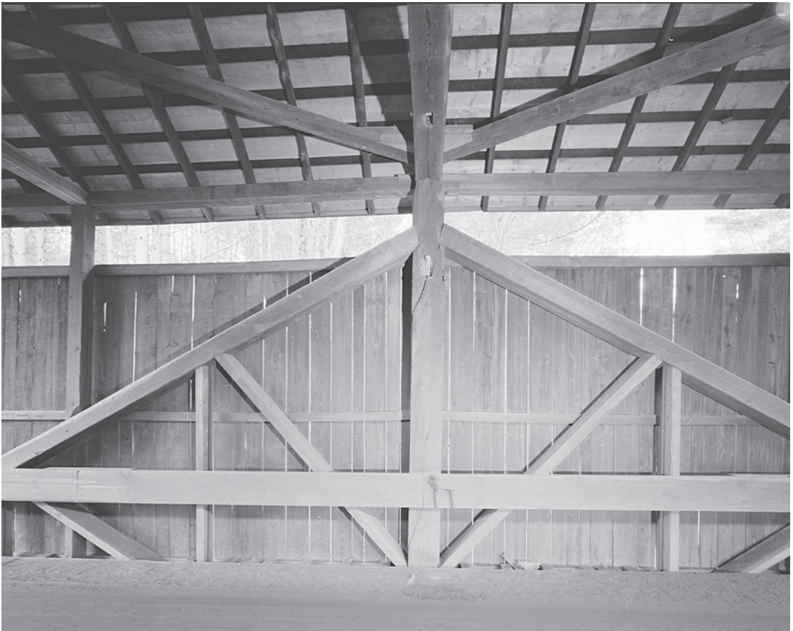
Figure 0.3 Pine Brook Bridge (1872) in Washington County, Vermont, is a 48-foot-long kingpost-truss bridge, rehabilitated by Milton Graton in 1977. The kingpost truss, a simple truss design commonly used for roof framing for centuries, was a common truss type sufficient for modest spans. There are only about twenty historic examples of kingpost-truss covered bridges remaining in the United States. HAER VT-37-8, Jet Lowe, photographer, 2006.
