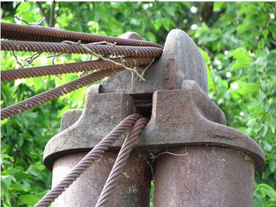
TX_Erath County_Bluff Dale Bridge_0013.tif Castings on top of northeast tower, looking north northwest
