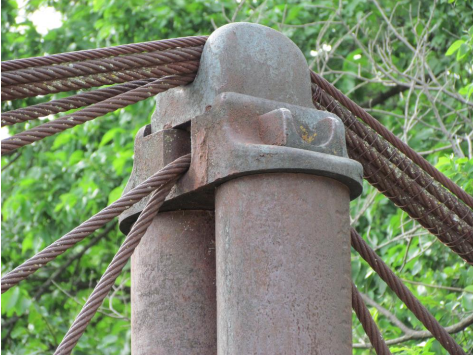
TX_Erath County_Bluff Dale Bridge_0012.tif Castings on top of northwest tower, looking northwest
