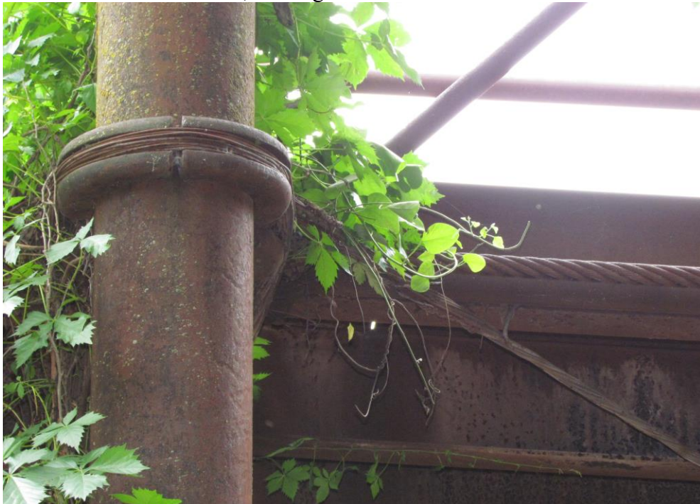
TX_Erath County_Bluff Dale Bridge_0017.tif Patented tower connection, looking east
