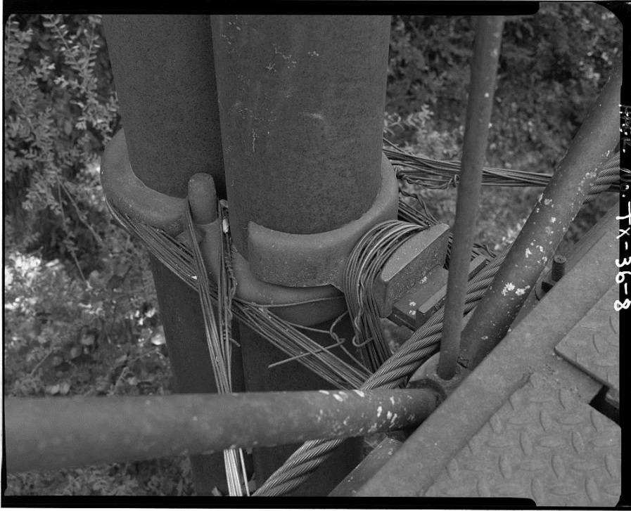
Figure 15: HAER TX-36 Photograph by Joseph E. B. Elliot (1996). Connection details at southeast column.
