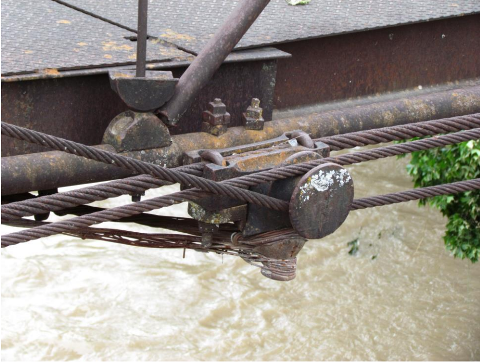
TX_Erath County_Bluff Dale Bridge_0018.tif Patented deck beam castings and cable details, looking northwest
