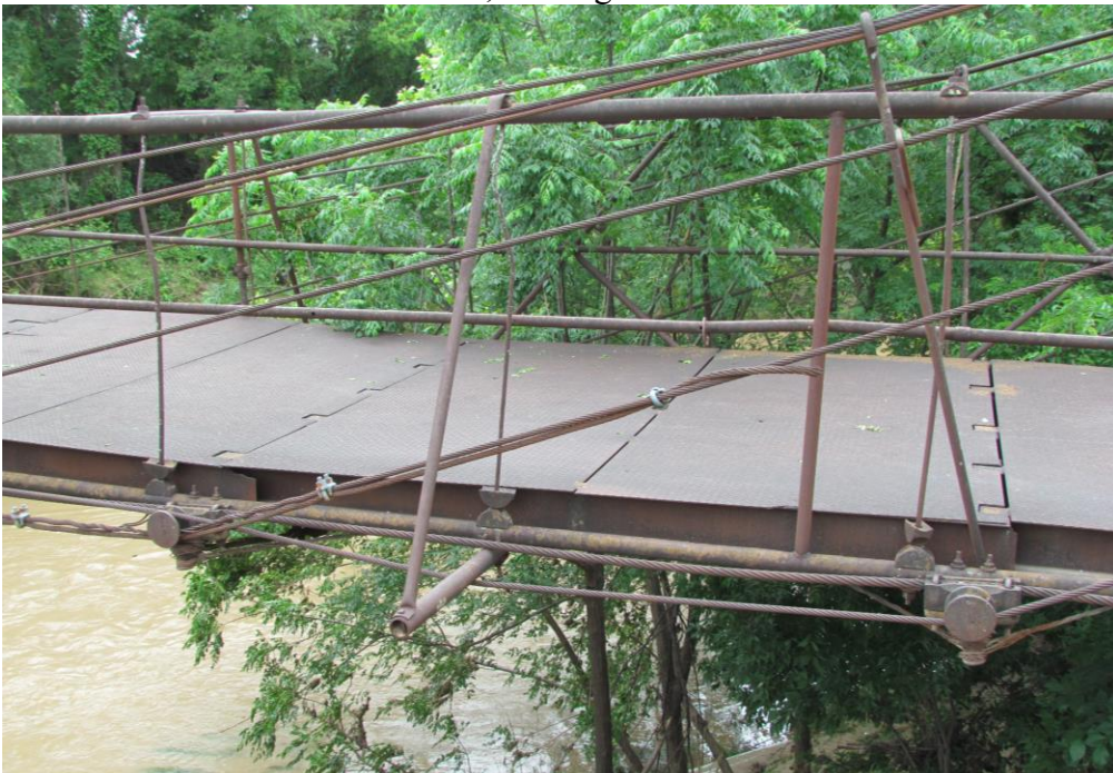
TX_Erath County_Bluff Dale Bridge_0011.tif Deck connections and truss losses, looking west southwest
