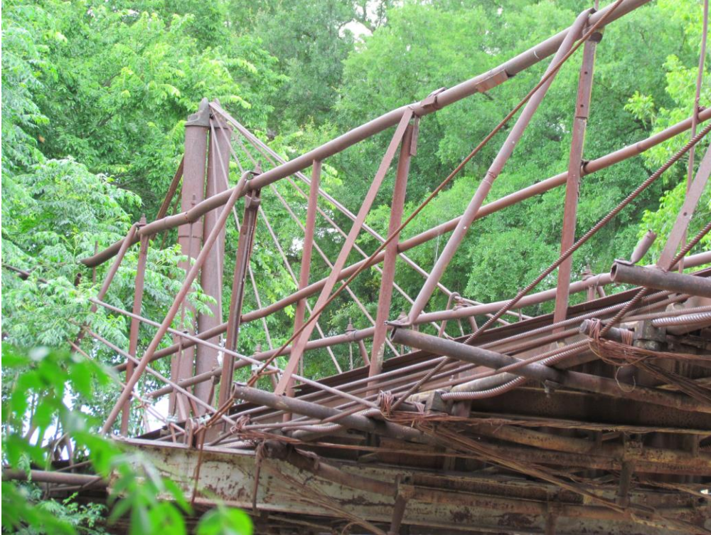
TX_Erath County_Bluff Dale Bridge_0010.tif Oblique view of deck and northeast tower, looking northeast
