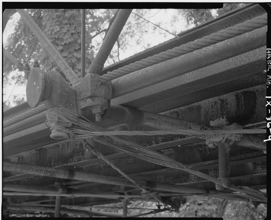
Figure 16: HAER TX-36 Photograph by Joseph E. B. Elliot (1996). Detail, cable attachment point, from below.
