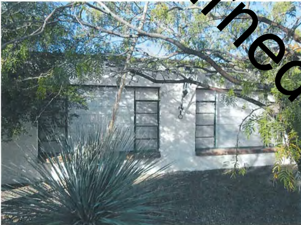
Photograph #8 Garage conversion (1964) detail of large casement windows (inspired by north living room window) in original garage door openings, camera facing southwest.
