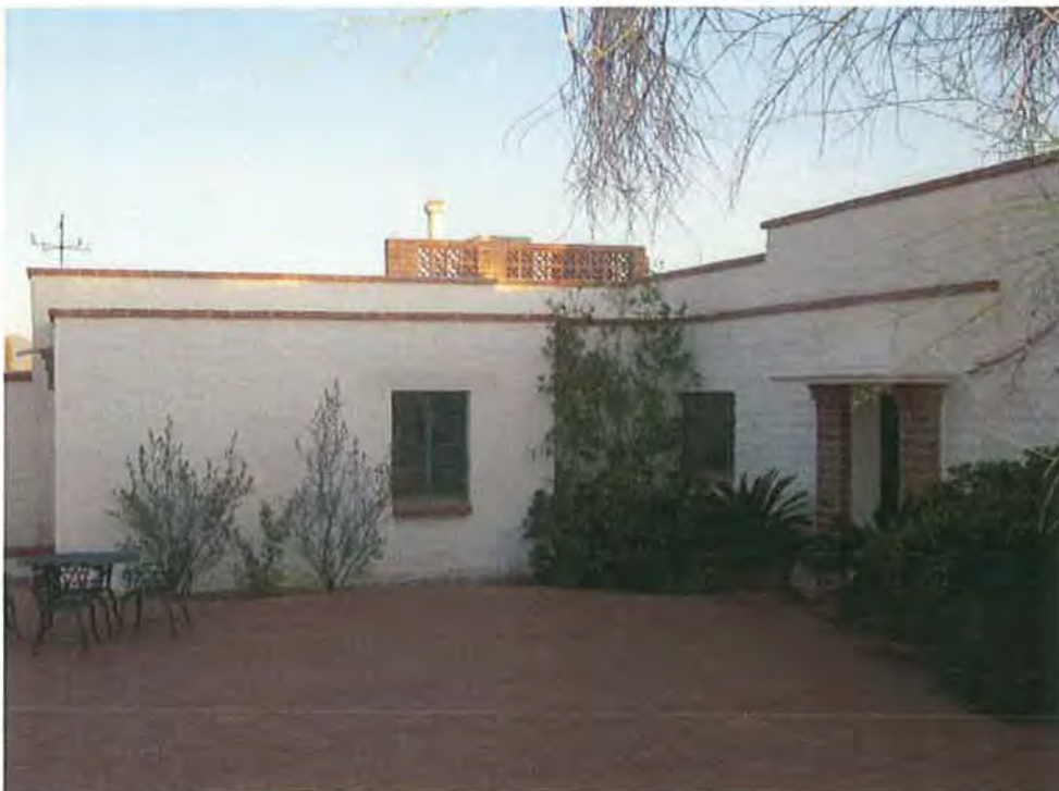
Photograph #10 View of Connector (1958); its modest square footage and lower profile comply with the Secretary of the Interior's Standards (NPS2002) note characteristic wrought iron weathervane atop bedroom wing, camera facing south.
