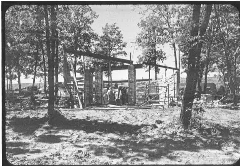
Summer, 1959, looking westerly at the stone walls and east side piers under construction. The workmen are standing on the lower level floor.
