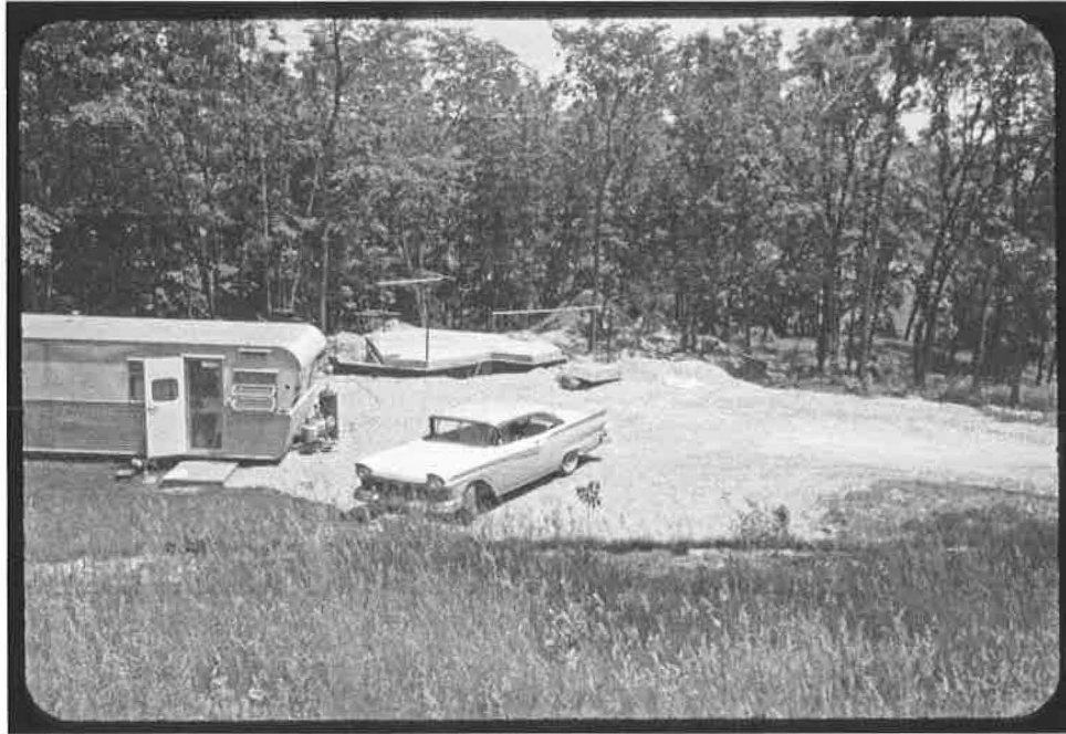
Summer, 1959, from the highway shoulder looking down at the entry level floor under construction. This precast concrete floor covers the block foundation.
