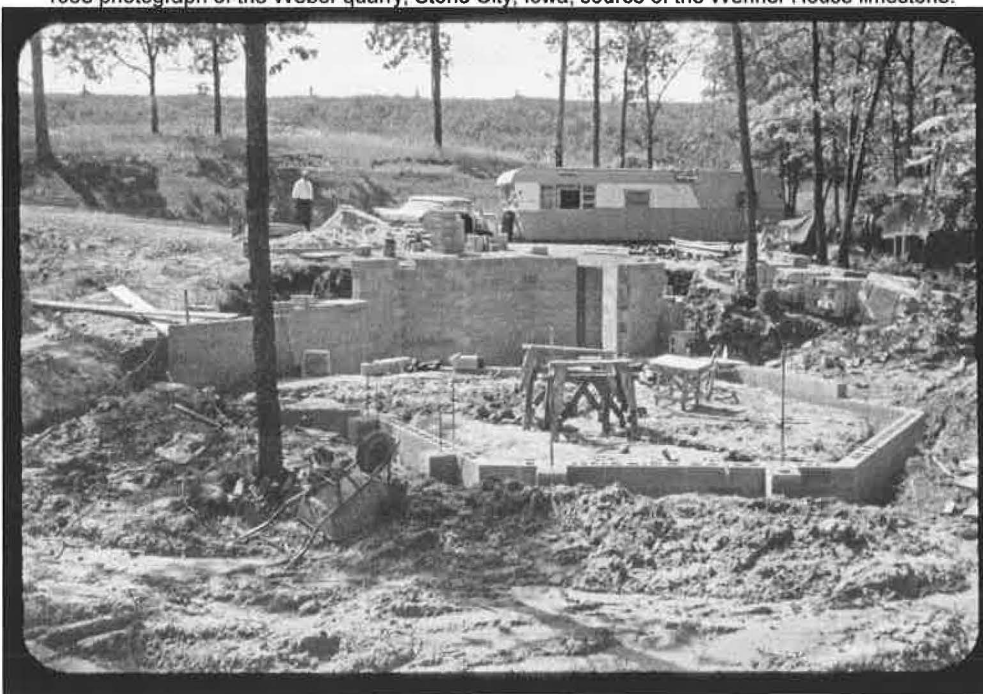
Summer, 1959 photo of the building site with concrete block foundation walls being laid up.
