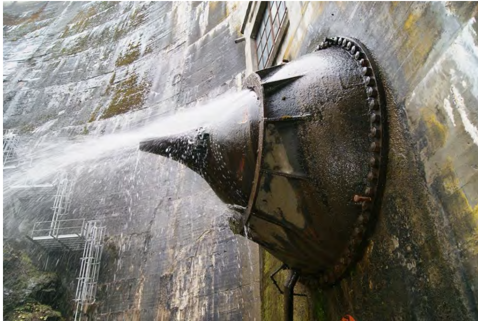
Photo 13. Needle valve detail on Cushman No. 1 valve house.
