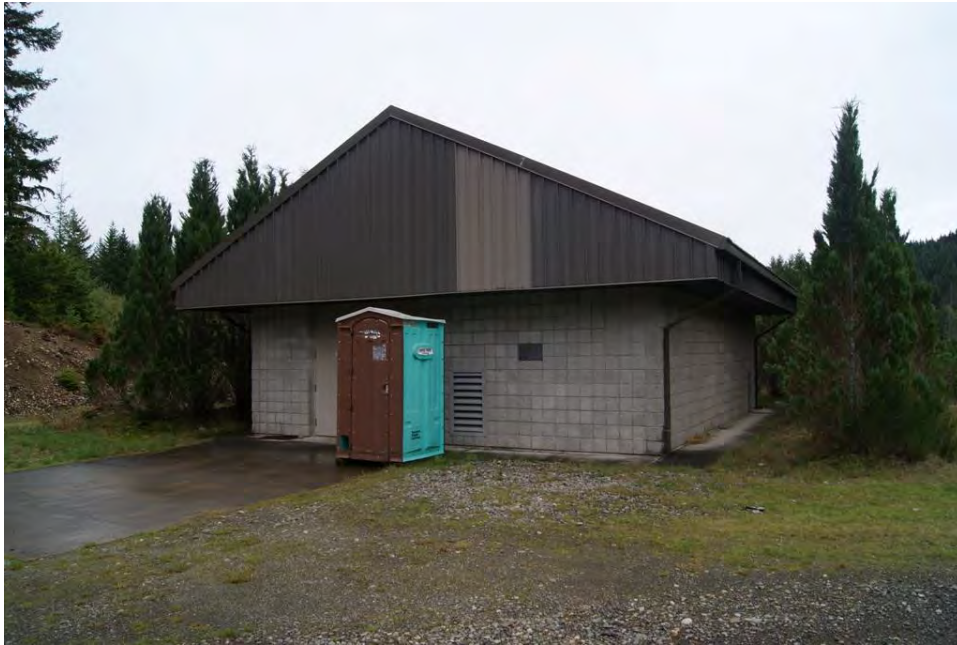
Photo 19. Spillway Control House, located west of the modern spillway at Cushman No. 1.
