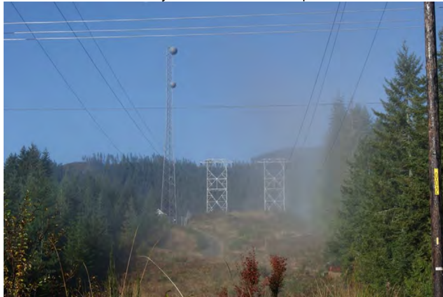
Photo 45. View of steel lattice towers located east of Cushman No. 1 along the Cushman transmission-line corridor.
