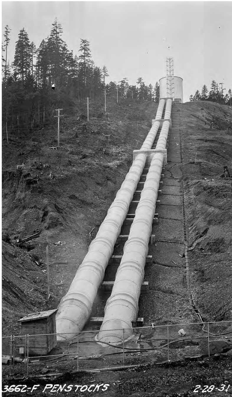
Figure 17. Cushman No. 2 penstocks, surge tank and vent pipes, February 28, 1931. Image courtesy of Tacoma Power.
