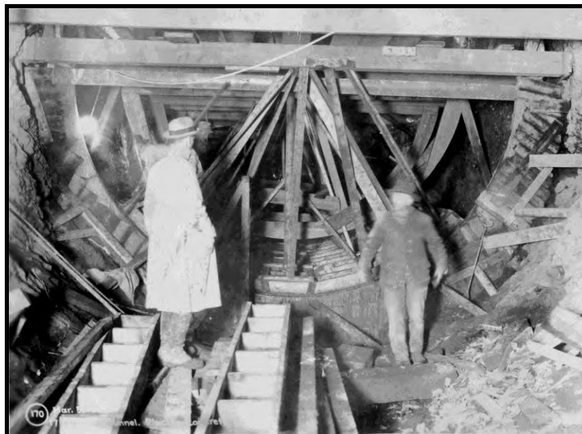
Figure 8. Cushman No. 1 power tunnel concrete forms, March 5, 1926. Image courtesy of Tacoma Power.
