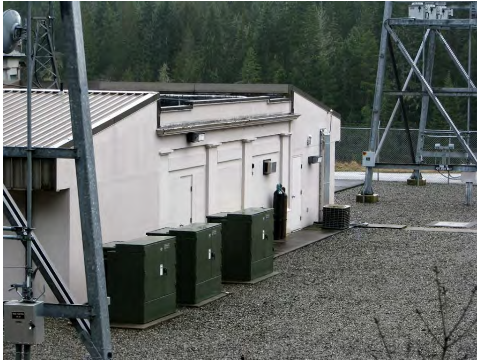
Photo 21. Close-up of Cushman No. 1 substation building north face, showing evidence of original building (center), with concrete parapet and engaged pilasters, surrounded by modern construction, viewing south.
