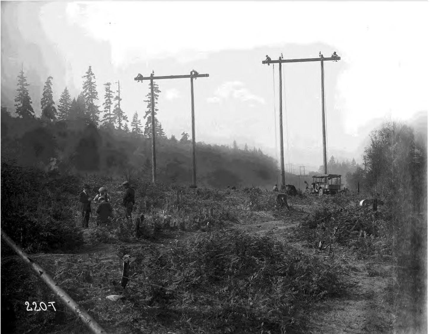
Figure 18. Construction of the Potlatch (Cushman) Transmission Line, ca. 1925. Image courtesy of Tacoma Power.
