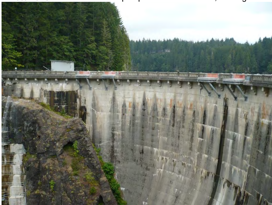
Photo 29. Cushman No. 2 dam, showing modern crane pads at parapet and spillway control house, viewing northeast.
