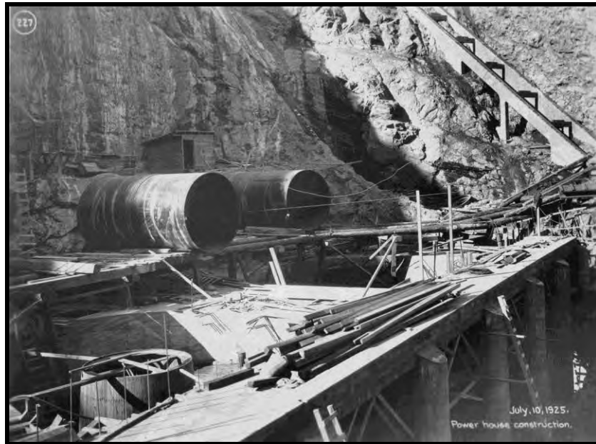
Figure 9. Penstocks at entry to Cushman No.1 powerhouse (powerhouse under construction), July 10, 1925. Image courtesy of Tacoma Power.
