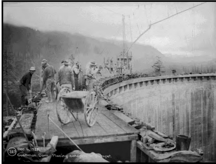
Figure 3. Construction of parapet at Cushman No. 1 dam, December 6, 1925. Image courtesy of Tacoma Power.
