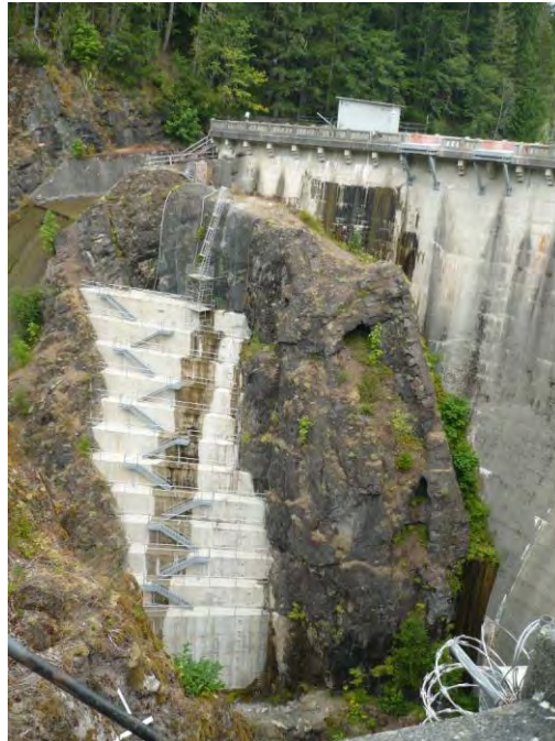
Photo 30. Cushman No. 2 dam, showing abutment infill, spillway, and spillway control house, viewing north.
