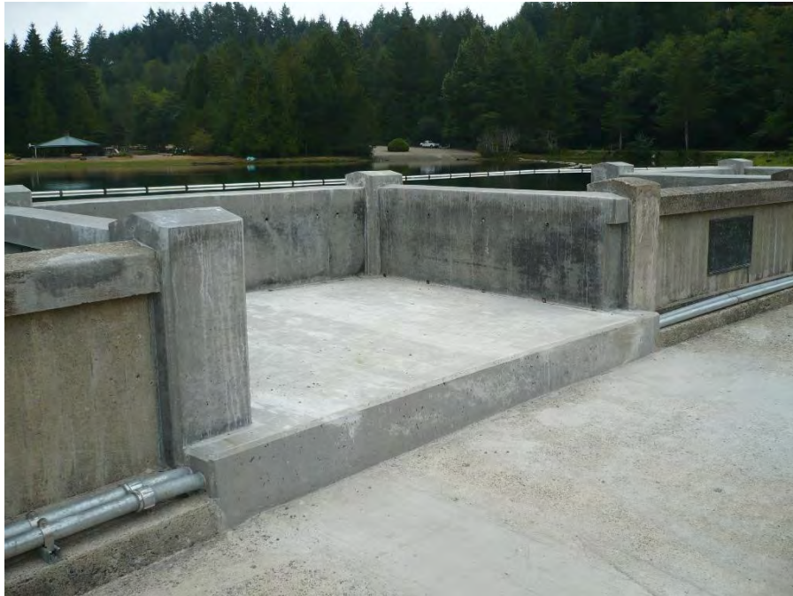
Photo 32. Detail of modern crane pads on Cushman No. 2 dam parapet, viewing east.
