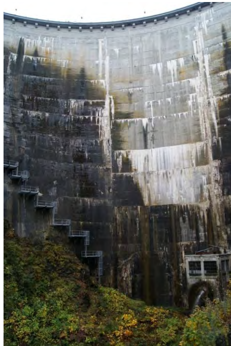
Photo 11. Cushman No. 1 dam, downstream face, showing valve house (right) and new stairs (left), viewing west.
