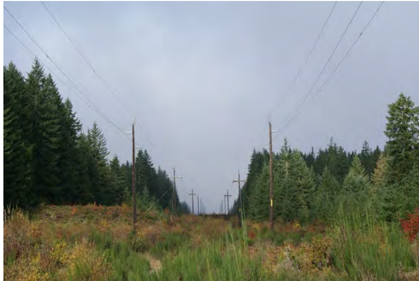
Photo 46. Typical view of the Cushman Nos. 1 and 2 transmission line corridor.
