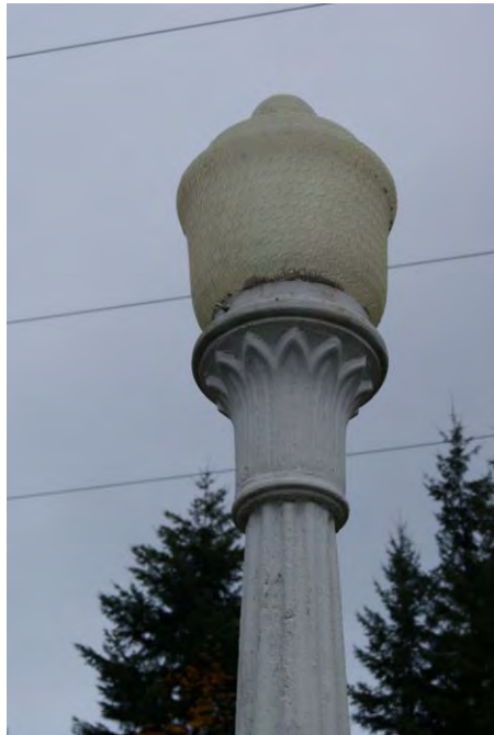
Photo 24. Detail of cast concrete lamp post (with modern plastic globe) at Cushman No. 1.
