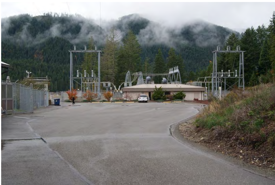
Photo 20. The substation and switchyard at Cushman No. 1, viewing west.
