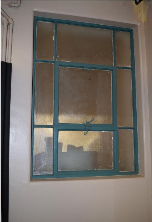
4 of 30: Ferry County Courthouse original steel-framed exterior window, W side of basement
