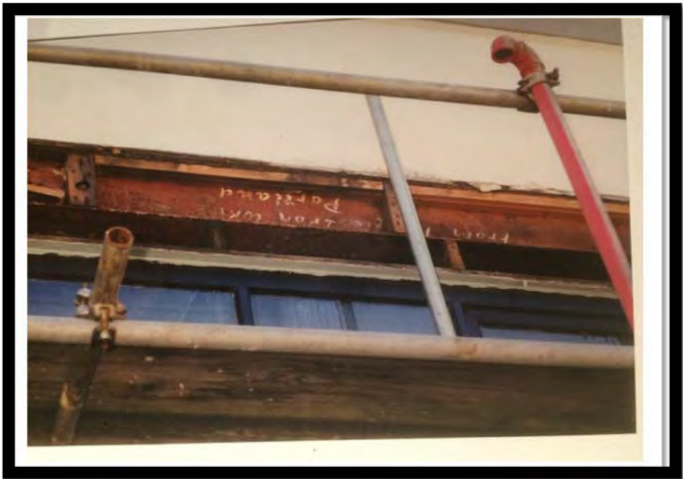
Figure 24: Uncovered during the 1997 renovation, on the north façade of the building, are the pairs of steel I-beams above transom windows. View is looking south.
