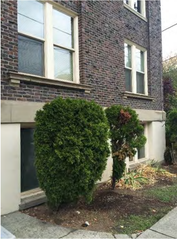
8 Detail view of the concrete, stone and masonry base and basement and first floor windows.
