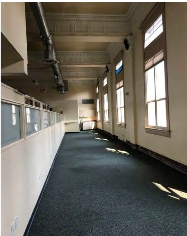
41. Left, looking east along the third-floor perimeter south wall and inserted office partitions.
