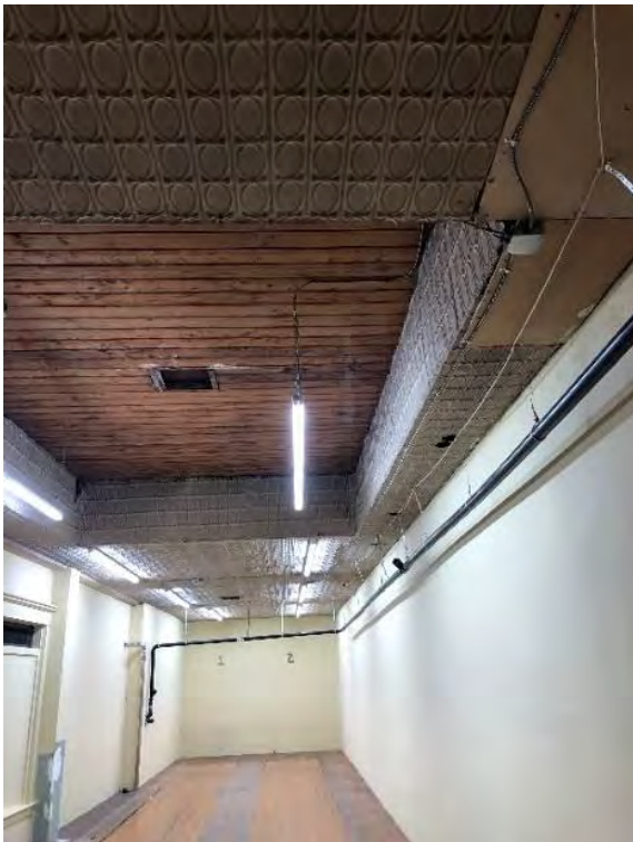
21. Below left, looking west in the former bowling in the basement. The unfinished ceiling was originally a skylight (RAG, June 2018).
