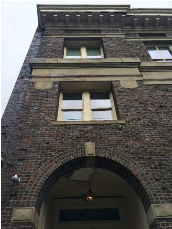
10. Detail view above of the club entry near the west end on the south facade.
