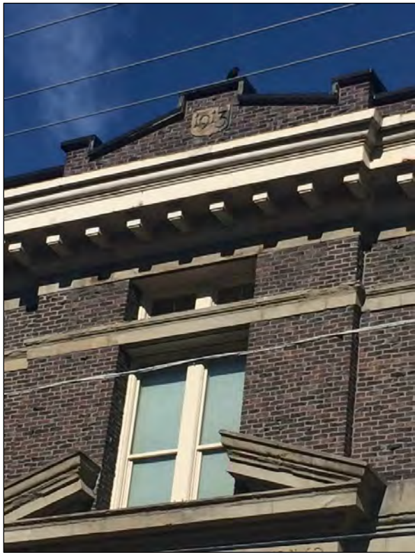
16. Above right, a detail view of the cornice and construction date above the current primary entry.
