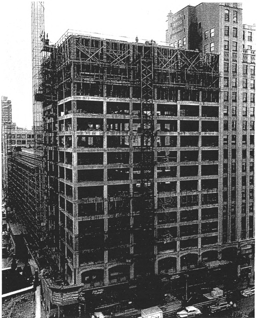
Historic Preservation Certification Application – Part I MEDICAL DENTAL BUILDING, 509 Olive Way, Seattle, King County, Washington 98101
