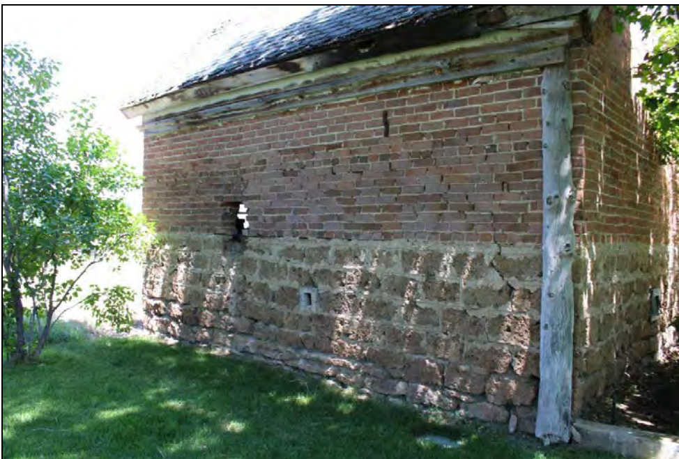
22 of 36. Outbuilding 1 (creamery/granary). Camera facing northeast. Note attached sections of wood on west side of building
