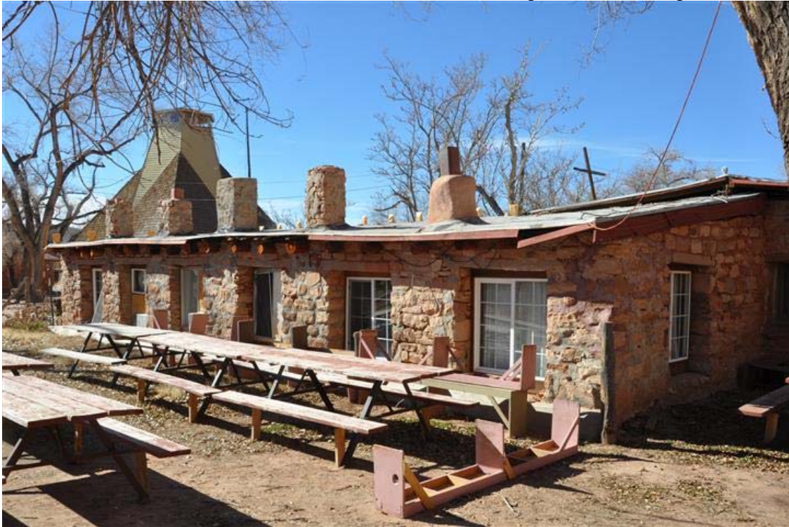
31 of 50. North and east elevation of mission house east wing. Camera facing southwest.
