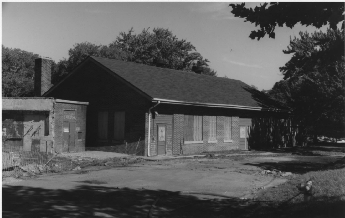
Marconi Power Plant (9006) / Camp Evans Historic District / Monmouth Co., NJ / photo 8 of 20
