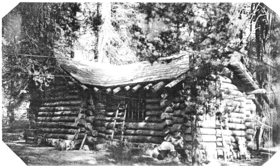
Historic Photo #2. West bedroom addition during construction. Photo is from final construction report, January 1935. Photographer unknown. Photo: Yosemite National Park, Division of Resources Management and Science, Branch of History, Architecture and Landscapes, El Portal, CA.
