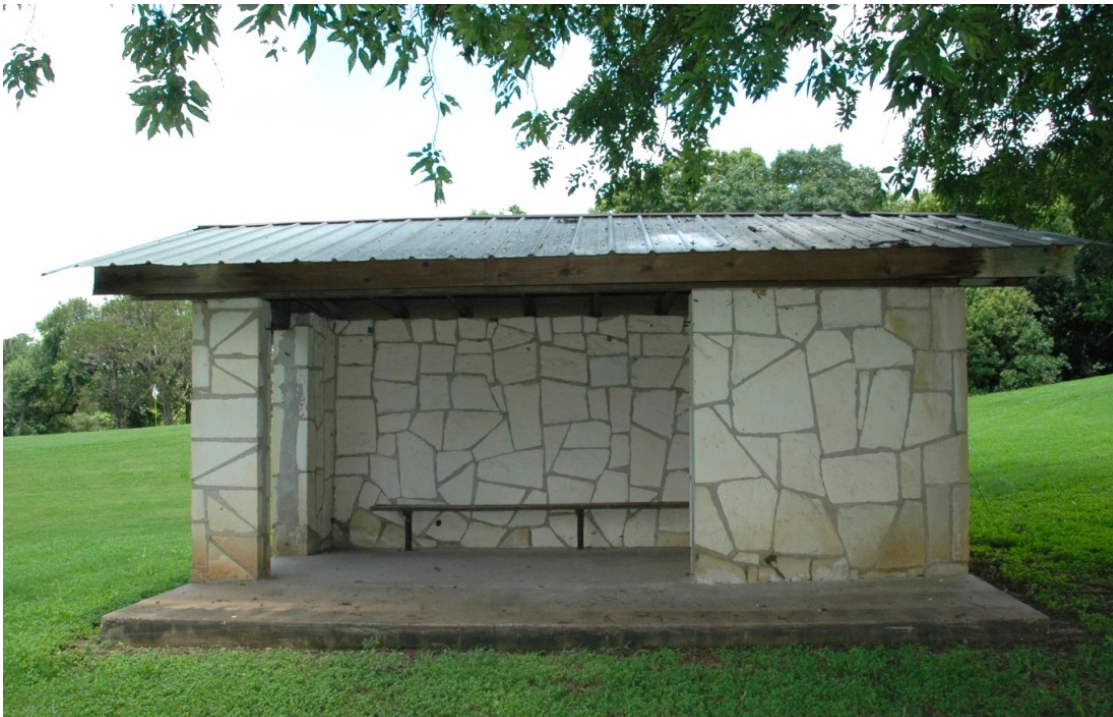
Photo 32: Camera Facing E. Limestone storm shelter (#24) between 12 th green and 13 th tees. West elevation.
