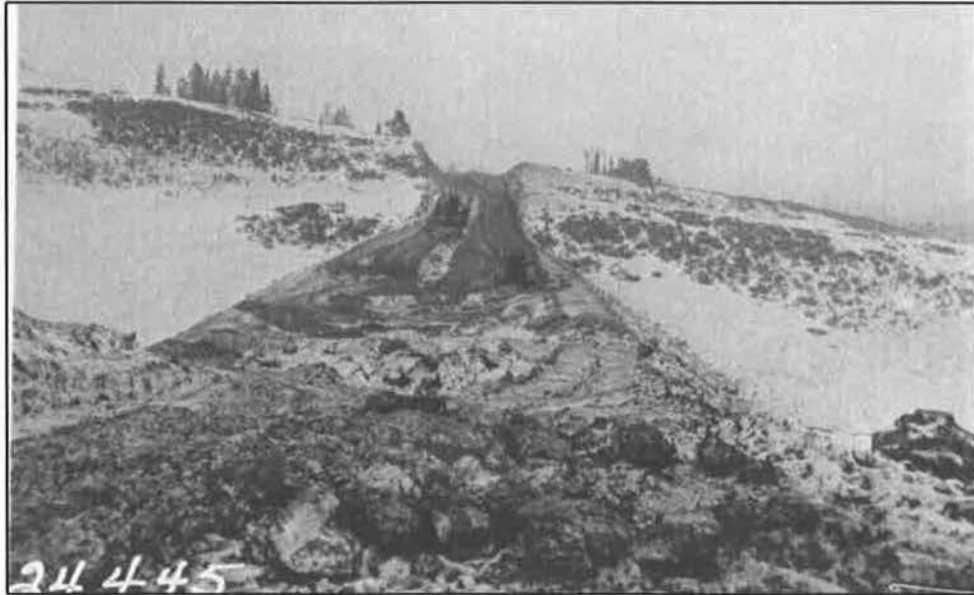
“Making the fill at Station 2266 with caterpillars and scrappers.” Final Construction Report (1931-1933) on Section B, Grading Red Lodge-Cooke City Approach Road to Yellowstone National Park, H. E. Mitchell, 1934. Photo No. 24445 from page 20A.
