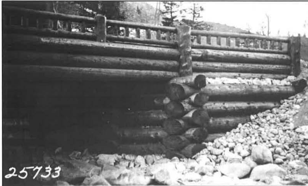
“Showing abutments, side logs and handrail on Rock Creek Bridge at Station 486.” Final Construction Report (1932-1933) on Red Lodge-Cooke City Approach Road to Yellowstone National Park, E-Section C, Grading E-Sections A and C, Surfacing. H. E. Mitchell, 1934. Photo No. 25733 from page 7.
