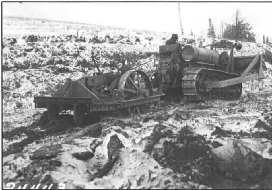
“Ripper and 60-caterpillar tearing up frozen common material. This 6-inch crust froze in the four hours intervening between the night and day shift.” Final Construction Report (1931-1933) on Section B, Grading Red Lodge-Cooke City Approach Road to Yellowstone National Park, H. E. Mitchell, 1934. Photo No. 24443 from page 20A.
