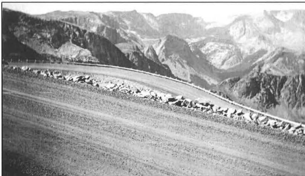
“Showing guardrail and bituminous mat during the curing process.” Final Construction Report (1933-1935) on Red Lodge-Cooke City Approach Road to Yellowstone National Park, on Section A, B, C, Portion D Bituminous Surface Treatment. H. E. Mitchell, 1935. Photo No. 29706 from page 9.
