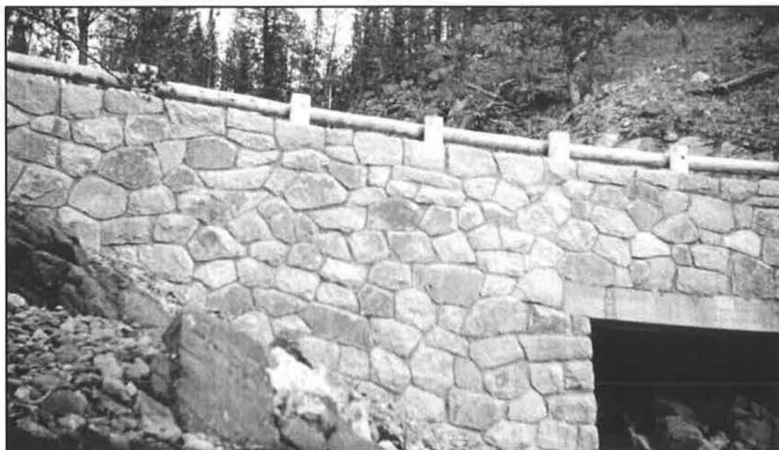
“End view of Rock Creek culvert.” Final Construction Report (1932-1934) on Section D, Grading Red Lodge-Cooke City Approach Road to Yellowstone National Park, H. E. Mitchell, 1934. Photo No. 26055 from page 8.
