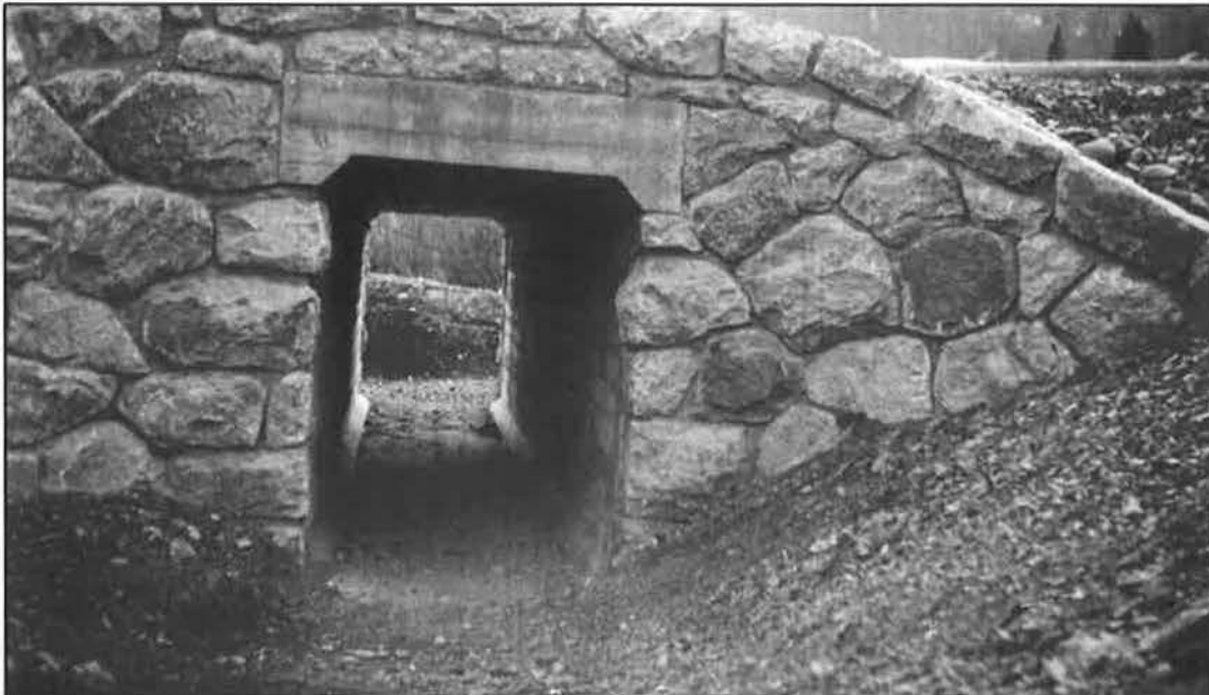
“Cattle pass at Sta. 2889+50.” This cattle pass was located adjacent to a private ranch. Final Construction Report (1932-1934) on Section D, Grading Red Lodge-Cooke City Approach Road to Yellowstone National Park, H. E. Mitchell, 1934. Photo No. 26056 from page 10.
