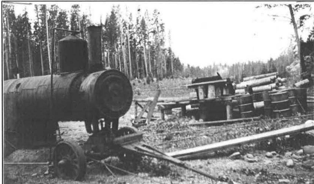
“Plant for treating guard rail posts. Steam from boiler on left was used to heat the creosote to the required temperature.” Final Construction Report (1935-1936) on Red Lodge-Cooke City Approach Road to Yellowstone National Park, on Section D (Portion), Surfacing, Bituminous Base Treatment and Bituminous Road Mix. L. A. Deklotz, 1936. Photo No. 29306 from page 7.
