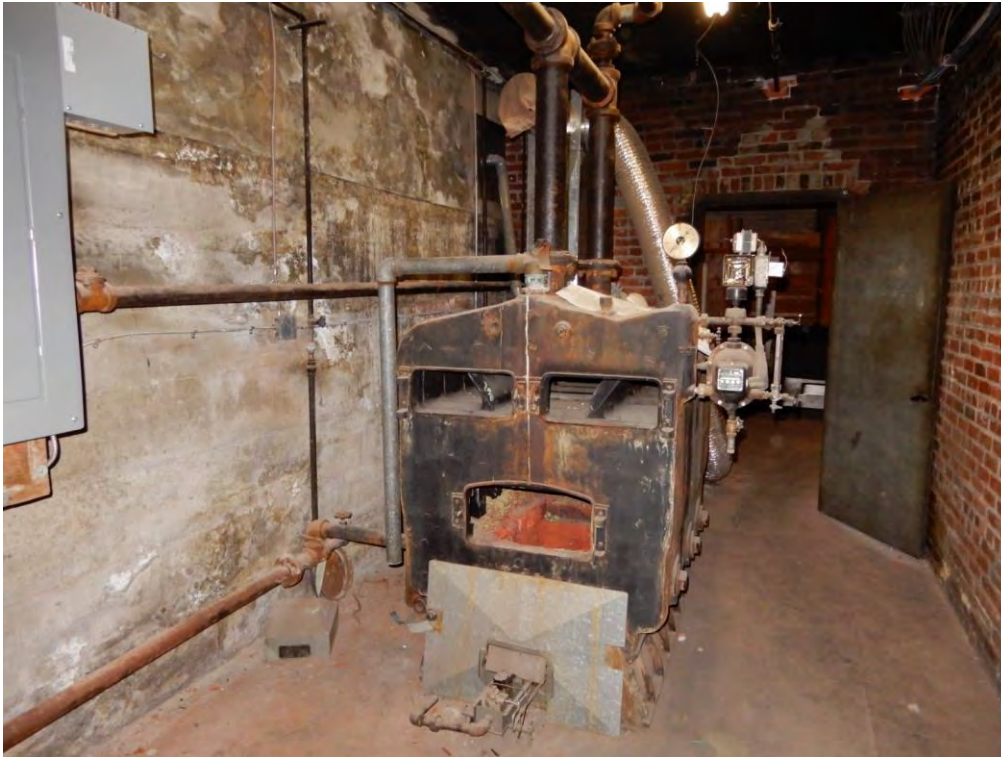
24 of 25 – Basement Boiler room.
