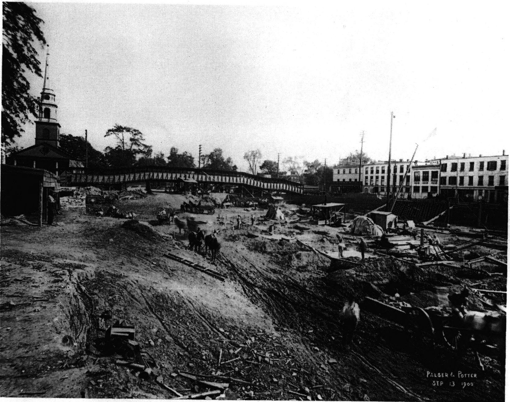
Plate 3 of 9: Hahne and Company department store construction site, northwest corner of Broad and New Streets. Original photograph by Palsler and Potter, September 13, 1900. View looking east.
