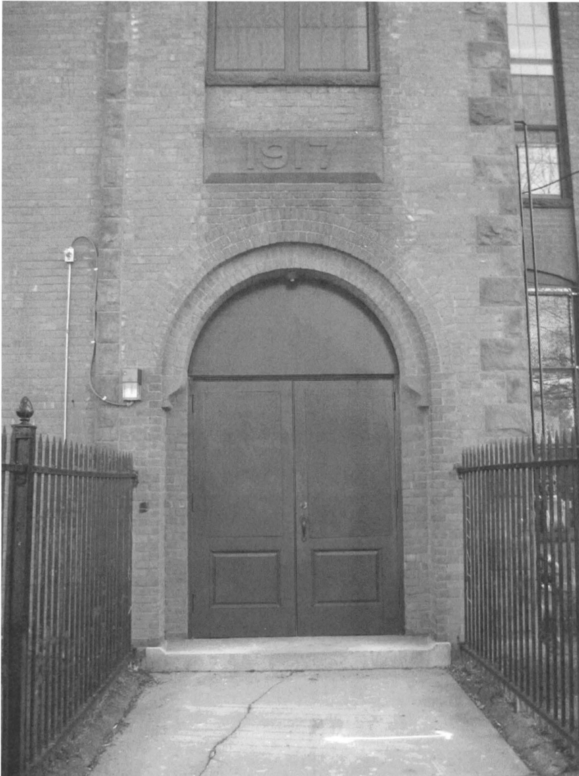
Detail of north stair tower; showing entryway, double fireproof doors, brick segmented relief arch, architrave, and brownstone quoins.
