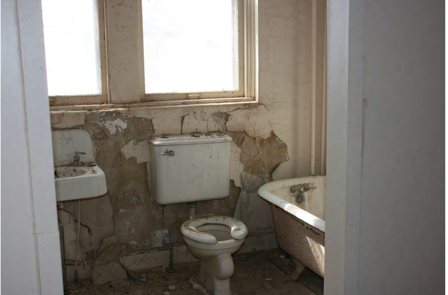
Photo 14: Second floor; private bathroom in the southwest corner room. Camera facing south.
