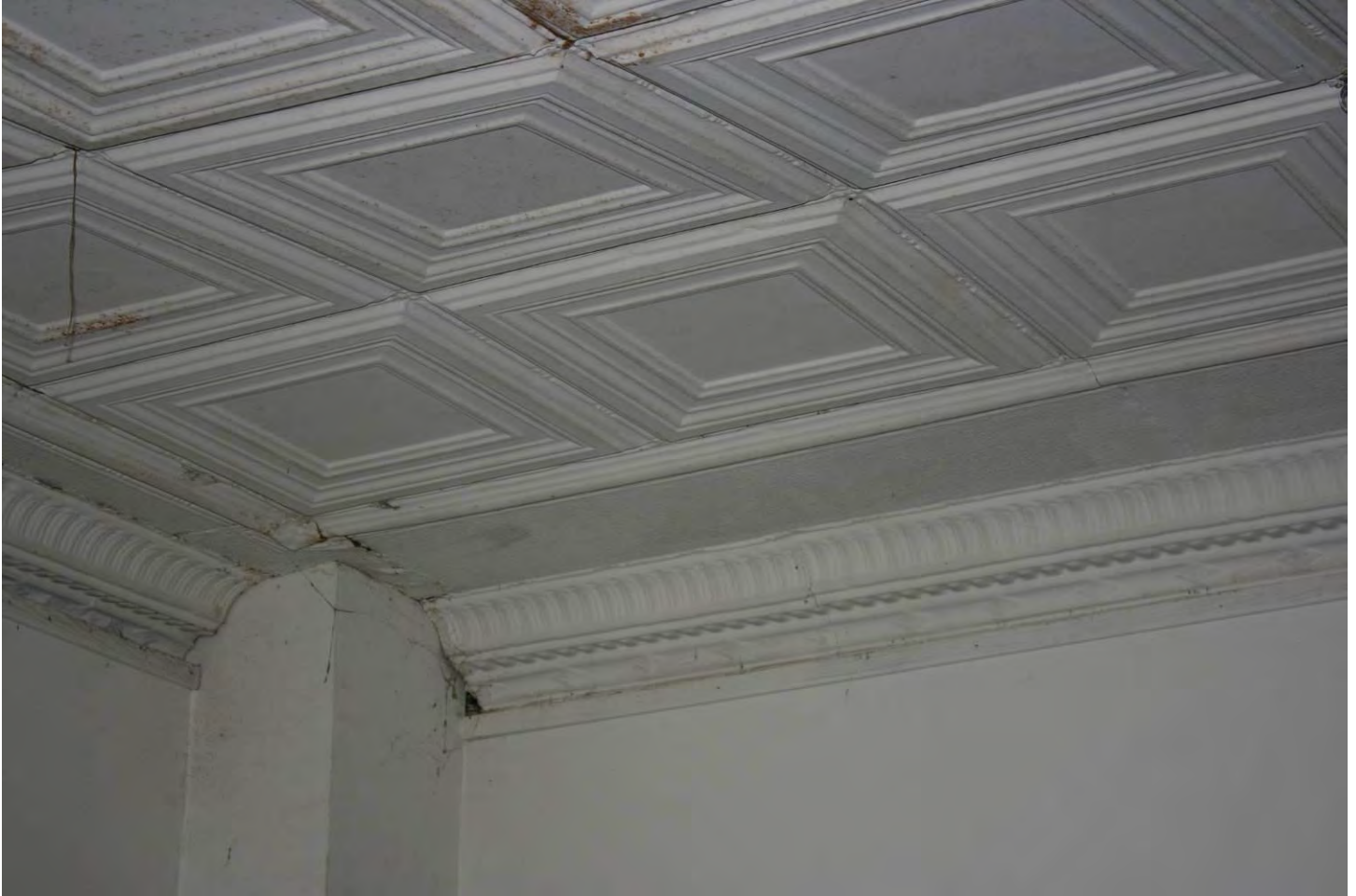
Photo 8: Pressed metal ceiling in a retail space.
