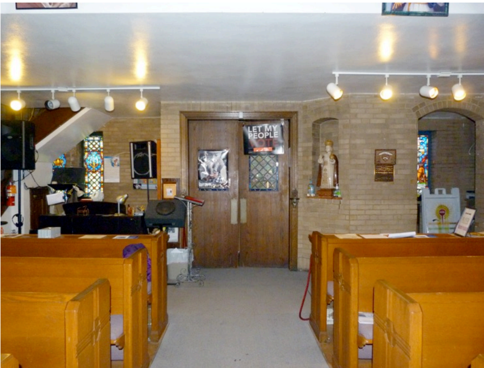
NJ_CAMDEN_ST. BARTHOLOMEW ROMAN CATHOLIC CHURCH_0017 Detail of central vestibule doors, looking south from nave.
