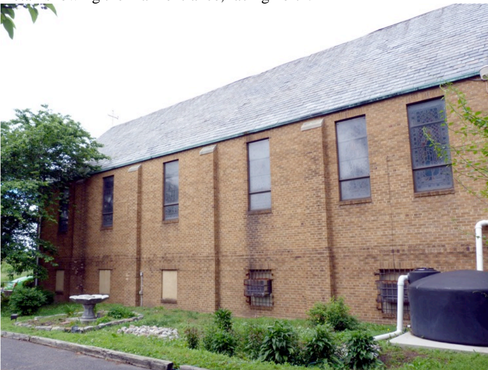
NJ_CAMDEN_ST. BARTHOLOMEW ROMAN CATHOLIC CHURCH_0011 View of the east elevation, facing southwest.
