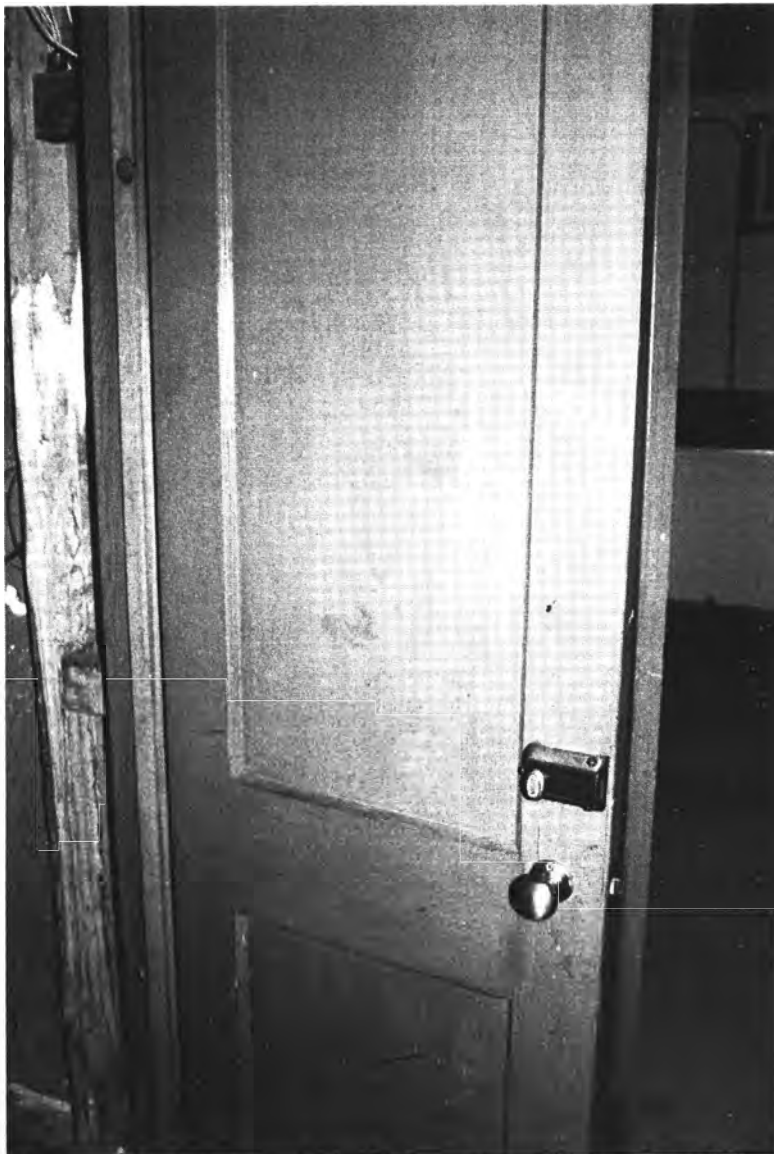
Name of Property: Target Range Elementary School City or Vicinity: Missoula County: Missoula State: Montana Photographer: Christine Brown Date Photographed: July 22, 2010 Location of Original Digital Files: Montana Preservation Alliance, 120 Reeder's Alley, Helena, MT.
