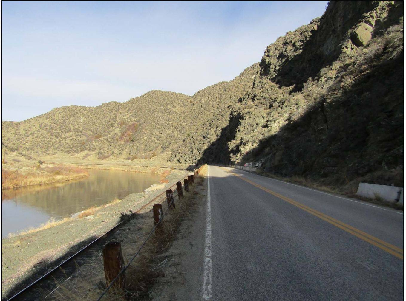
Photo # MT_JeffersonCounty_JeffersonCanyonHighwayHD_0012: The Jefferson Canyon Highway Historic District. Milepost 3.54. Rock Cut (Feature 8). View to the north. Photo date: November 30, 2017.
