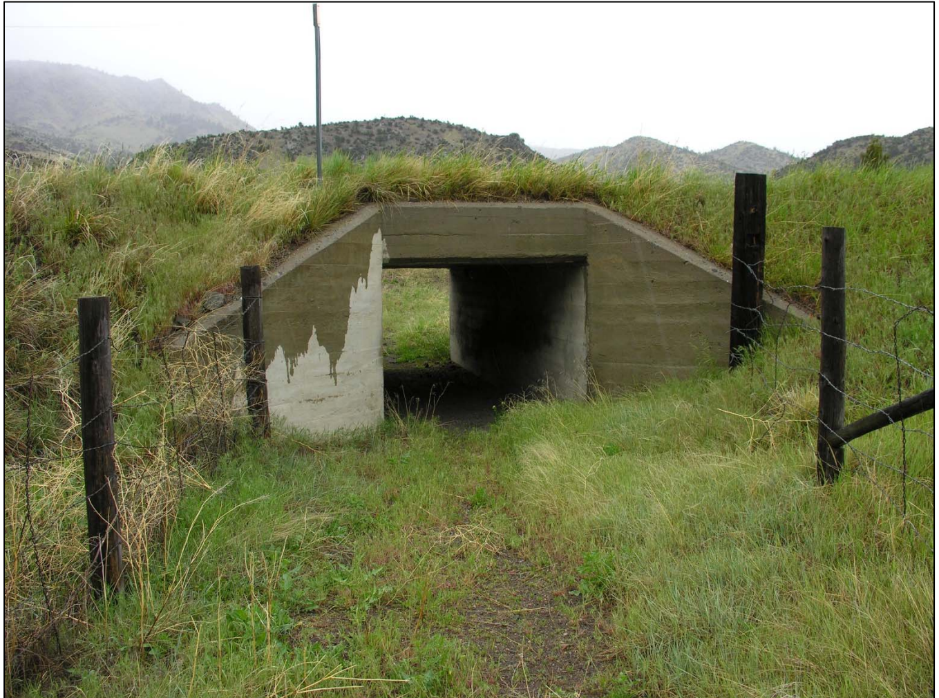
Photo # MT_JeffersonCounty_JeffersonCanyonHighwayHD_0028: The Jefferson Canyon Highway Historic District. Milepost 8.3. Culvert/Stockpass (Feature 14). View to the north. Photo date: June 2008.
