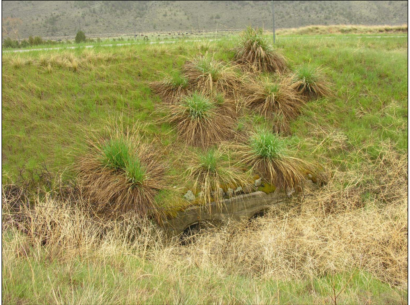
Photo # MT_JeffersonCounty_JeffersonCanyonHighwayHD_0025: The Jefferson Canyon Highway Historic District. Milepost 7.6. Culvert (Feature 12). View to the north. Photo date: June 2008.
