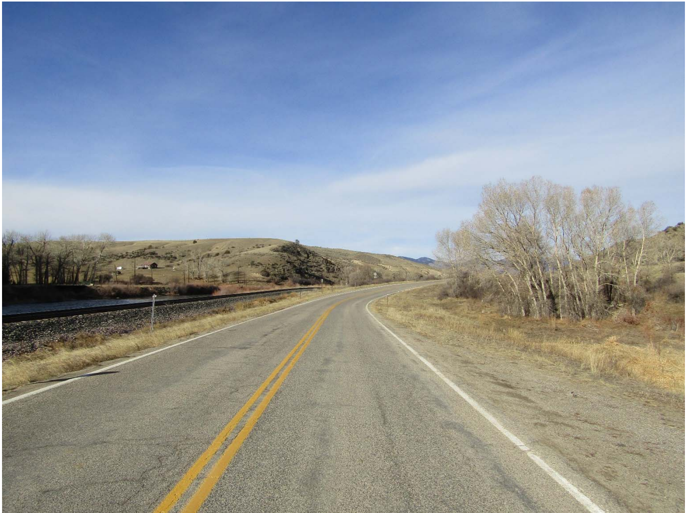
Photo # MT_JeffersonCounty_JeffersonCanyonHighwayHD_0002: The Jefferson Canyon Highway Historic District. Milepost 3.04. View to the northwest. Photo date: November 30, 2017.
