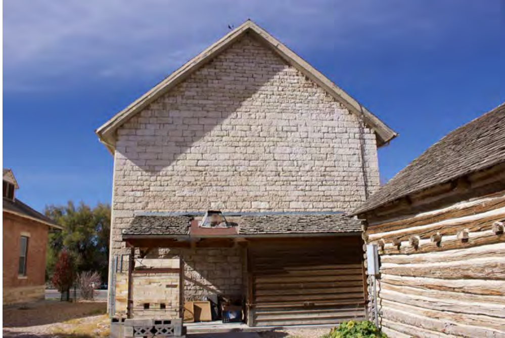
5 of 21: East elevation of granary. Camera facing west. (Photo by Jamyn Maddox, 10/31/18)
