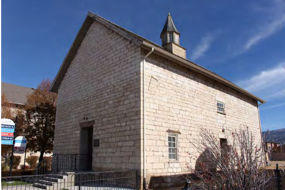
3 of 21: South-west corner of granary. Camera facing north-east. (Photo by Jamyn Maddox, 10/31/18)
