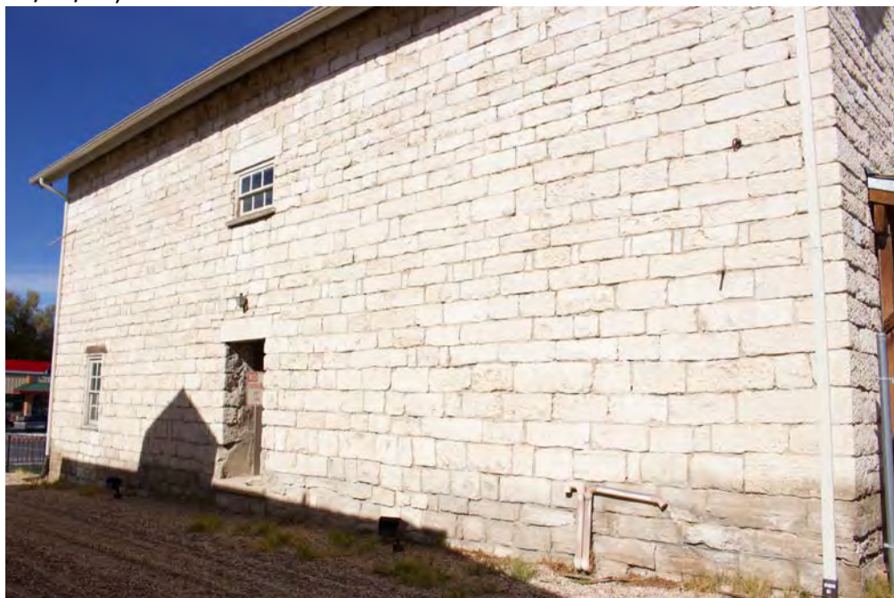
2 of 21: South elevation of granary. Camera facing north-west. (Photo by Jamyn Maddox, 10/31/18)
